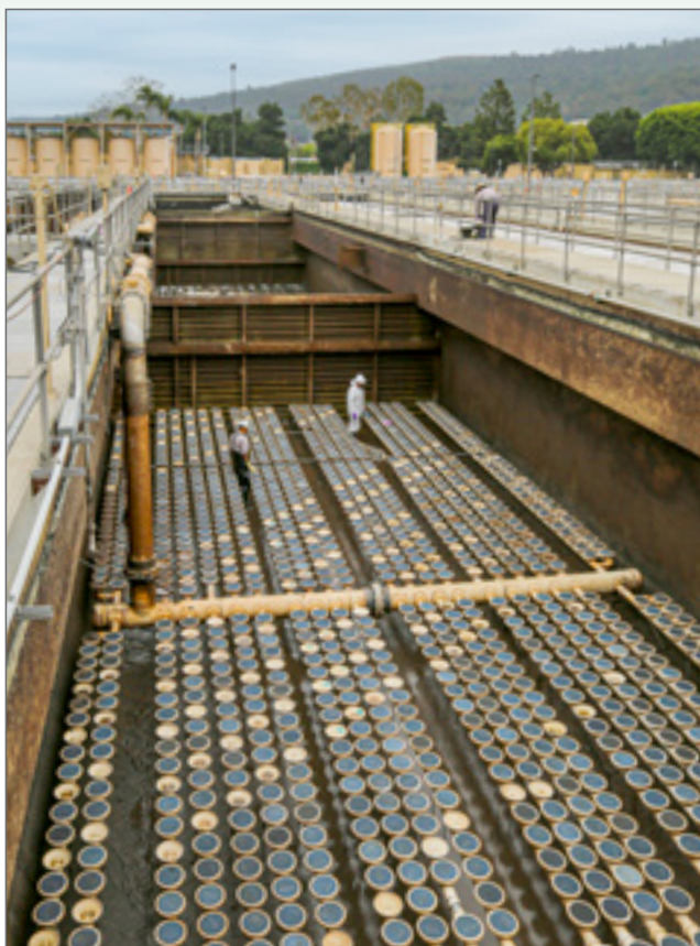
Three of our 1,700 employees performing maintenance work at San Jose Creek WRP
