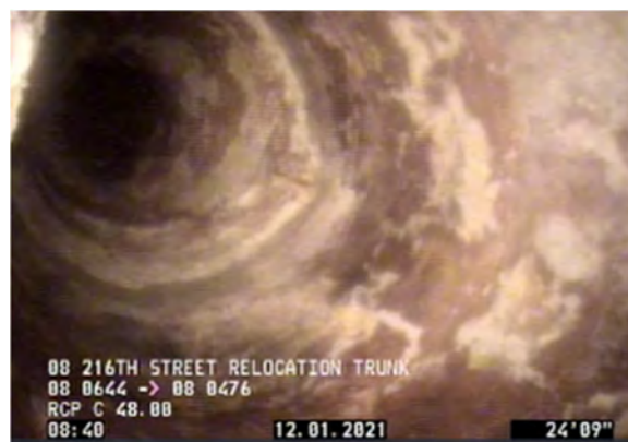
Photo 3-3 CCTV Inspection Photograph 3
