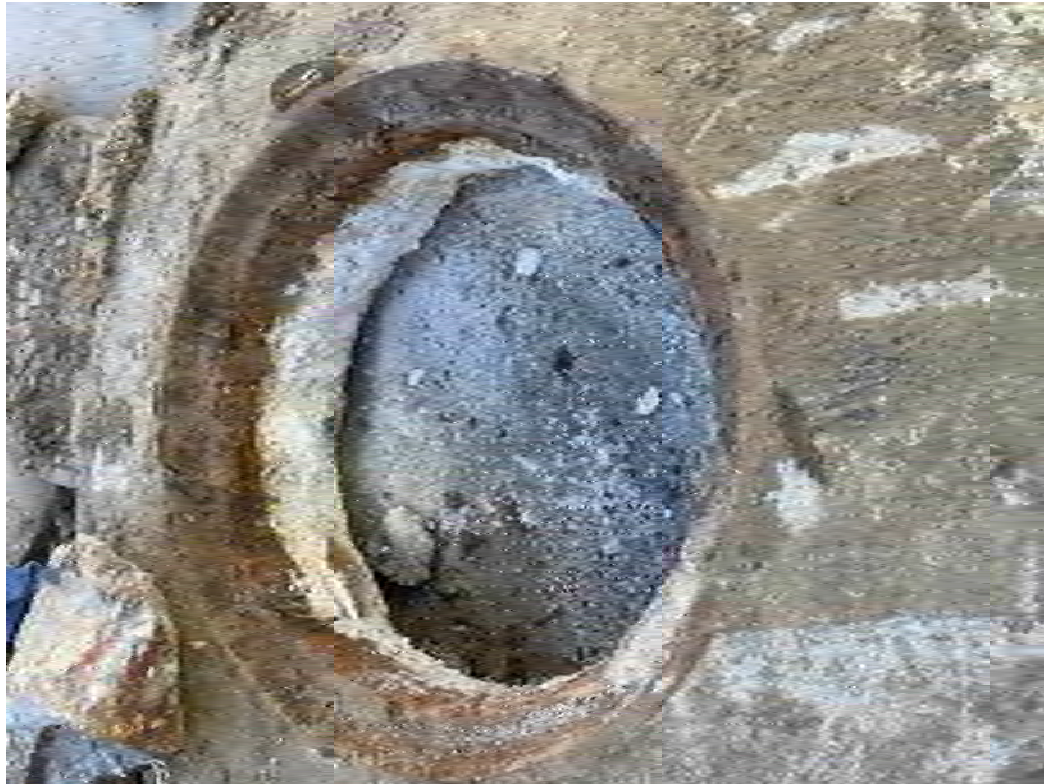
Photo 3-12 Manhole Ring and Cover Debris
