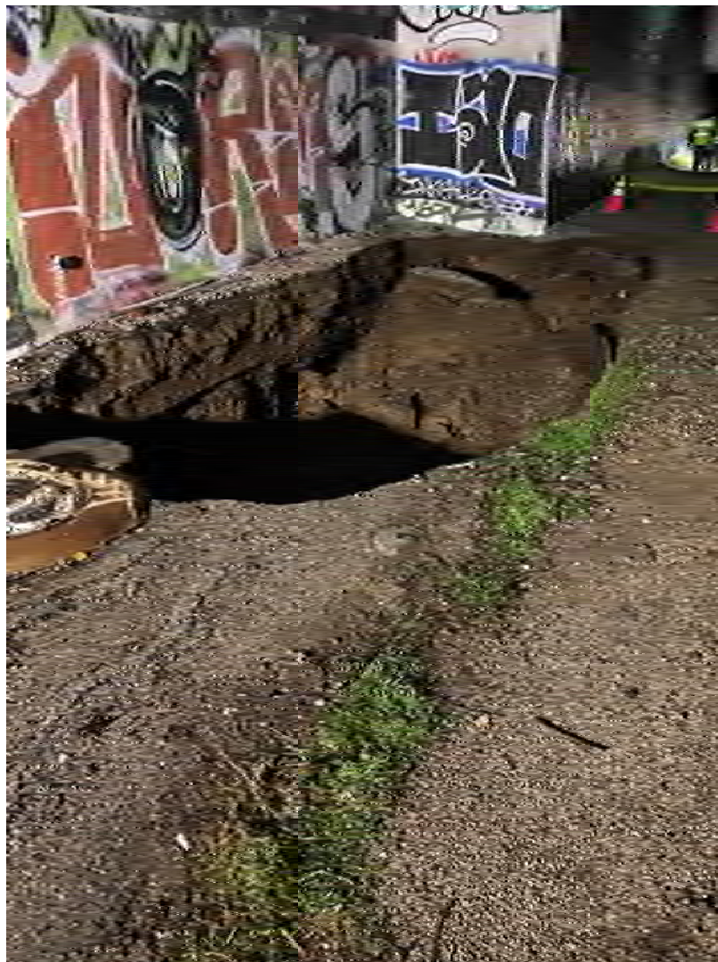
Photo 3-5 Location of the Pipe and Manhole After the Failure
