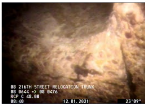
Photo 3-2 CCTV Inspection Photograph 2
