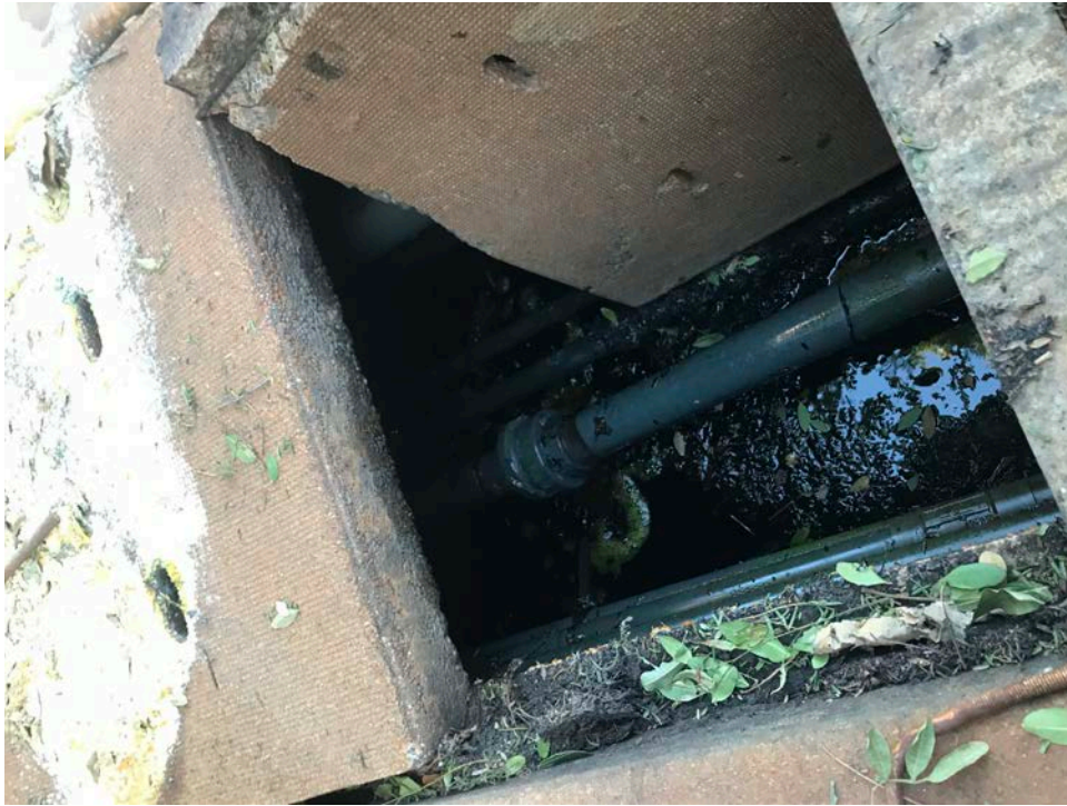
Figure 9: 10-13-2021 picture of the separated connection on the ferrous chloride line that was causing the chemical to leak into the influent sewer line at the Long Beach WRP, causing the orange and green colors noted at the WRP.
