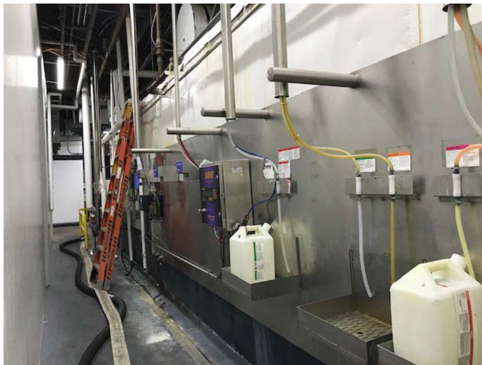
Figure 6: 5-21-2021 photo of the chiller water tank that contained the released ammonia at Safeway, Inc. in Commerce.
