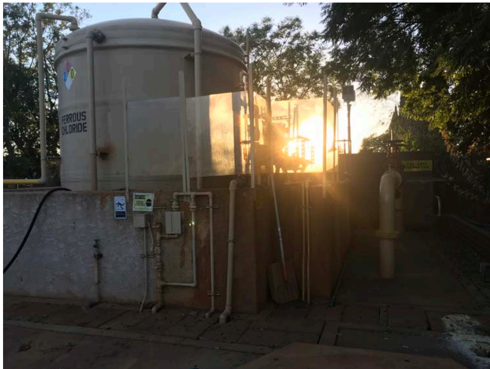
Figure 8: 10-13-2021 photo of the ferrous chloride addition system at the Long Beach WRP odor control station.
