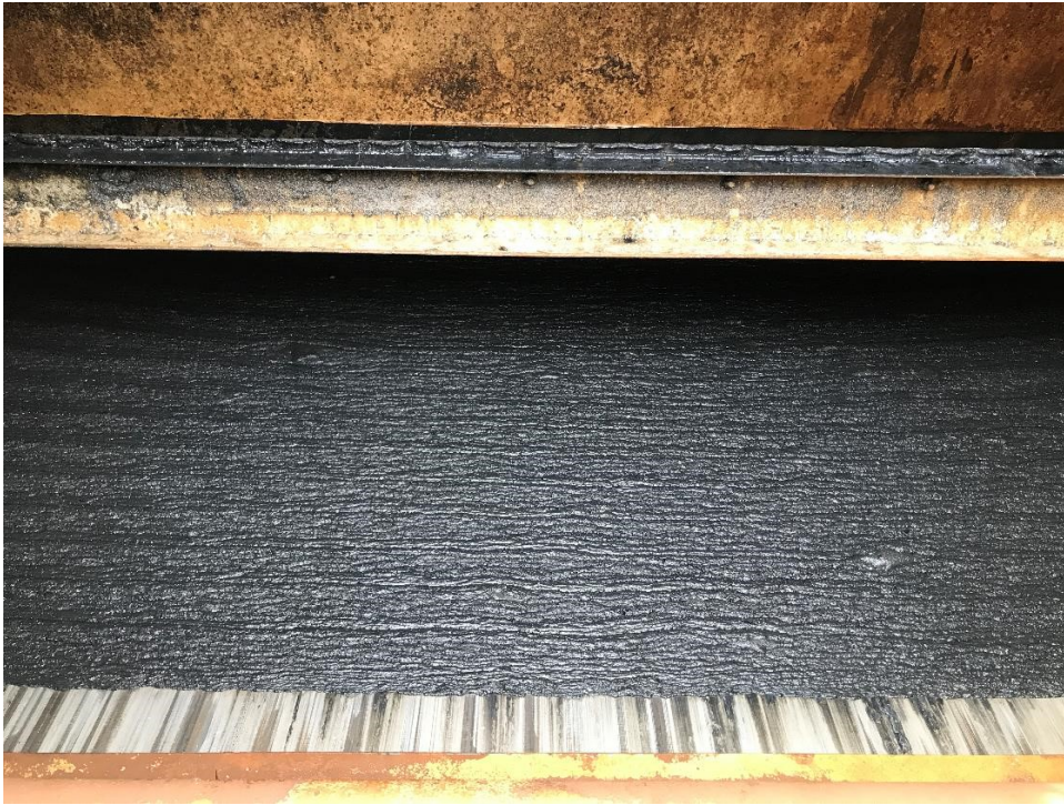
Figure 4: 4-25-2021 floating black oily solids in the skimming trough of the E-1 battery of sedimentation tanks at JWPCP.
