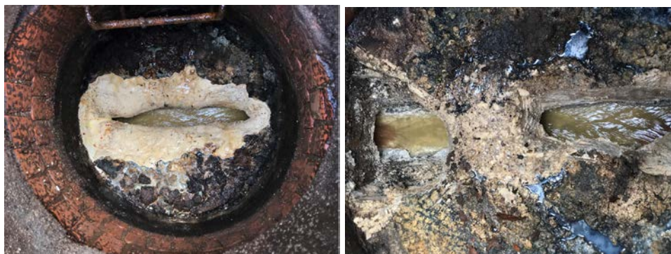
Figures 7 and 8: 3-23-2021 local sewer line manhole grease in Azusa.
