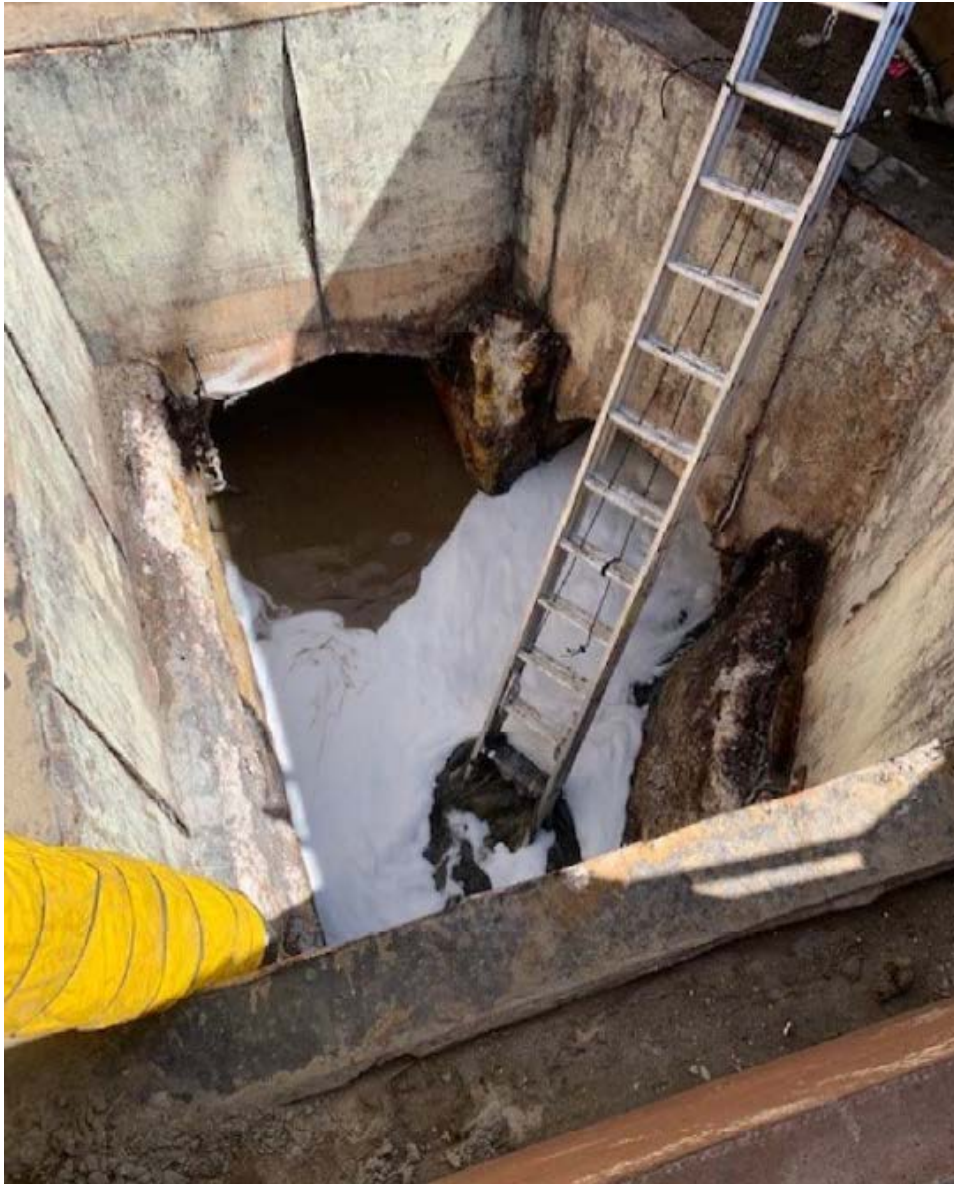
Figure 3: Looking into the vault that is MH 18 A575 on 3-17-2021. Note the white foam and the yellow air blower hose used to control the presence of sulfide gas.
