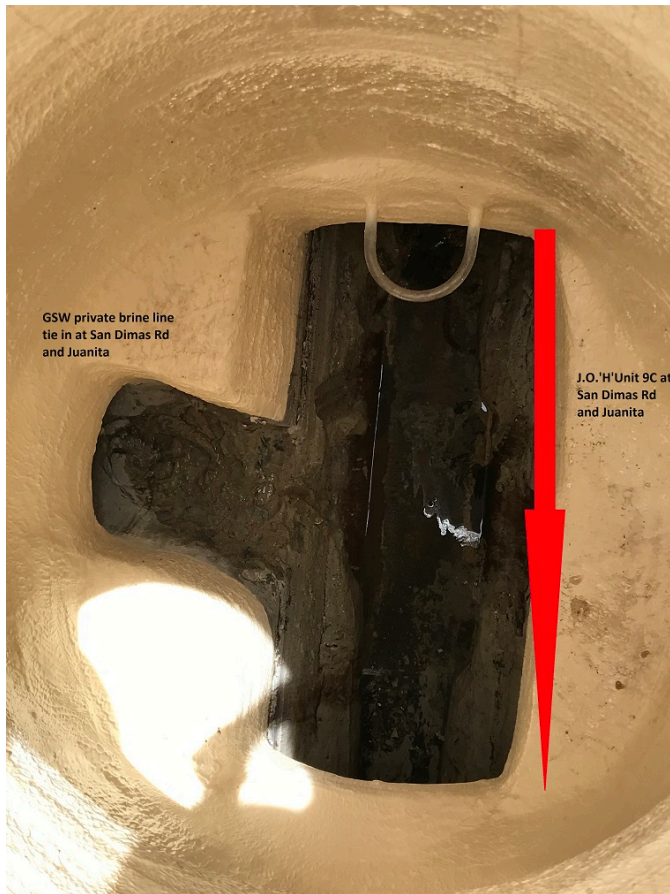
Figure 2: 7-26-2021 new manhole and connection to the J.O. 'H' Unit 9C trunk sewer, located at San Dimas Canyon Road and Juanita Avenue. Note the lack of solids in the line.
