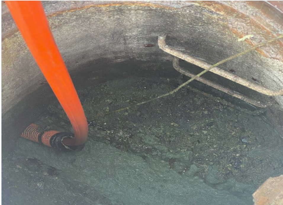
Figure 6: City of Pomona sewer maintenance staff photo showing excessive grease in a city sewer line at approximately 1047 E. 3rd Street. Note that the line channel is completely full of grease.
