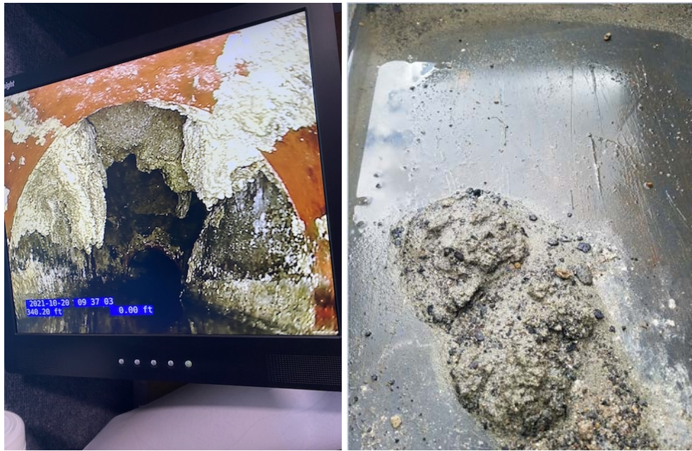
Figures 10 and 11: 10-20-2021 Pomona city sewer maintenance CCTV and photo of the FOG and debris removed from the local line at approximately 4200 Valley Boulevard.
