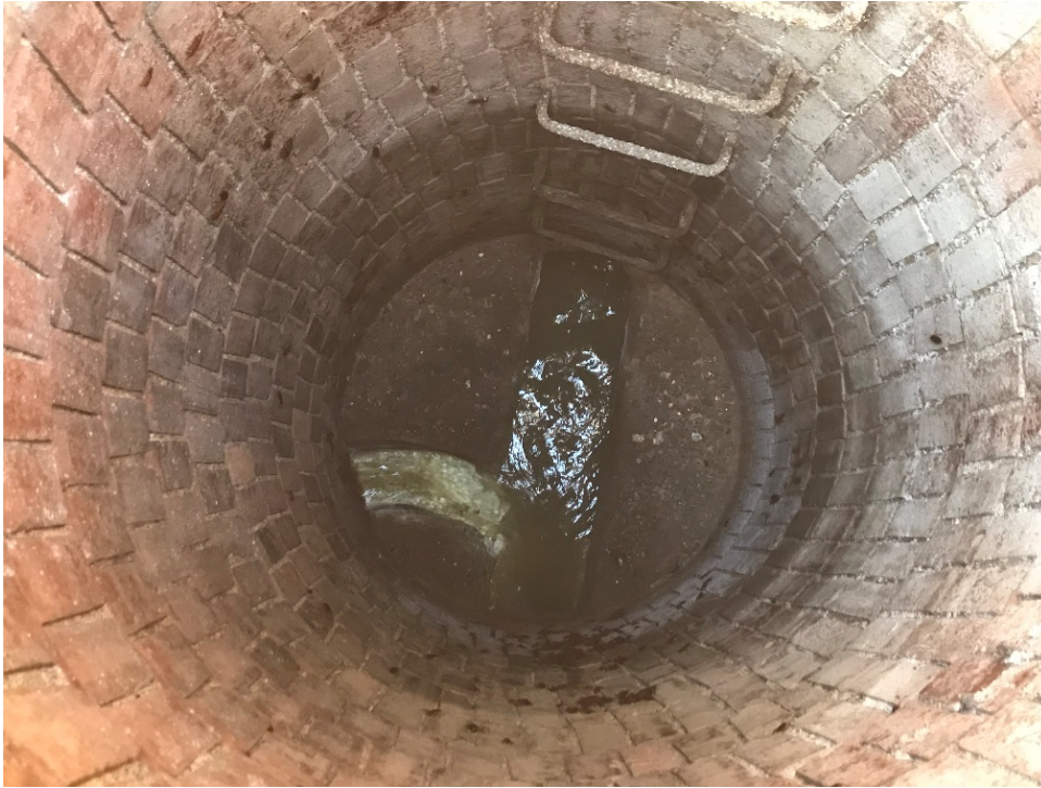
Figure 9: 3-23-2021 MH 22 0914A; where the local line shown above joins the Districts' 15" diameter Coney trunk sewer. Note the grease in the local sewer line and lack of such in the Districts' line. The Coney trunk was cleaned at this location on 2-24-2021.
