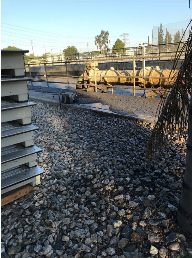
Figure 8: 2-18-2021 excessive foam in aeration tank at LCWRP at 0730 hours. Note that the foam got deep enough to overflow onto the walkway above the tank.
