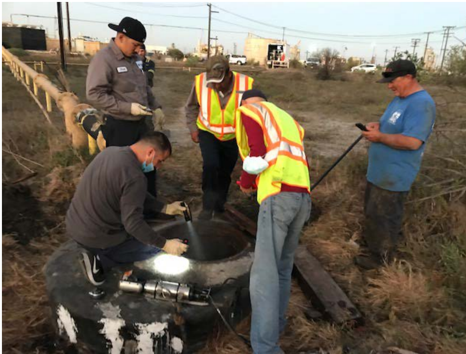
Figure 13: WCS personnel examining MH 03 0556 on 8-13-2021. Note the above ground 8" diameter Synergy IW discharge line in the background.
