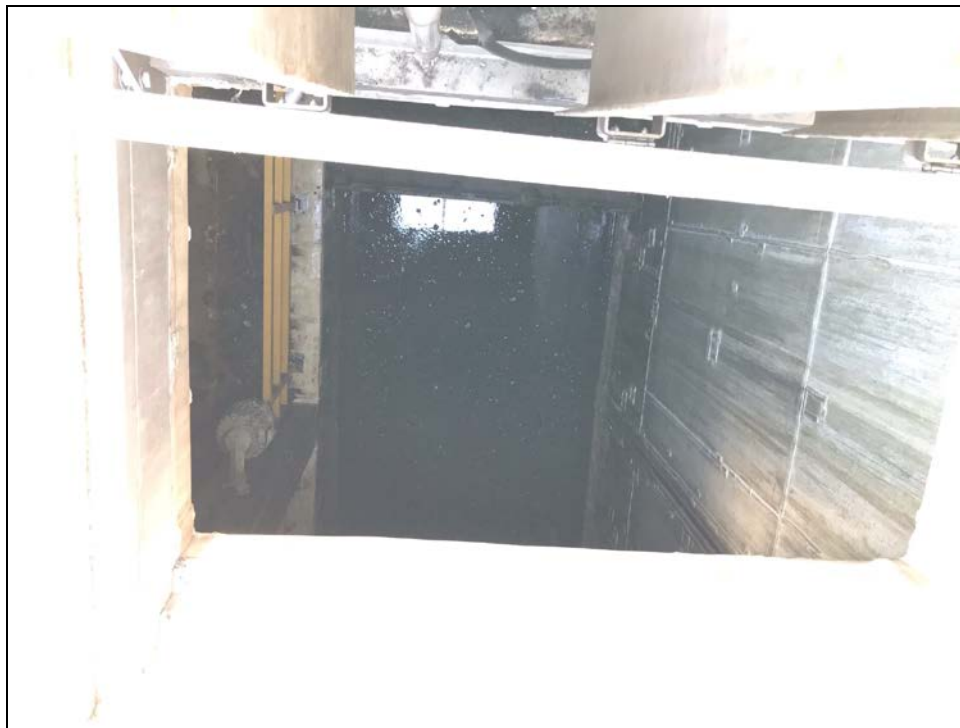
Figure 1: Floating oil in the wet well at the Long Beach Main Pumping Plant on 3-9-2021.
