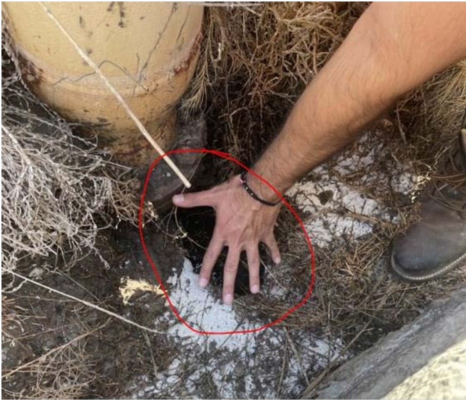
Figure 11: 6" wide hole in the ground next to Synergy's discharge line and MH 03 0556 on 8-13-2021. MH 0556 cover structure at lower right.
