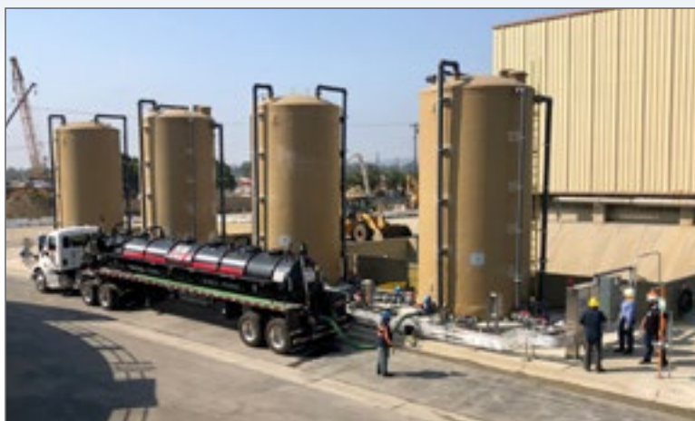
A tanker truck unloads food waste slurry at the JWPCP receiving station
