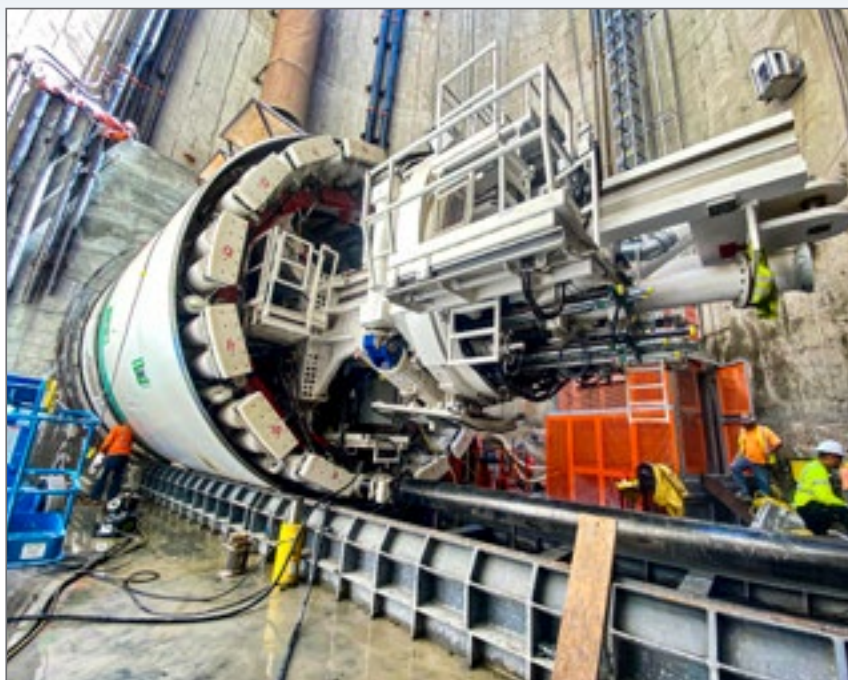
In 2021, the Clearwater Project's tunnel boring machine, Rachel , began her four-year, seven-mile journey from Carson to Royal Palms Beach
