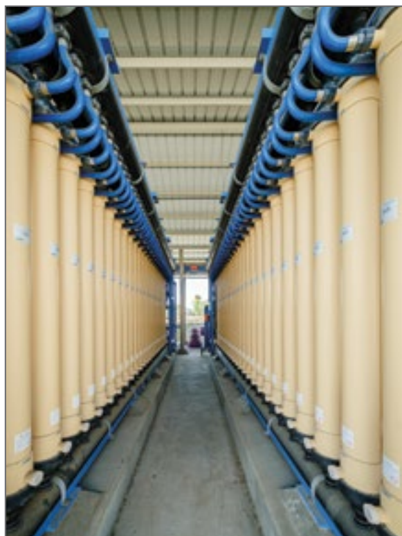
The Leo J. Vander Lans Advanced Water Treatment Facility purifies effluent from the Long Beach WRP
