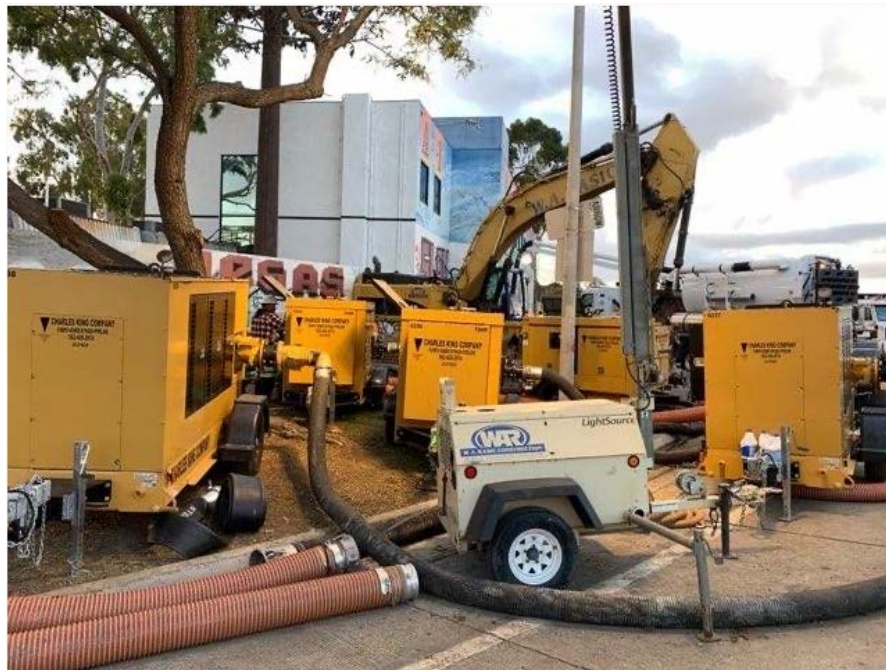
Photo 12: Emergency repair site on January 1, 2022 showing five of the eight bypass pumps installed to bypass flow around the collapsed sewer to MH 08 0475. Tight site conditions presented challenges for installing the bypass pumping equipment. View facing southeast from the I-110 Freeway off-ramp to 220 th Street.
