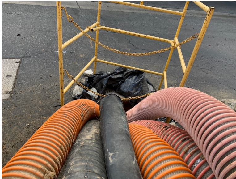
Photo 14: Pump discharge piping into MH 08 0475 on the morning of January 1, 2022 after all eight bypass pumps were in operation. Installation of the final four pumps required modifications to the discharge piping of the first four pumps to fit the additional discharge pipes into the manhole.
