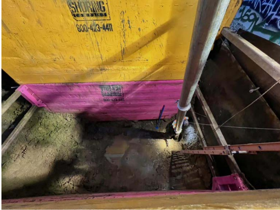
Photo 9: Removal of collapsed soil and debris in the excavation pit using a combination jetter-vacuum truck on December 31, 2021 at 6:44 a.m.
