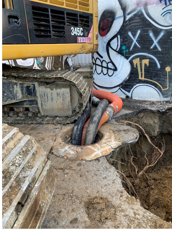
Photo 13: Pump suction piping in one of two suction manholes on the morning of January 1, 2022 after all eight bypass pumps were in operation. Installation of the final four pumps required modifications to the suction piping of the first four pumps to fit the additional suction pipes into the manhole.
