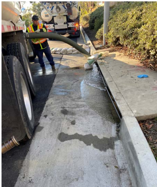
Photo 16: LACSD staff using a water truck to flush storm drain with potable water on January 1, 2022. View facing west on West 212 th Street.
