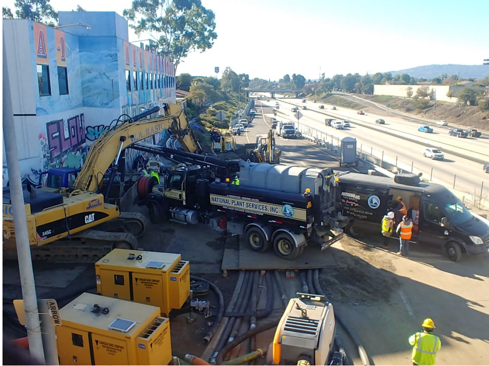
Photo 21: Combination jetter-vacuum truck working to remove soil and debris from the downstream sewer pipe while CCTV inspection is intermittently used to check the condition of the pipe (black CCTV van at right). View facing south on January 2, 2022 at 9:51 a.m.
