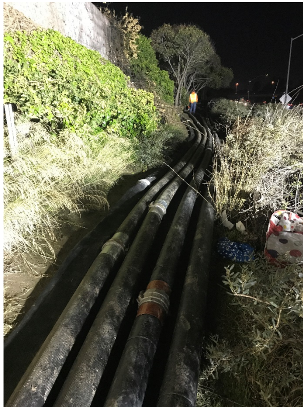
Photo 6: Discharge piping for bypass pumps along I-110 Freeway soundwall while piping was being installed for fifth bypass pump on December 31, 2021 at 7:21 p.m. Difficult terrain and thick vegetation presented challenges for installing the bypass piping. View facing south.
