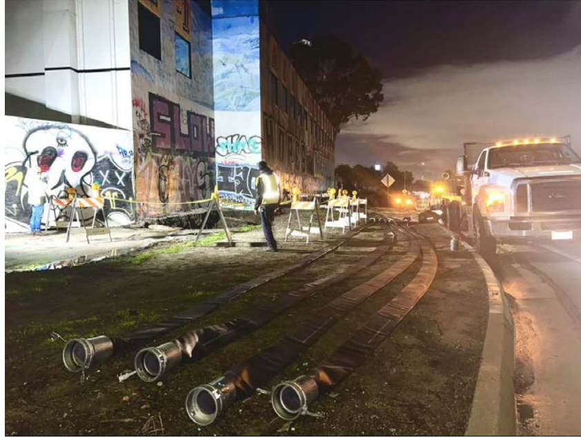
Photo 5: Preparation of discharge hoses for the emergency bypass between MHs 08 0644 and 08 0475 on the 216 th Street Relocation Trunk Sewer. Photo taken on December 30, 2021 at 8:47 p.m. View facing south from the I-110 Freeway northbound off-ramp to 220 th Street.
