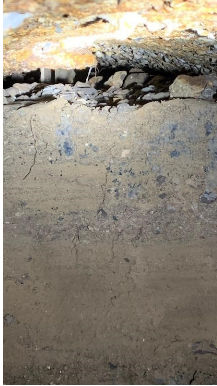
Photo 19: Closeup of the soil and debris found in the sewer just downstream of the sinkhole on December 31, 2021 at approximately 1:30 p.m. The soil and debris filled the pipe up to a couple inches from the top of pipe for about 20 feet downstream of the sinkhole.
