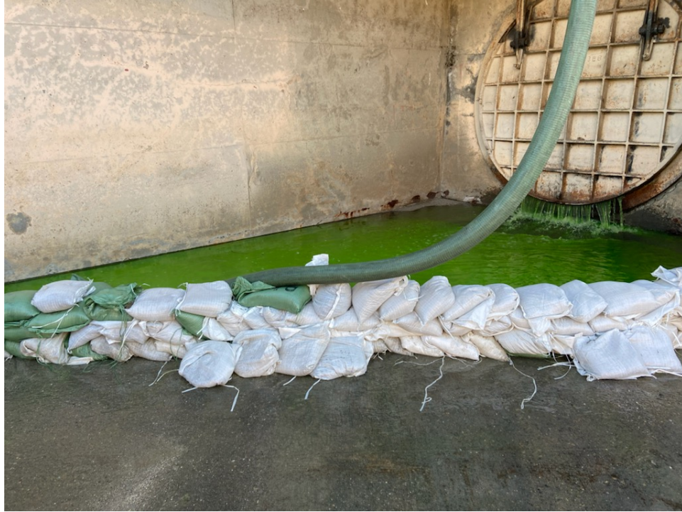
Photo 17: Storm drain flush water containment setup at the storm drain outlet to the Torrance Lateral on January 1, 2022. Green dye was used as an indicator to ensure that all flush water was captured. All flush water was returned to the sewer system.
