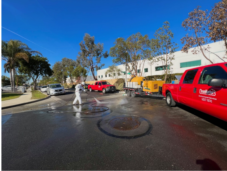
Photo 27: Clean Harbors, Inc. washing and sanitizing the impacted street area on the morning of January 5, 2022. View facing northwest at the intersection of West 212 th Street and South Moneta Avenue.
