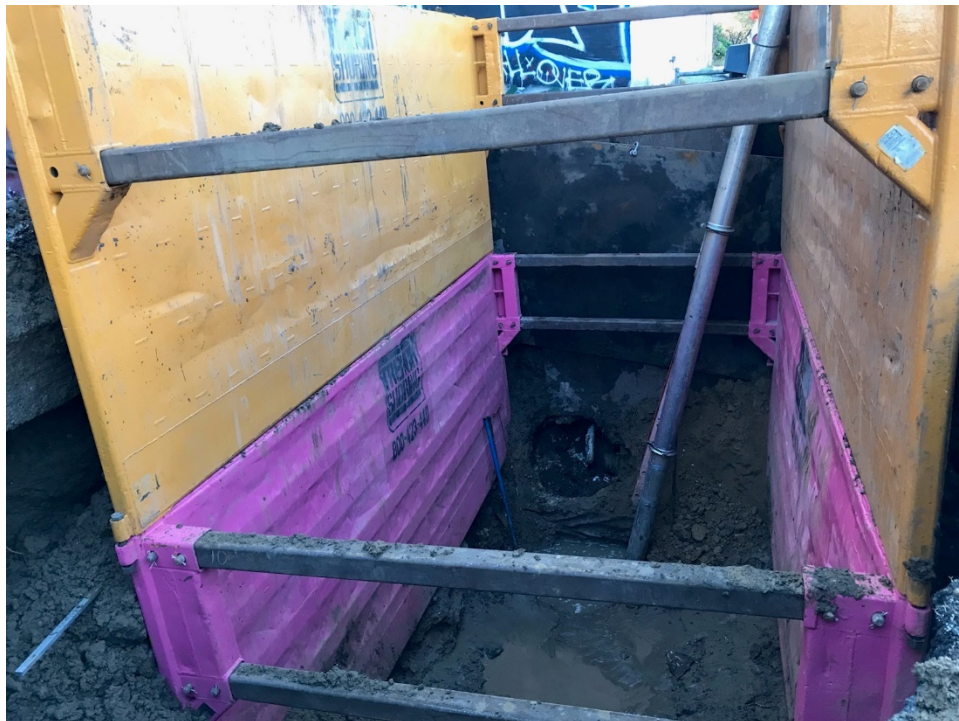
Photo 18: Sinkhole excavation pit on December 31, 2021 at 8:03 a.m. A large amount of soil and debris was encountered in the downstream sewer pipe that slowed progress with restoring flow in the sewer.
