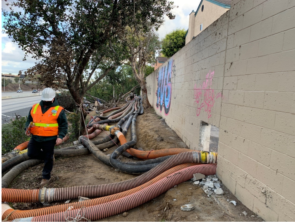
Photo 7: A hole was cut in the I-110 Freeway soundwall to gain access to the downstream discharge manhole for the bypass system. The hole was later repaired after the bypass system was removed. View facing north on the morning of January 1, 2022 with piping for all eight bypass pumps installed.
