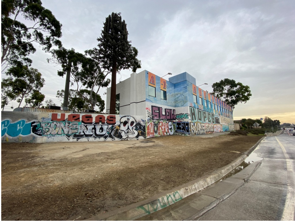
Photo 25: Restoration of the sinkhole site was completed on January 13, 2022 and the I-110 Freeway off-ramp was reopened that night at approximately 8:00 p.m. View facing southeast from the I-110 Freeway off-ramp.
