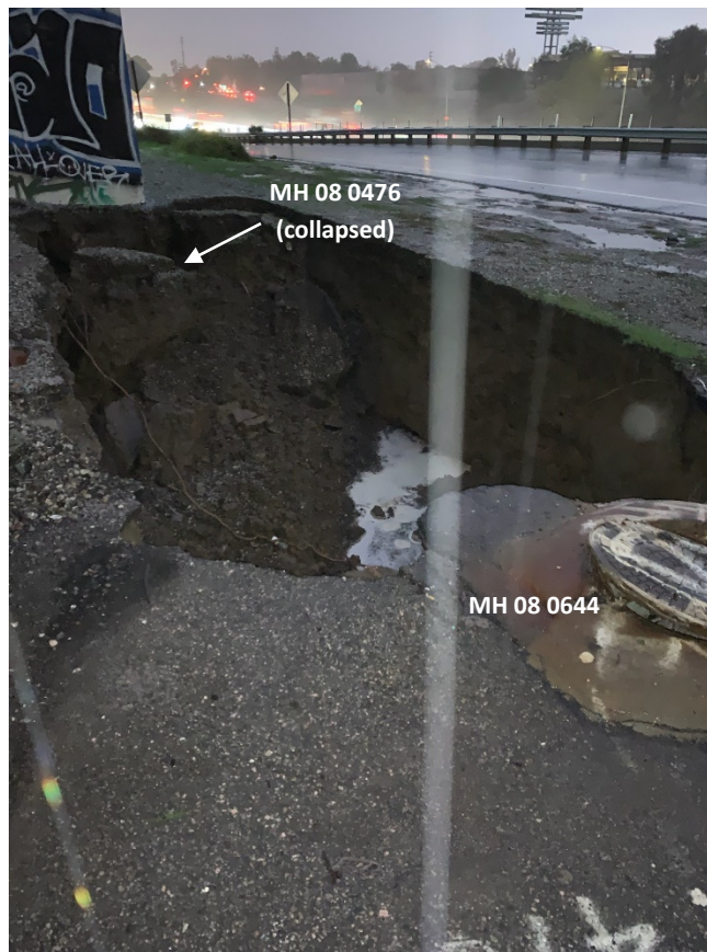
Photo 4: Sinkhole between MHs 08 0644 and 08 0476 on the 216 th Street Relocation Trunk Sewer immediately after it was found at approximately 5:03 p.m. on December 30, 2021. View facing southwest, approximately 30 feet east of the I-110 Freeway northbound off-ramp to 220 th Street.
