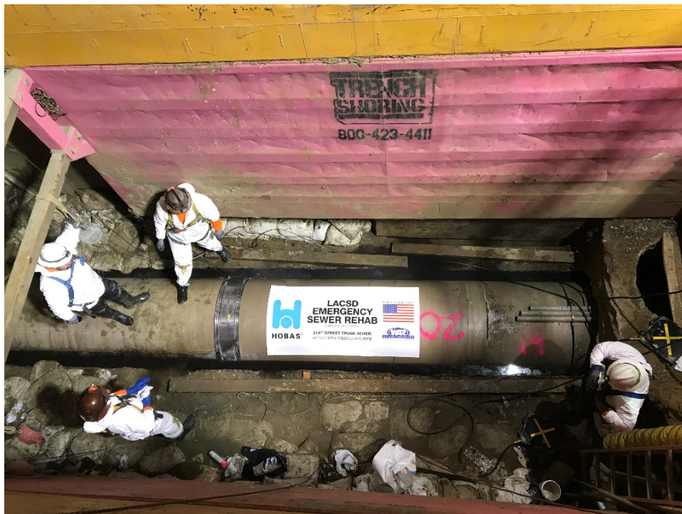
Photo 24: Final segment of 42-inch CCFRPM pipe installed on January 8, 2022 at approximately 6:00 p.m. to repair the damaged sewer.
