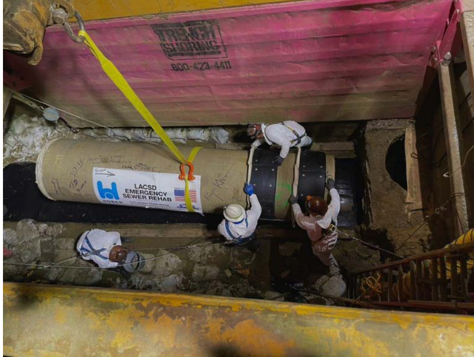
Photo 23: Emergency construction contractor installing the first segment of 42-inch CCFRPM pipe on January 7, 2022 to repair the 216 th Street Relocation Trunk Sewer by slip-lining the existing 48-inch pipe.
