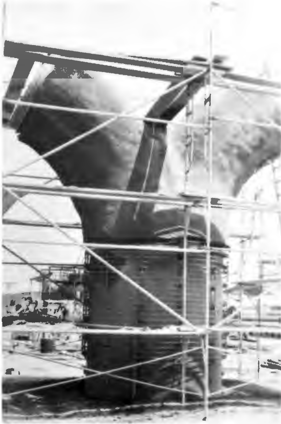
PRECAST WYE 90-INCH OCEAN OUTFALL — The 90 by 60 by 60 inch wye placed in ocean outfall at connection to wye diffusion structure. White's Point.
