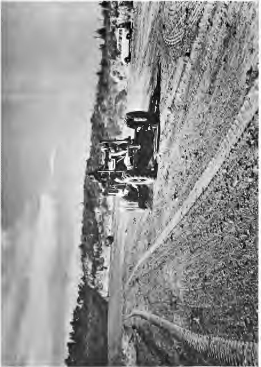
FINISHING OFF LANDFILL — Covering and grading top of landfill. Top cover not less than two feet of native material.
