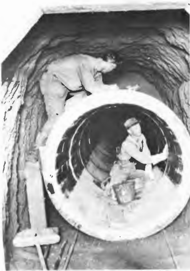
TILE-LINED PIPE IN TUNNEL, DISTRICT 5 —Tunnel construction in the District 5 main trunk, January, 1928. Note tile lining in pipe, placed to protect against deterioration of concrete from oxidized hydrogen sulfide.
