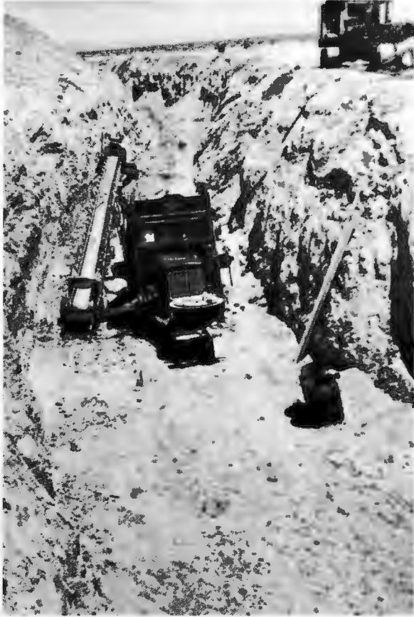
DEEP TRENCHING; DISTRICT 14—Rosamond Outfall Sewer, District 14. Deep trench partially excavated with dragline; later with trencher to grade.
