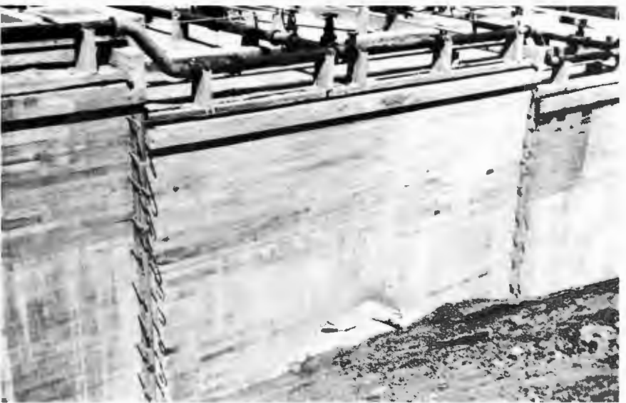
MULTISTAGE DIGESTION TANKS—View of the east wall of Battery B of the sludge digestion tanks completed at Joint Disposal Plant in 1930. Protruding reinforcing rods are for connecting Battery C later.
