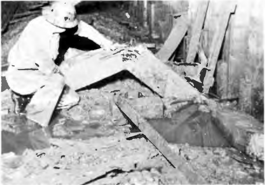
HEAVING GROUND IN TUNNEL CONSTRUCTION —In particularly heavy and squeezing ground in the White's Point tunnel construction, heavy bracing was required. Steel ribs were difficult to obtain at all times; hence, some tunnel support with timber.
