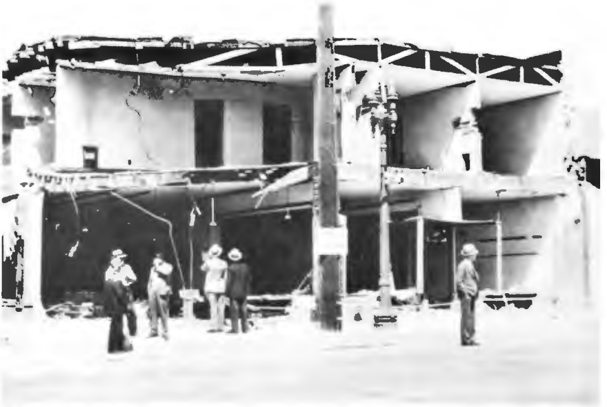
EARTHQUAKE (MARCH 10, 1933) DAMAGE. COMPTON—Most of the Districts' structures, being underground, suffered little damage in a quake that was intense enough to severely damage many surface structures.
