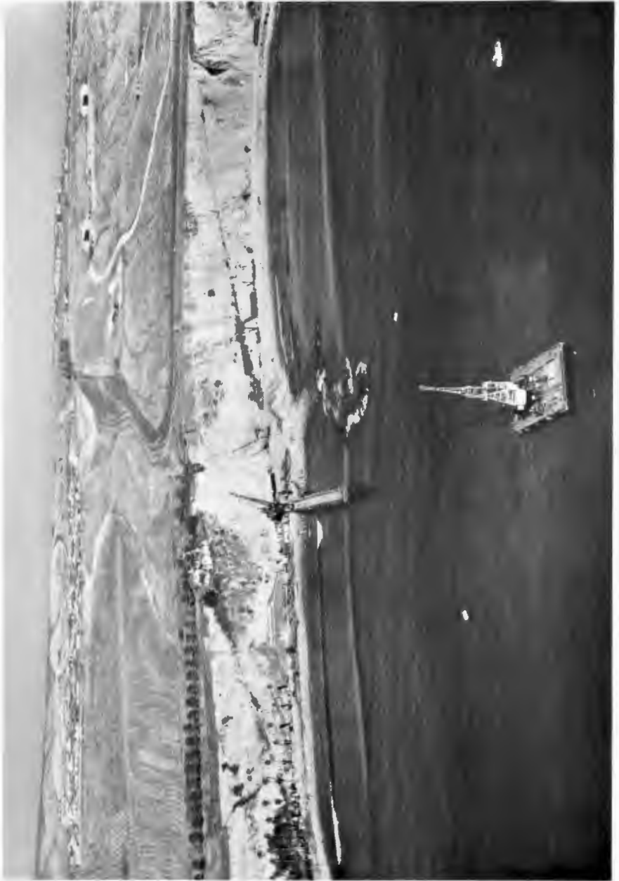
CONSTRUCTION OF NINETY INCH DIAMETER OUTFALL — District construction barge in foreground; construction trestle through surf, White's Point, 1955. The outfall tunnels terminate at cliff. Palos Verdes hills in background.
