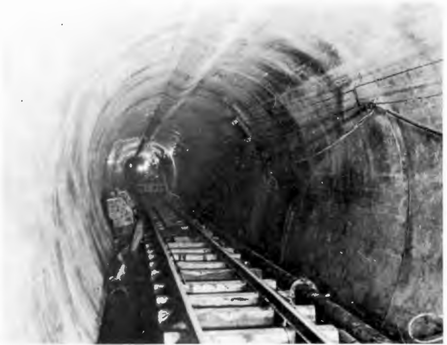
EIGHT FOOT DIAMETER, CONCRETE-LINED TUNNEL — Final cleanup of White's Point 8' diameter, reinforced concrete-lined tunnel. Protrusion down from tunnel crown occasioned by concrete placing spout.
