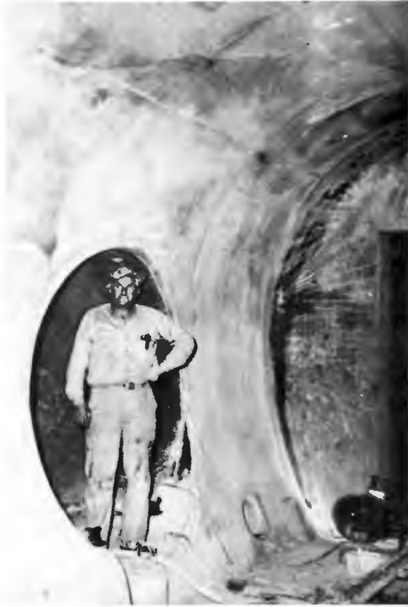
CROSSOVER 12-FOOT TO 8-FOOT TUNNEL— Crossing from twelve to eight foot tunnel for bypass from completed sections of 12-foot sections to 8-foot operating line.
