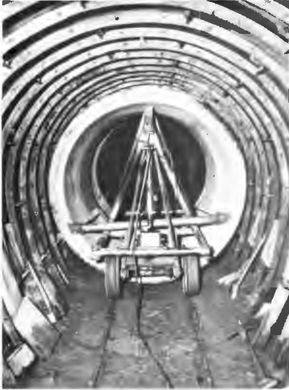
DISTRICT THREE "BACKBONE" TRUNK SEWER—The "backbone" line in District Three, under Eleventh Street, was excavated in sand, supported by steel ribs under corrugated iron. Section of 60-inch diameter R.C. pipe being laid. Space between pipe and lining, grouted.
