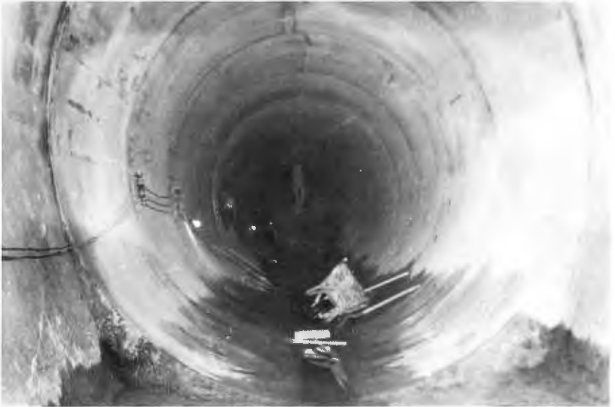
TWELVE FOOT DIAMETER REINFORCED CONCRETE PIPE IN OUTFALL. Upper end of 12-foot diameter line from Bixby to White's Point was constructed of precast R. C. pipe. View shows junction with 12-foot nominal diameter tunnel section at about Vermont Avenue.
