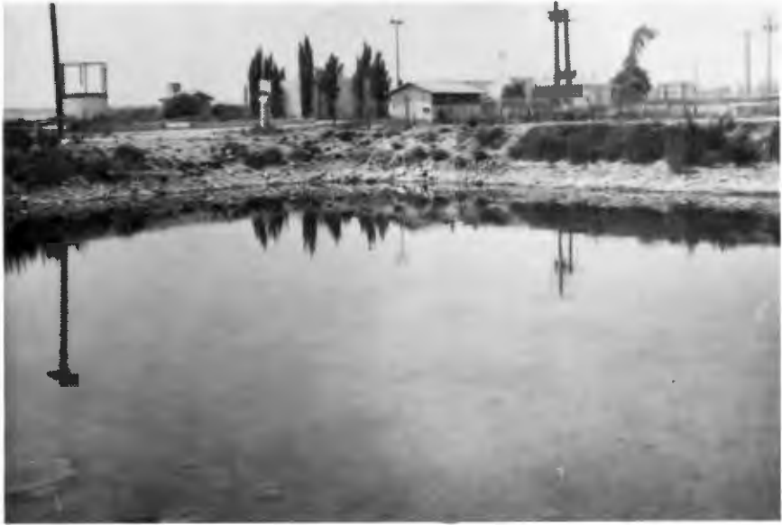
AZUSA PLANT PERCOLATION POND — City of Azusa Sewage Treatment Plant and percolation bed. The plant is being operated as a water reclamation plant by District 15, of which Azusa is a part.
