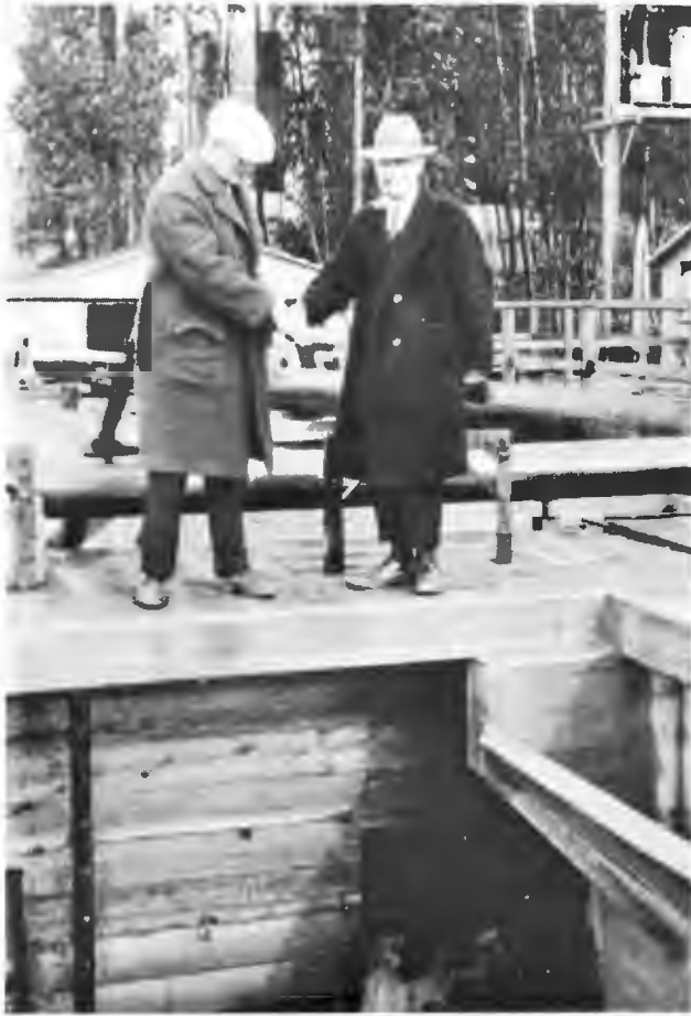
FIRST SEWAGE INTO TEMPORARY PLANT — On February 4, 1928, Chief Engineer Warren opened the gates from the joint outfall into the activated sludge plant at Bixby. The action set the plant in motion which continued—with minor interruptions and difficulties—for nearly ten years. Warren (right), Rawn (left).
