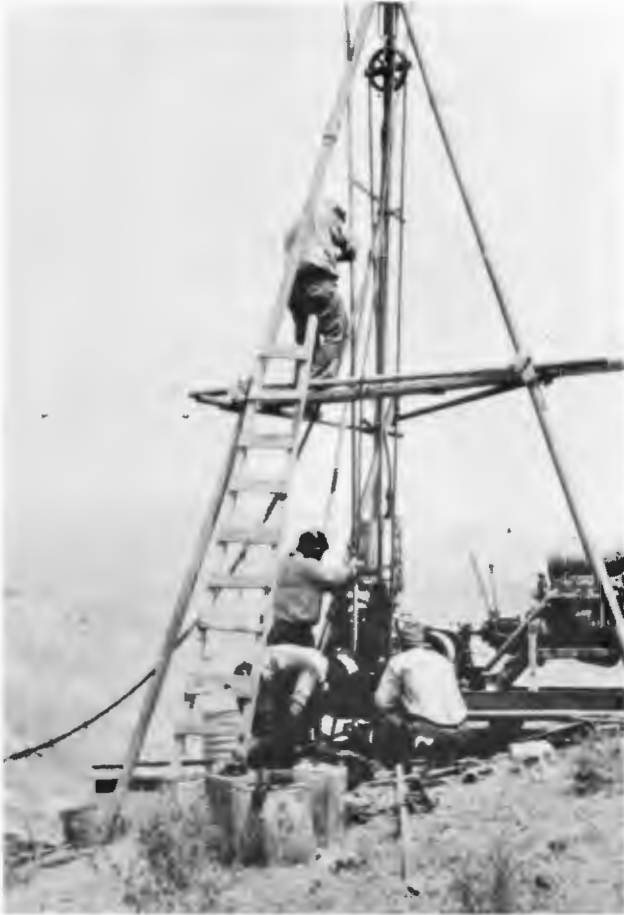
CORE DRILLING WHITE'S POINT TUNNEL, 1933—Where possible, cores were taken of the material to be encountered in excavating the tunnel. A record of all holes at tunnel level was preserved and shown to prospective bidders.
