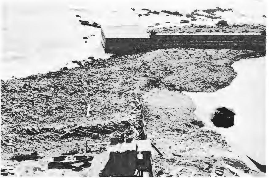
GRAVEL WASHED INTO SWIMMING POOL, WHITE'S POINT—In February, 1926, a storm blew in from the southeast and washed away a fill placed there a few months previously. The rock in the fill was, quite largely, washed into the mouth of a combination swimming pool and small boat harbor.
