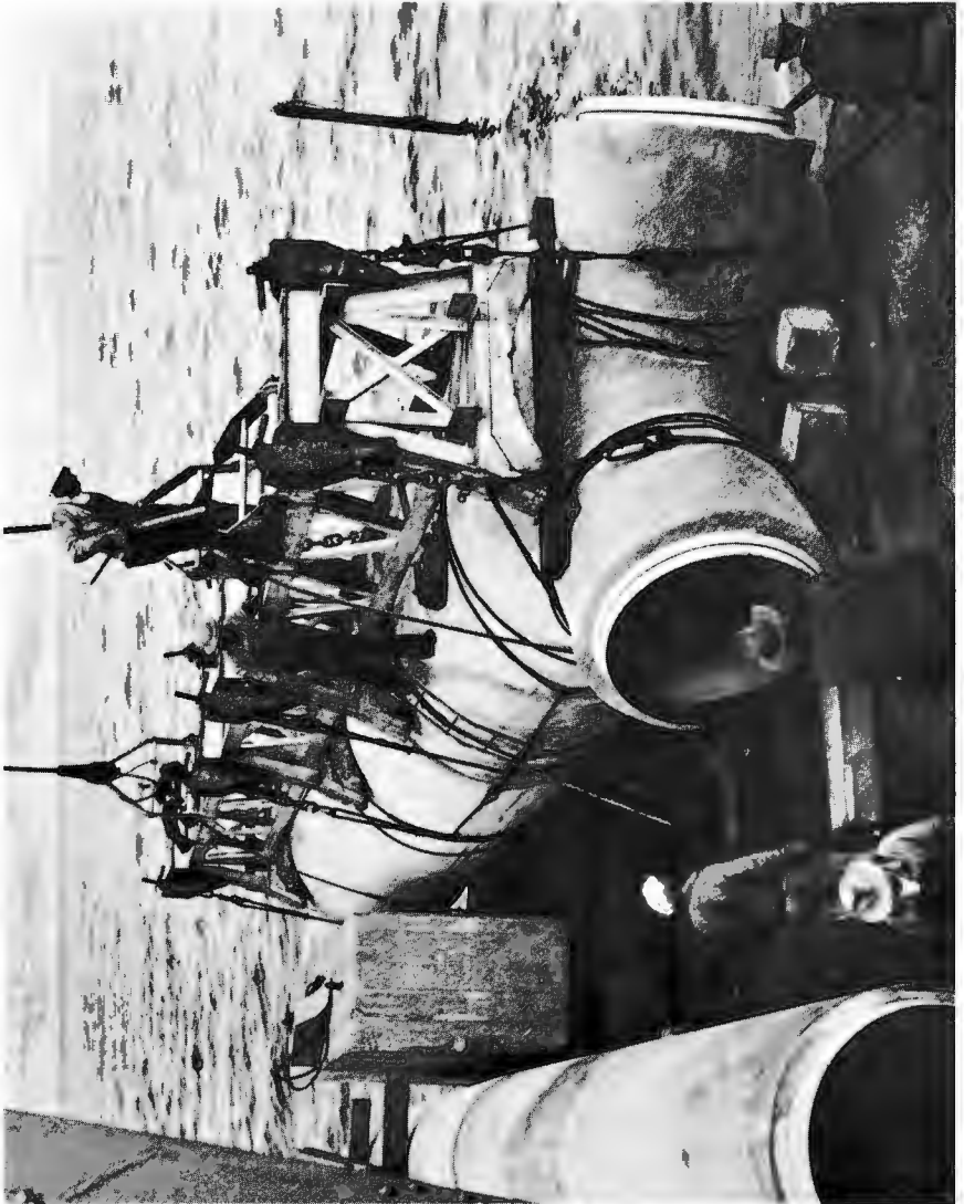
SEVENTY-TWO INCH OUTFALL EXTENSION WYE —The second ocean outfall was extended seaward in 1954, terminating in perforated wye branches 48" in diameter and 216 feet long. Wye section is shown on barge ready for launching.
