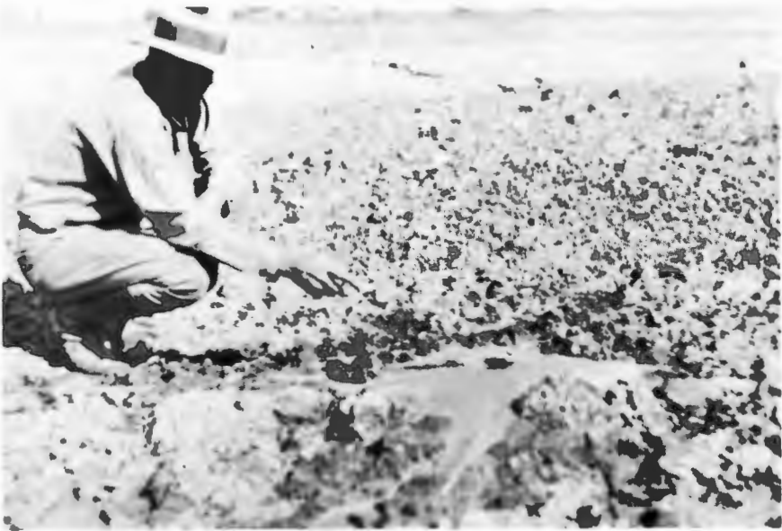
MUD BOIL OVER OUTFALL FOLLOWING EARTHQUAKE —Following the earthquake of March 10, 1933, a number of mud boils, as shown, appeared. Backfill over the trunk sewer had been in place for five years without showing settlement. The structure was not affected in any way.
