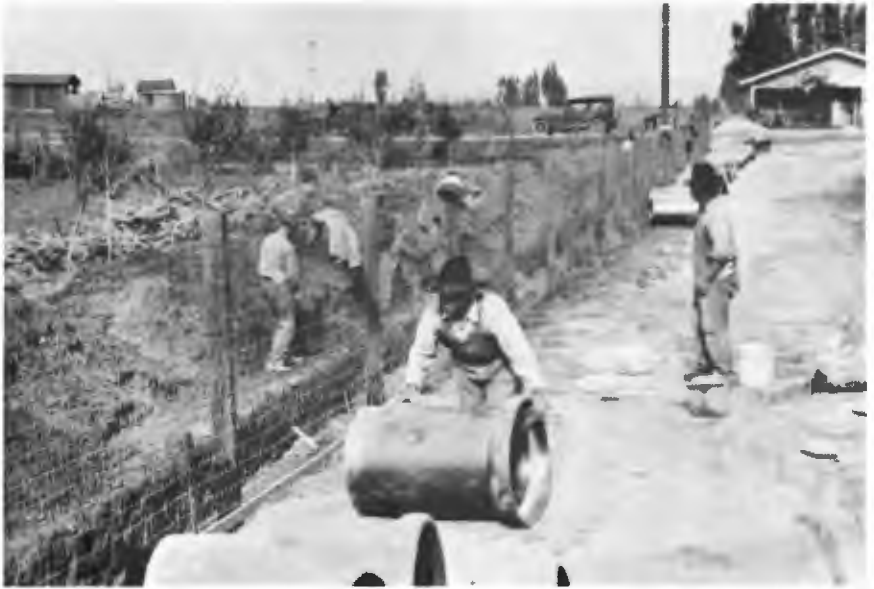
CONSTRUCTION OF MONTEBELLO TRUNK — Picture shows condition of development in late '20s. Area now densely developed.
