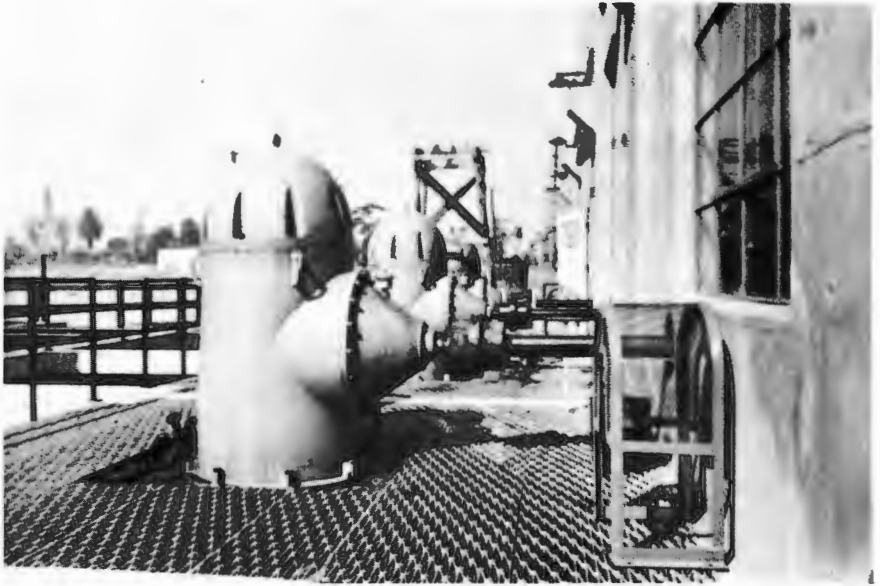
FOUR GAS ENGINE PUMPS, 1948 — Effluent pumps at Bixby. Four of these units were installed. Power furnished by sludge gas, internal combustion engines connected through angle gears. Gas engines originally purchased were unsatisfactory and were rejected and replaced by others.
