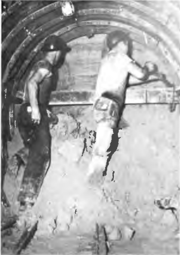
EXCAVATING "BACKBONE" SECTION THREE—Excavation in heading of tunnel under Eleventh Street, Long Beach. Excavation continued in three shifts daily. Three men to a shift at night, and enough during day shift to remove excavated material from access shafts and furnish night shifts with lining and well point material and equipment.
