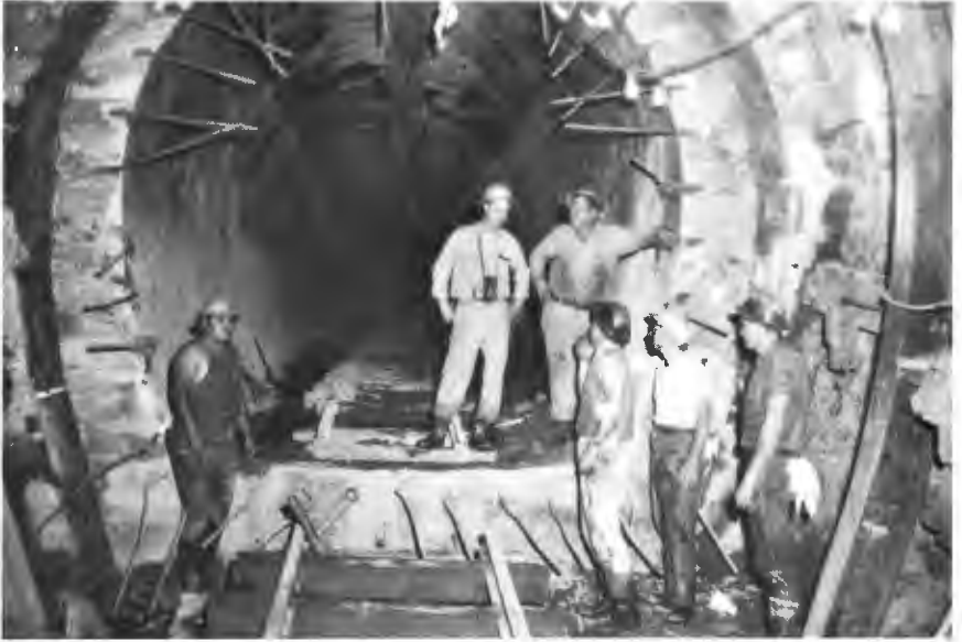
TWELVE-FOOT DIAMETER TUNNEL UNDER CONSTRUCTION — Cross section of 12-foot tunnel lining. Note how the tunnel support is embedded in concrete. Picture taken at connection point of finished tunnel with Section 4.
