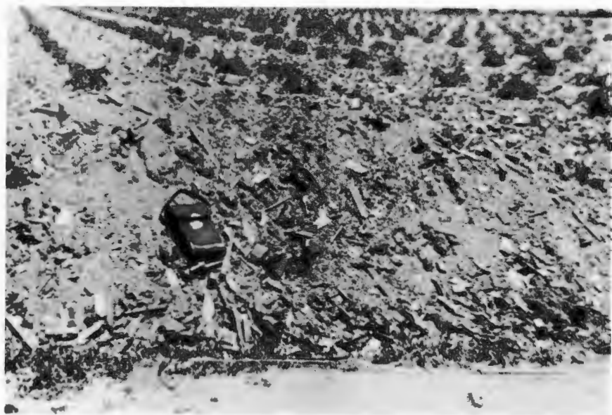
TRASH AND CLAY LINERS REMOVED FROM BULLIS ROAD TRUNK—Action of hydrogen sulfide gas, oxidized on the sewer walls, penetrated through the vitrified clay liners and forced the liners free from their bond to the concrete.
