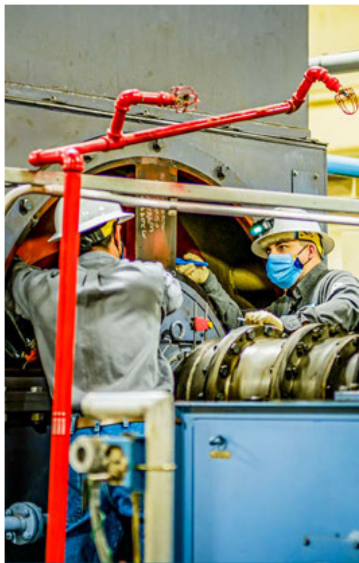
Electricians maintain equipment at the Warren Facility.
