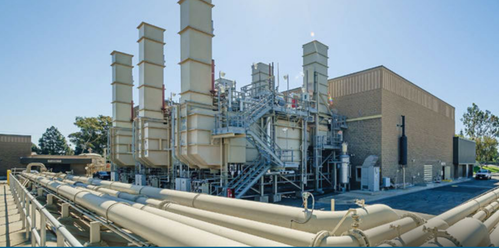
Total Energy Facility.
