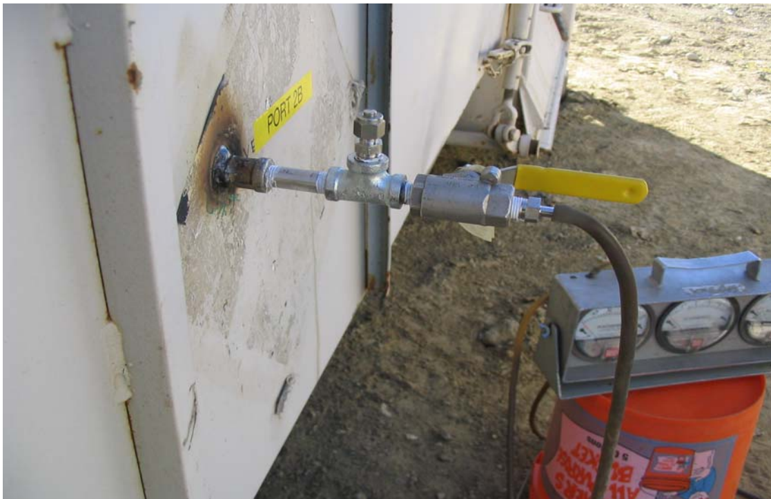
Photo 4 – Interior pressure monitoring
