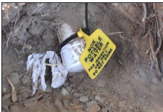
Non-potable water identification tag (yellow)
