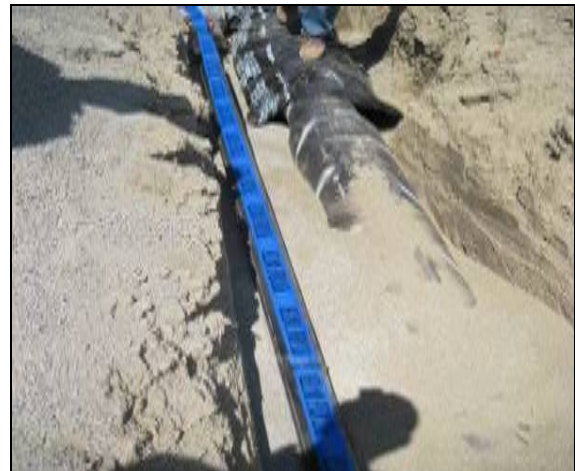
6-inch potable water HDPE mainline with POTABLE WATER identification tape affixed
