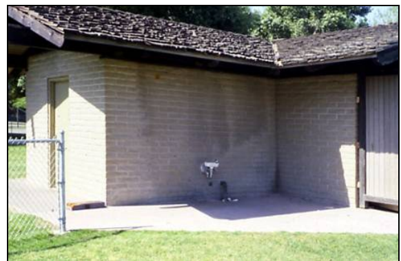
The pattern on the walls indicates that this drinking fountain is being sprayed by the irrigation water. If recycled water is to be used, then the spray pattern must be altered or the drinking fountain somehow shielded.
