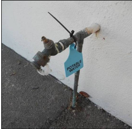
Potable water hose-bib with a POTABLE WATER identification tag
