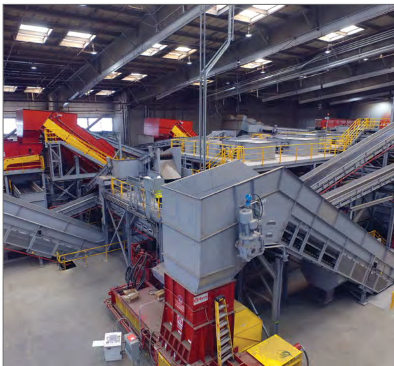
A new automated sorting line will improve efficiency and increase the purity of recyclables.
