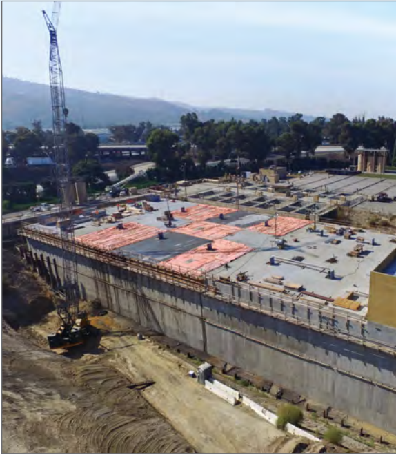
Construction of the 8-million-gallon Flow Equalization Tank at San Jose Creek WRP West.
