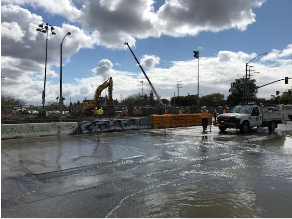
Figure 3: Street flooding on Figueroa Street at 0930 hours on 3-19-2020.
