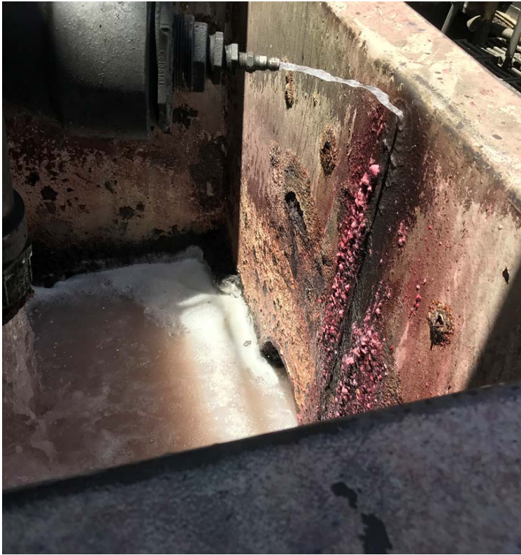
Figure 4: Primary grit chamber tank at Lancaster WRP on 6-30-2020. Note the pink color.
