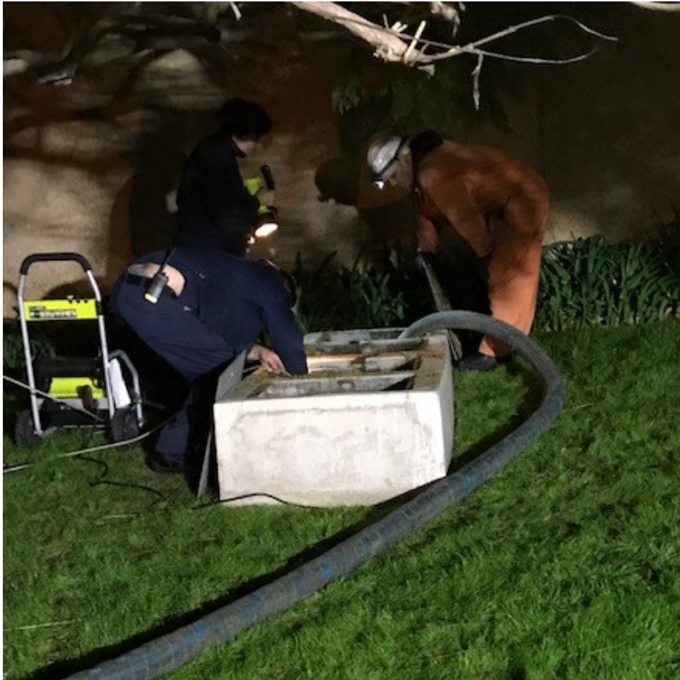
Figure 2: Clarifier at The Gill Corp being serviced on the evening of 1-21-2020 to remove accumulated hydraulic oil.
