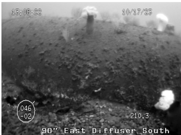
Figure 45: Area of partial undercutting, 5 th pipe section from the terminus, on the south side of the east diffuser leg of the 90-inch outfall.
