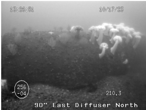
Figure 41: Area of partial undercutting, 2 nd pipe section from the terminus, on the north side of the east diffuser leg of the 90-inch outfall.
