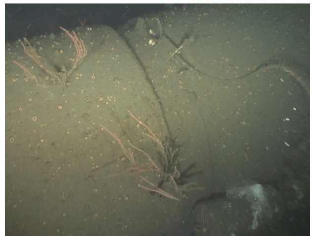
Figure 13: A cast iron joint with a concrete collar on the 72-inch outfall.
