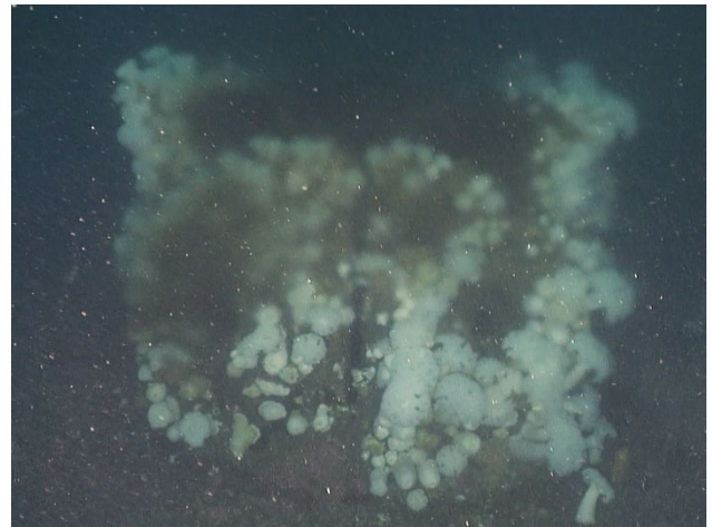
Figure 31: Terminus ports located within the gravity door of the end structure on the 120-inch outfall.
