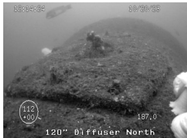
Figure 35: Detached anode on the 120-inch outfall.
