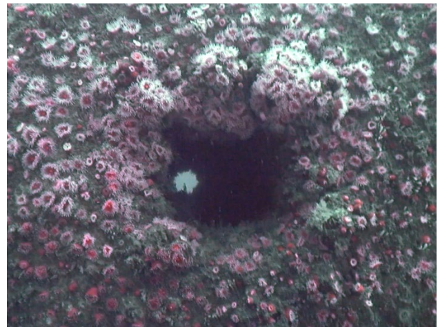
Figure 17: Diffuser port looking through to other side of the pipe section on the 60-inch outfall.
