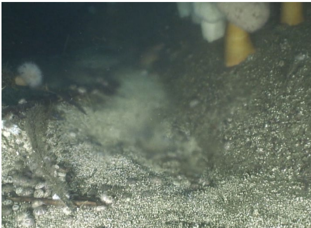
Figure 23: A buried port with reduced flow (weeping), 15 th from the terminus, on the north side of the 120-inch outfall.
