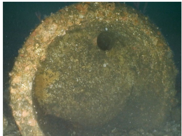
Figure 53: Terminus port on the east diffuser leg of the 72-inch outfall.
