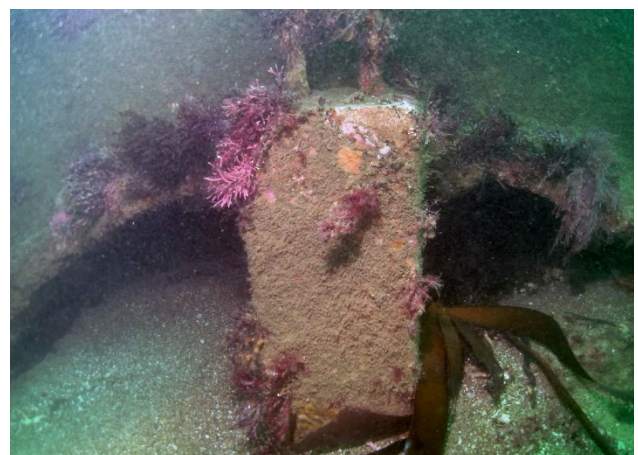
Figure 10: West side of j-box designed to provide an option for adding a second main barrel to the 90-inch outfall.
