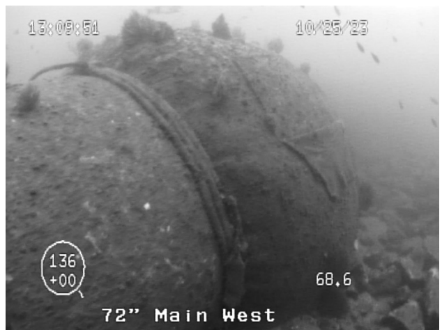
Figure 56: Encapsulated joint on the 72-inch outfall.
