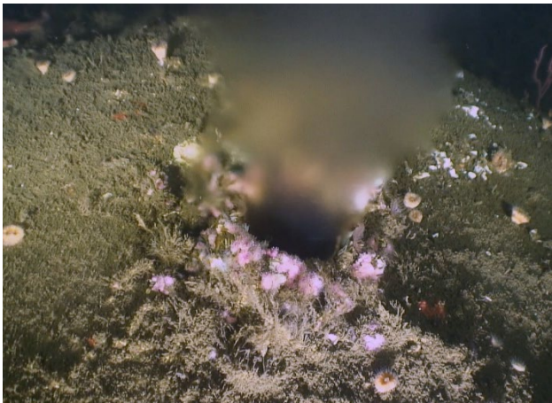
Figure 11: Vertical port with barnacle collar on the 90-inch outfall.
