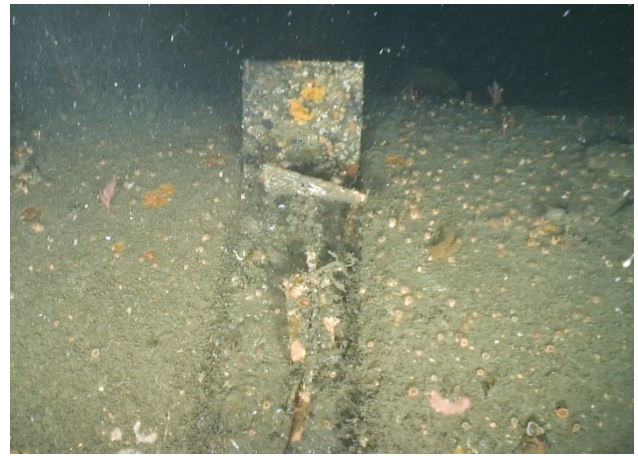
Figure 8: A cast iron joint wrapped with a hard rubber gasket and attached anode cable on the 90-inch outfall.
