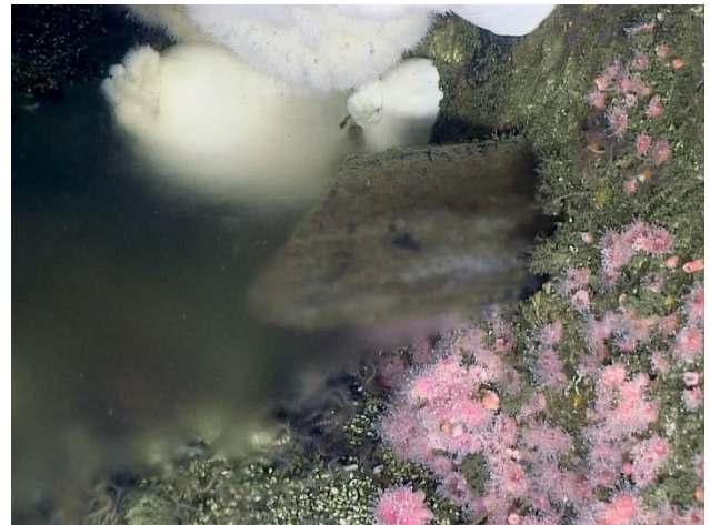
Figure 25: A partially blocked port, 8 th from the terminus, on the south side of the 120-inch outfall.
