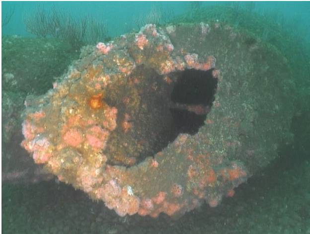
Figure 59: Partially corroded steel plate covering the east jet of the tri-jet end structure on the 60-inch outfall.
