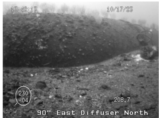
Figure 46: Area of partial undercutting, 10 th pipe section from the terminus, on the north side of the east diffuser leg of the 90-inch outfall.
