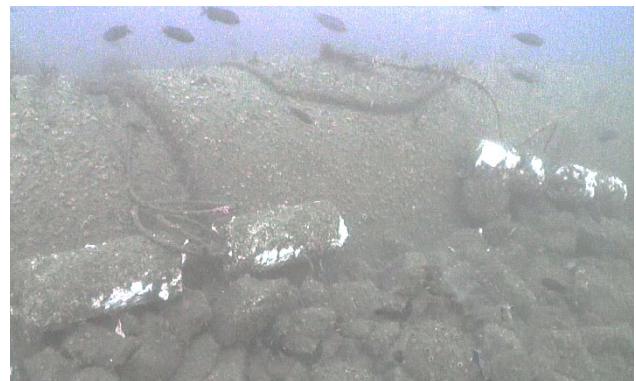
Figure 2: Overview of joint and flush manhole cover to cable connections and aluminum anodes to cable connections with anodes located within the ballast rock.
