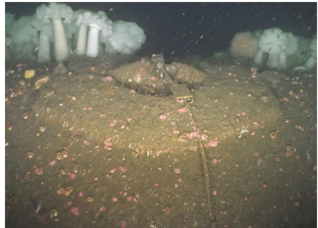
Figure 4: A flush manhole cover on the 120-inch outfall. This type of manhole cover is also on the 90- and 72-inch outfalls.
