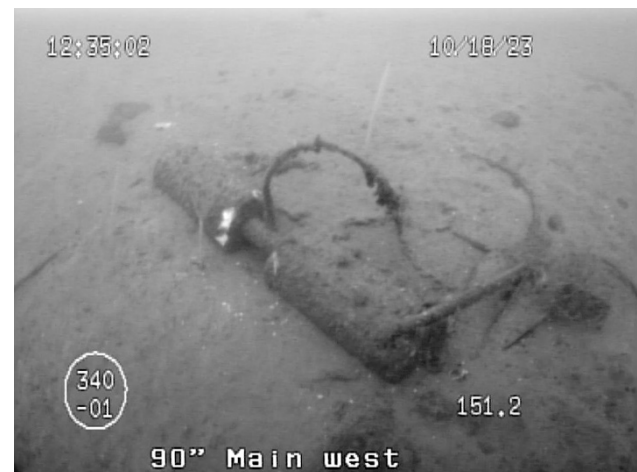
Figure 50: An anode that was previous reported missing entangled with a boat anchor several feet off of the 90-inch outfall.
