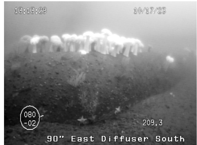
Figure 42: Area of partial undercutting, 2 nd pipe section from the terminus, on the south side of the east diffuser leg of the 90-inch outfall.
