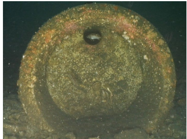
Figure 52: Terminus port on the west diffuser leg of the 72-inch outfall.
