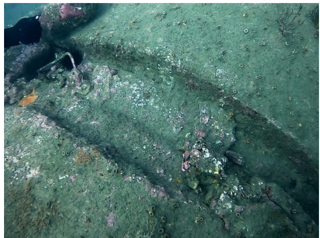
Figure 55: Deteriorating joint collar on the 72-inch outfall.
