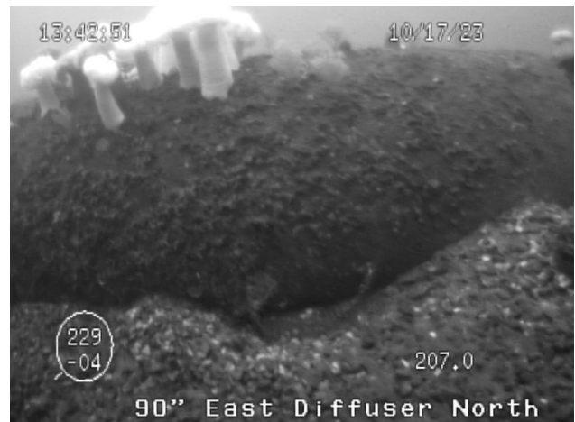
Figure 48: Area of partial undercutting, 12 th pipe section from the terminus, on the north side of the east diffuser leg of the 90-inch outfall.
