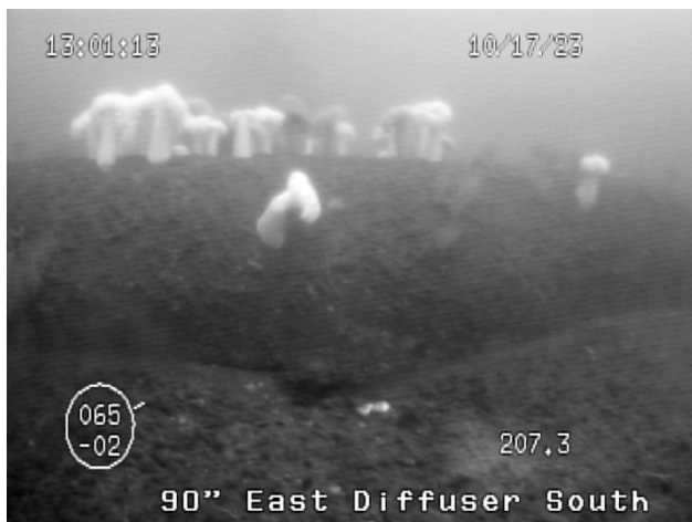
Figure 49: Area of partial undercutting, 12 th pipe section from the terminus, on the south side of the east diffuser leg of the 90-inch outfall.
