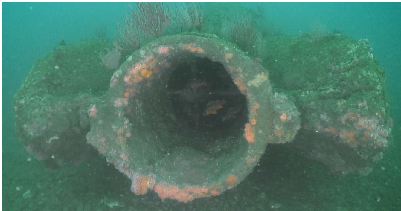
Figure 57: Tri-jet end structure of the 60-inch outfall showing the stainless steel crossbar within the middle jet. Little to no ballast material remains supporting the structure.
