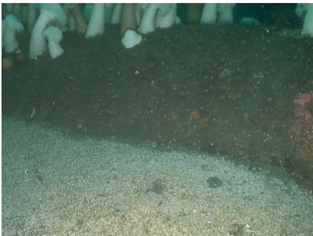
Figure 30: A buried port with no flow, 21 st from the terminus, on the south side of the 120-inch outfall.
