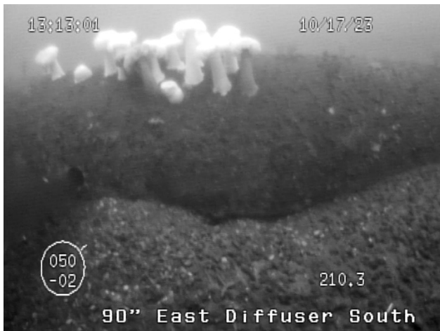
Figure 43: Area of partial undercutting, 3 rd pipe section from the terminus, on the south side of the east diffuser leg of the 90-inch outfall.
