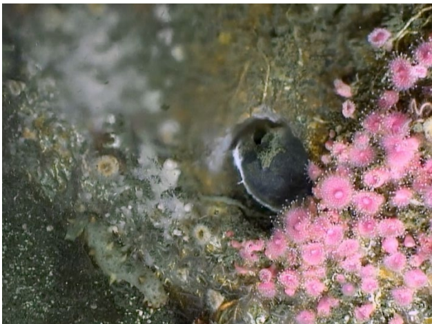
Figure 24: An internally blocked port with reduced flow, 7 th from the terminus, on the south side of the 120-inch outfall.
