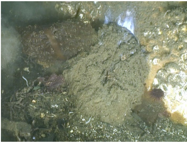
Figure 37: A partially blocked port with substantially reduced flow, 3 rd from the terminus, on the north side of the east diffuser leg of the 90-inch outfall.
