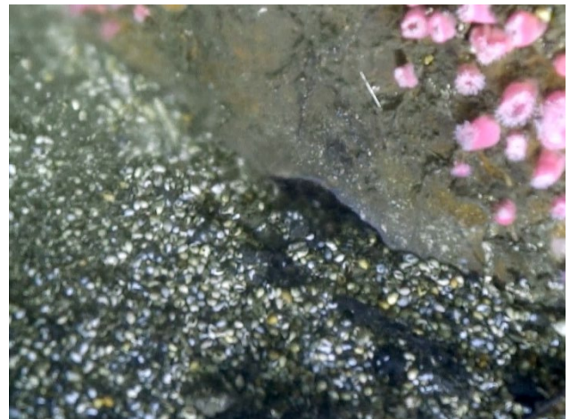
Figure 27: A partially buried port with reduced flow, 12 th from the terminus, on the south side of the 120-inch outfall.
