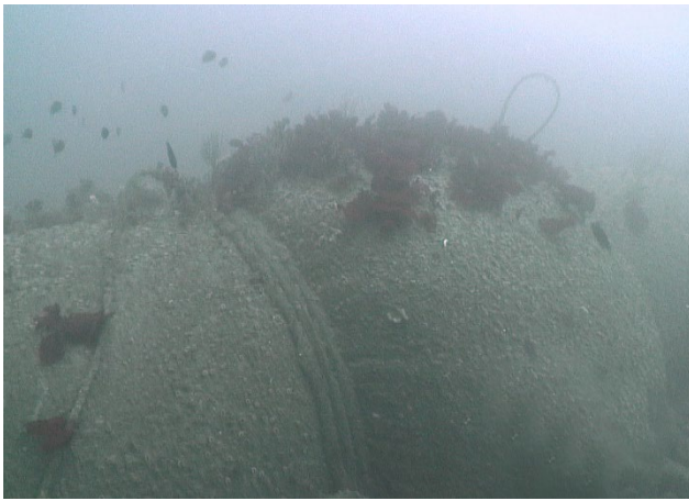
Figure 14: Encapsulated joint on the 72-inch outfall.
