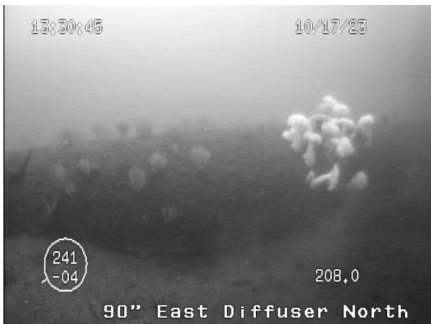
Figure 44: Area of partial undercutting, 4 th pipe section from the terminus, on the north side of the east diffuser leg of the 90-inch outfall.
