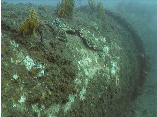
Figure 65: Area of spalling on the 60-inch outfall.
