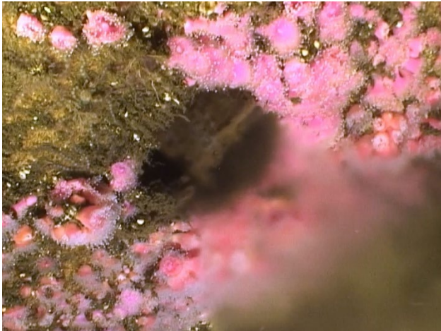
Figure 29: A partially blocked port, 20 th from the terminus, on the south side of the 120-inch outfall.
