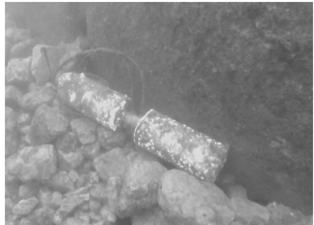
Figure A2: Aluminum anode, approximately four feet in length, residing within ballast rock along the west side of the 90-inch outfall. The joint connection is located on the top of the outfall.
