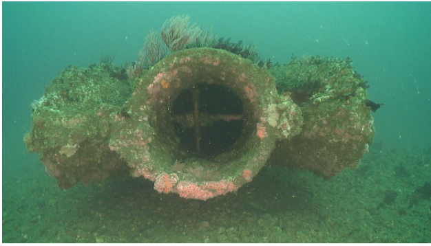
Figure 18: The tri-jet end structure of the 60-inch outfall with detached support girder.
