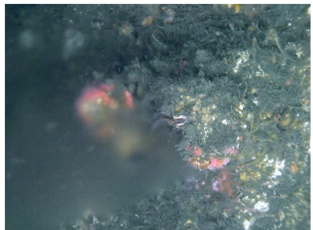
Figure 32: Barnacle collar formed around a port on the 120-inch outfall. Effluent flow does not appear to be altered by these collars.
