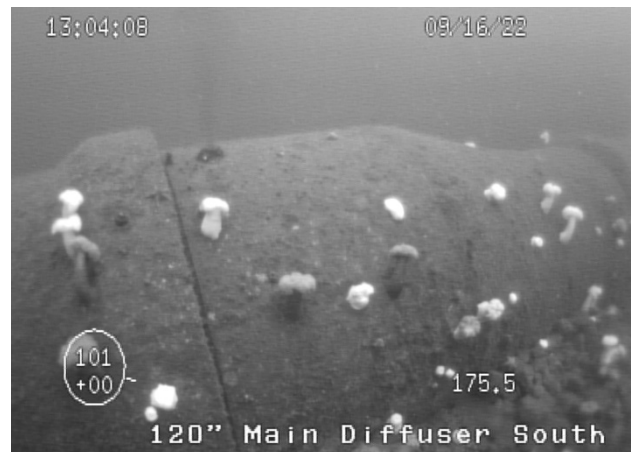
Figure 6: Vertical port on the 120-inch outfall. This port is located on a section reducing the diameter of the diffuser pipe from 120 to 102 inches.
