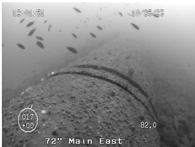
Figure 54: Cracked joint collar on the 72-inch outfall.
