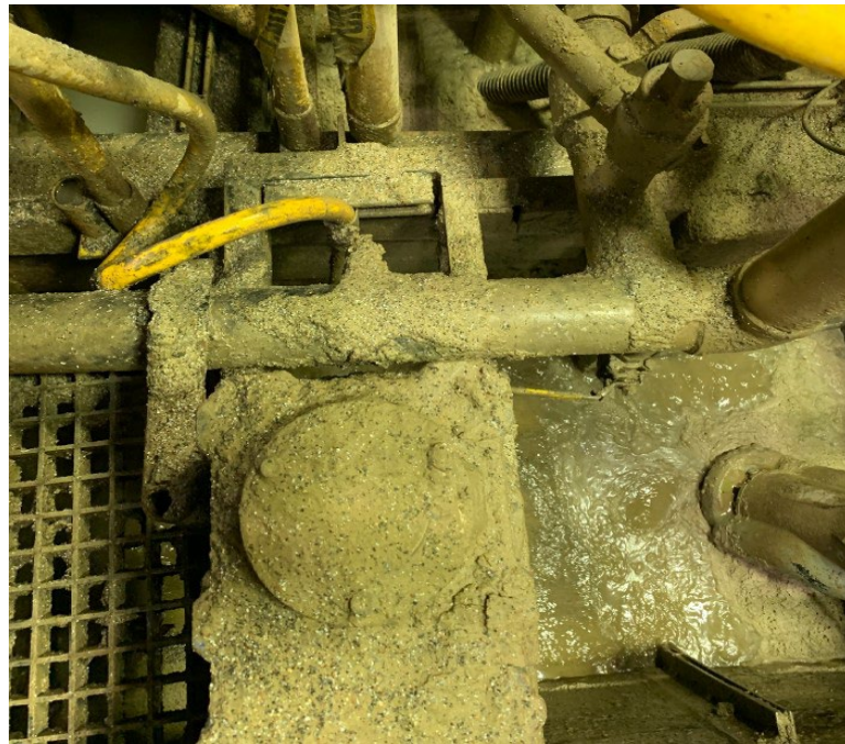
Figure 4. Sand in the collection pit at Owens Corning.
