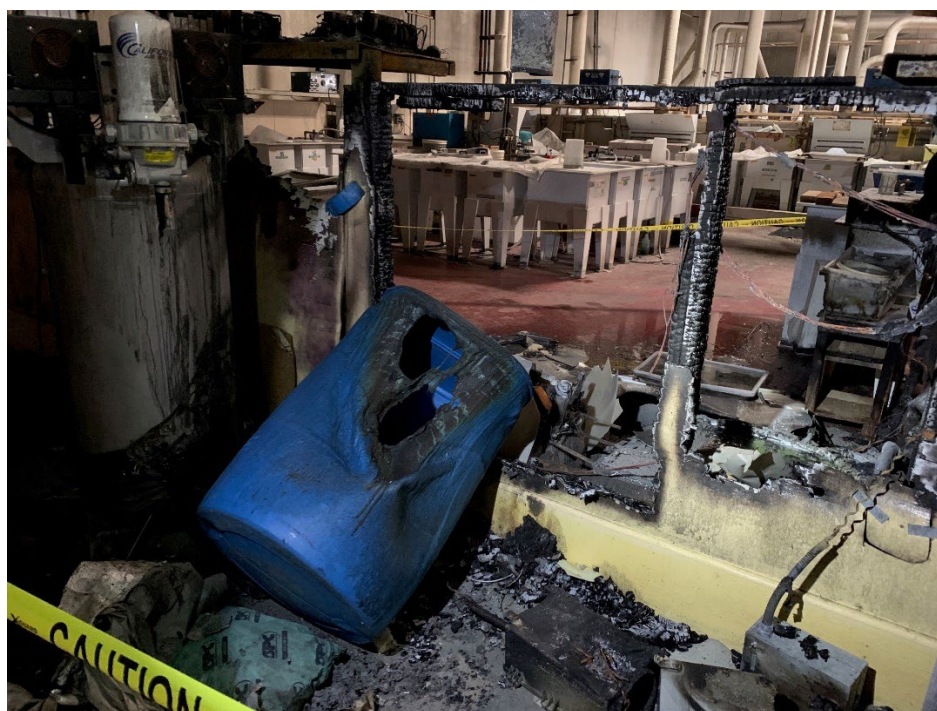
Figure 1. Fire-damaged gold plating line.
