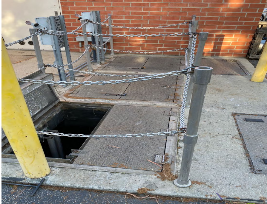
Figure 2. Submersible Side of Long Beach Interceptor Pump Plant
