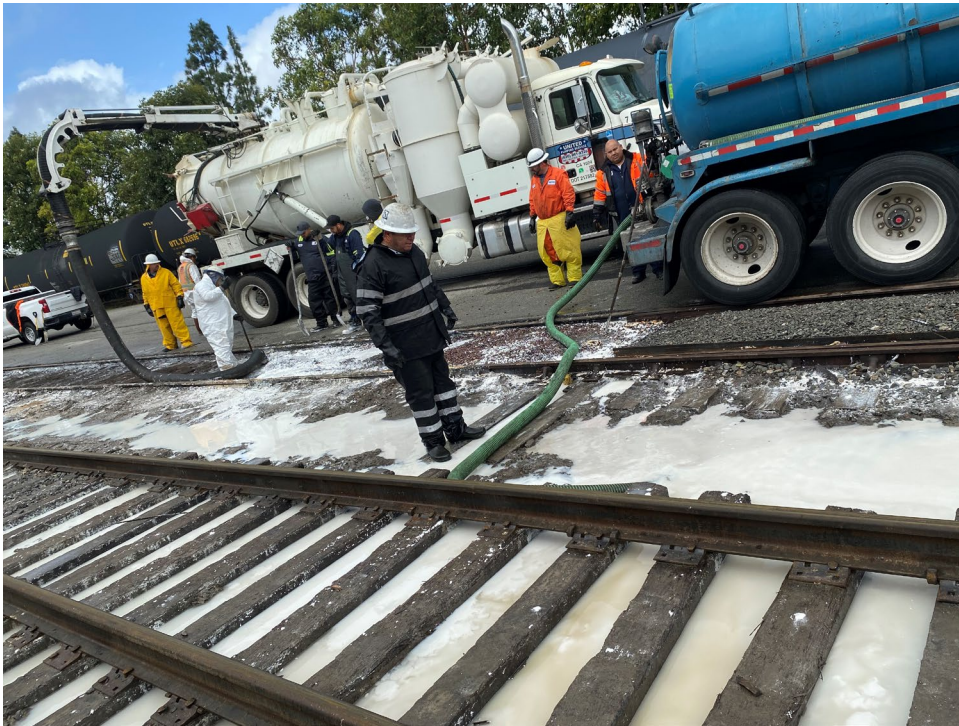
Figure 2: White Latex Paint Spill Clean Up
