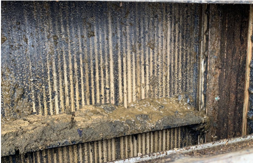
Figure 13. Heavy grease/solids impacting JWPCP J.O."A" bar screens.
