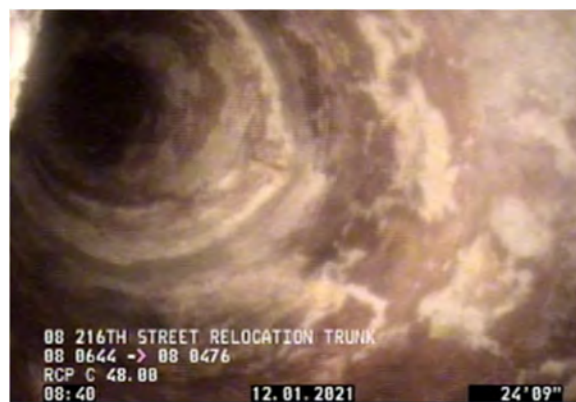
Photo 3-3 CCTV Inspection Photograph 3
