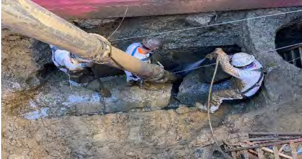
Photo 3-7 Pipe Condition When First Exposed
