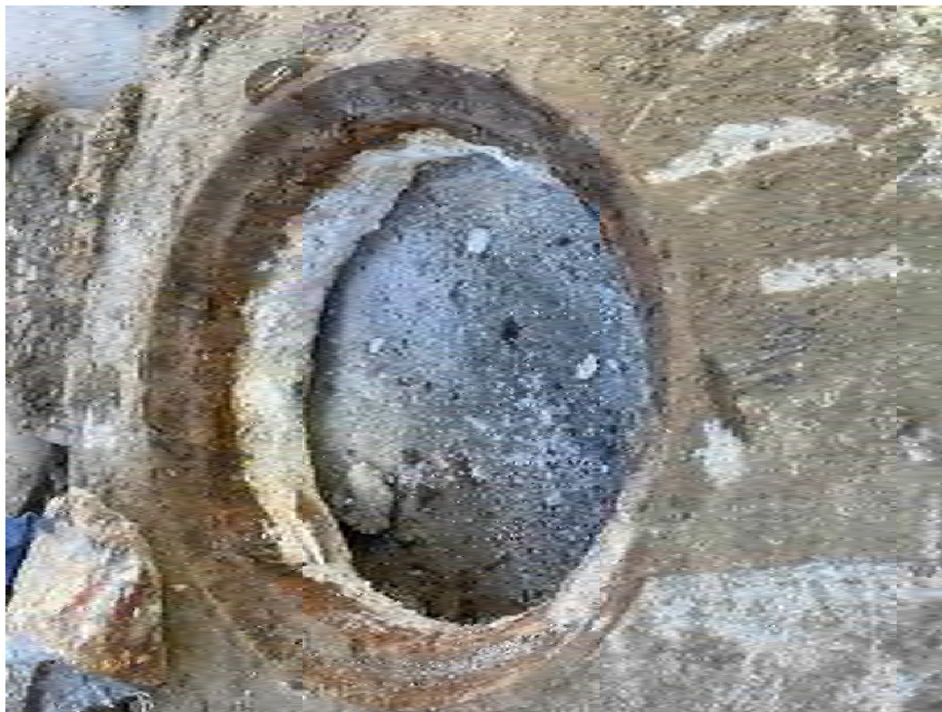
Photo 3-12 Manhole Ring and Cover Debris
