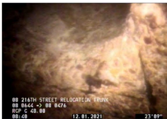
Photo 3-2 CCTV Inspection Photograph 2
