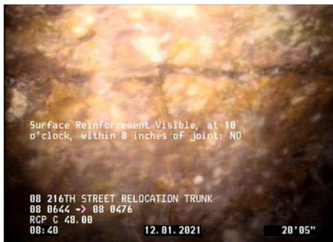
Photo 3-1 CCTV Inspection Photograph 1
