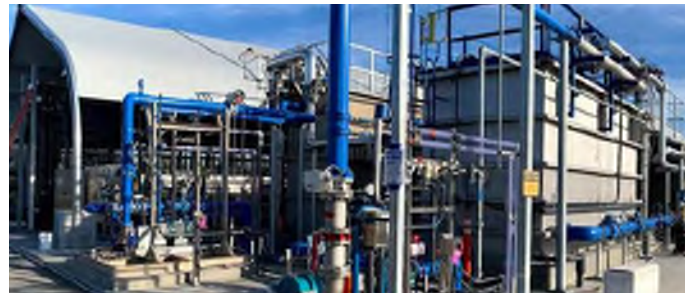
Metropolitan Water District of Southern California's Advanced Purification Center.
