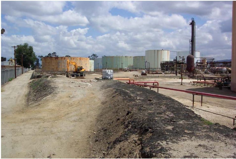
Figure 3: Large, old refinery tanks at the Ridgeline facility which are in the process of being emptied and demolished.
