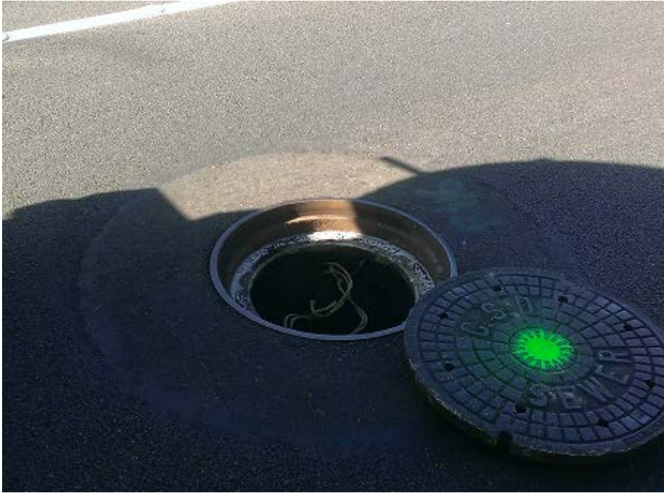
Figure 2: MH 02 F 0086 on the J.O. ‘F’-unit 4 trunk in Norwalk where the unusual smoking effect was observed.
