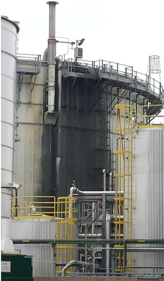
Figure 1: 2 MGD digester tank at the Ralphs' facility in Compton. Note dark staining on the side of the tank where foam from the tank has overflowed.
