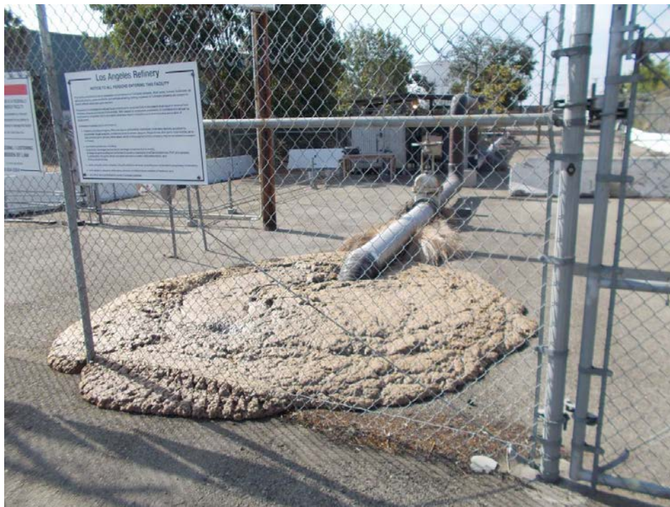
Figure 1: Thick brown foam overflowing the industrial wastewater discharge manhole at the Phillips 66 oil refinery at 0930 hours on 9-3-14.
