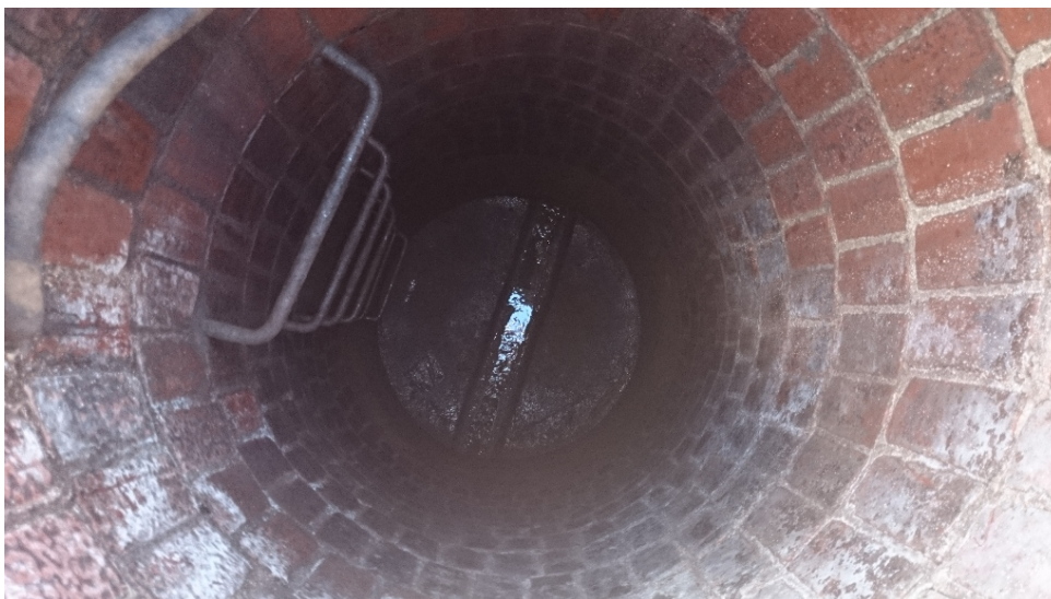
Figure 2: View into local sewer line manhole shown in Figure 1. Note the lack of oil or oily residue that would be expected if the manhole were being regularly used to dispose of waste oil.
