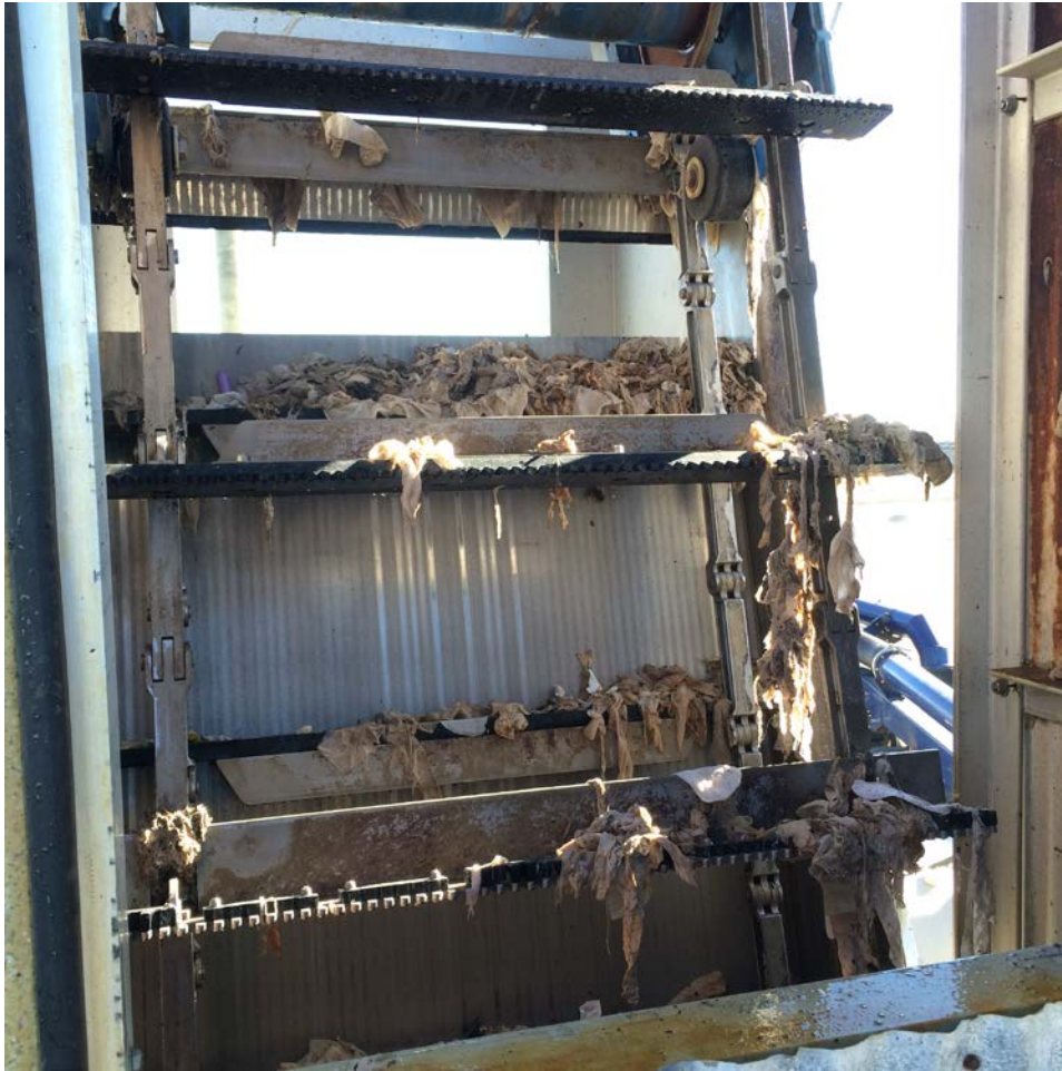
Figure 11: Excessive ragging on the flex rake screen at Lancaster WRP on 12-29-14.
