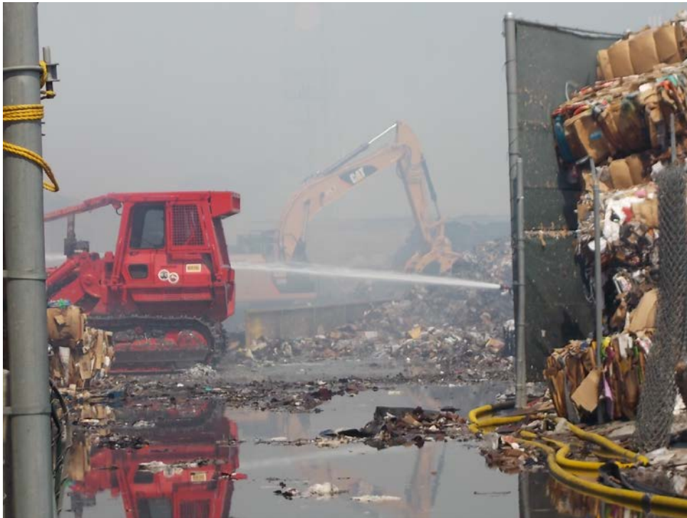
Figure 5: Fire Department heavy equipment working on 5-30-14 to expose and extinguish burning materials in tightly packed waste paper bales at the Pan Pacific Fiber facility. Note the large amount of firewater runoff being generated by this effort.
