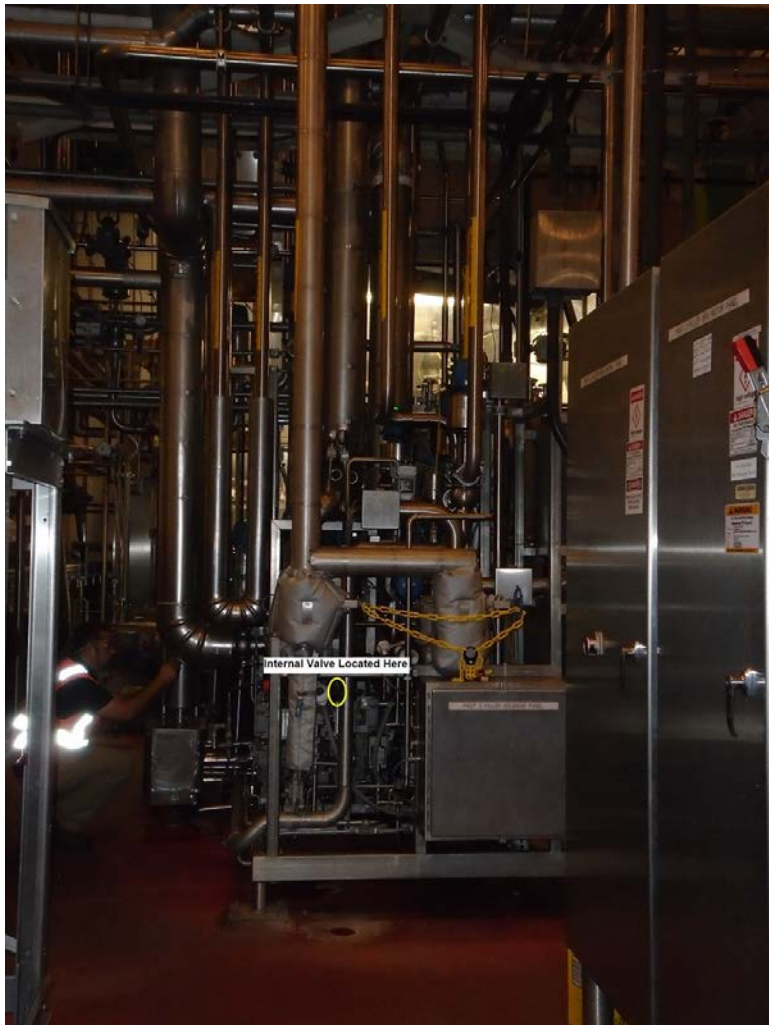
Figure 1: Tropicana filling line #2 filler bowl manifold. Note the location of the internal valve that failed and the floor drain immediately beneath that received the leaking juice.
