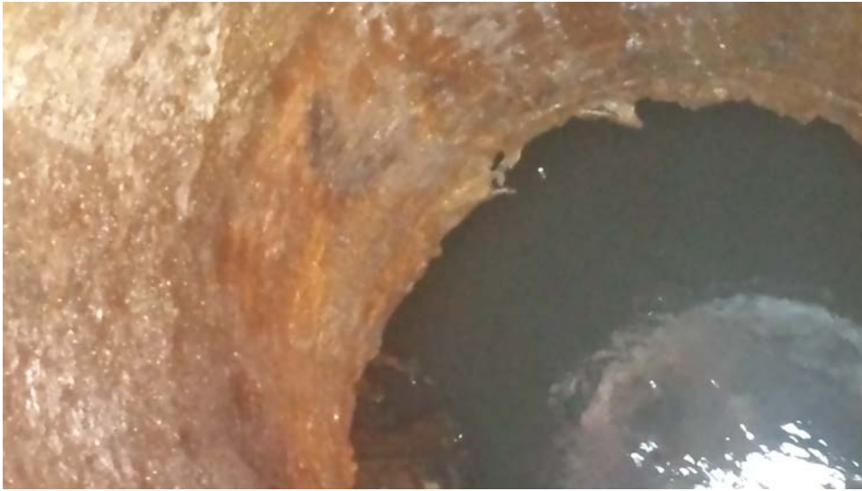
Figure 11: 4-27-15 photo of the interior of manhole 03 0427 on the Water Street trunk in Long Beach. Note the orange tint of the epoxy liner.
