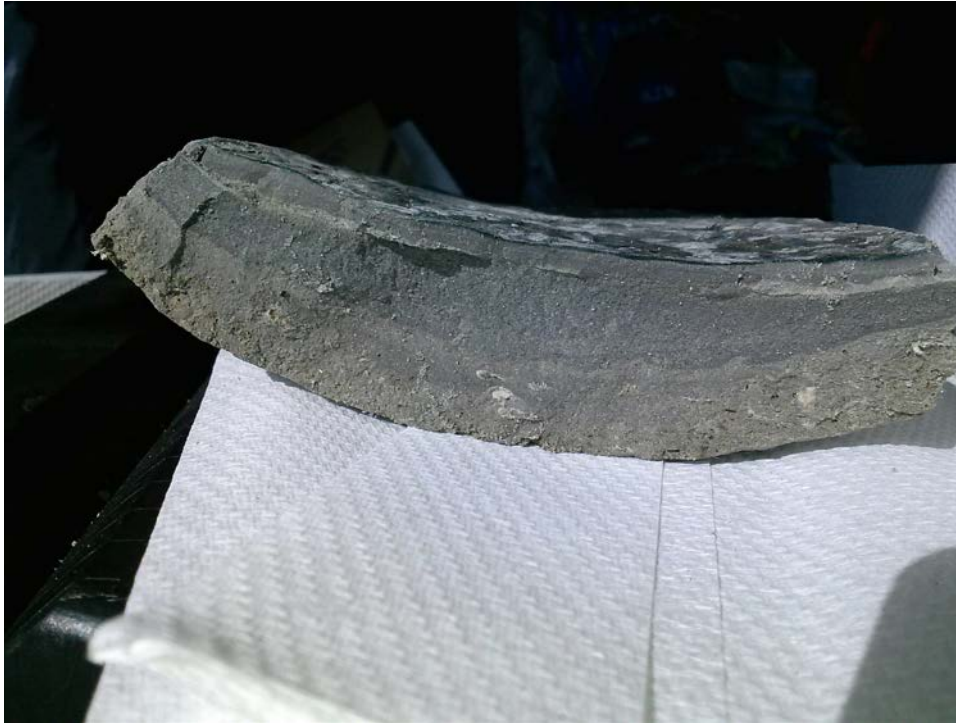
Figure 8: Layered concrete removed from Long Beach local sewer line by hydroblasting operations by National Plant Services on 2-15-15.
