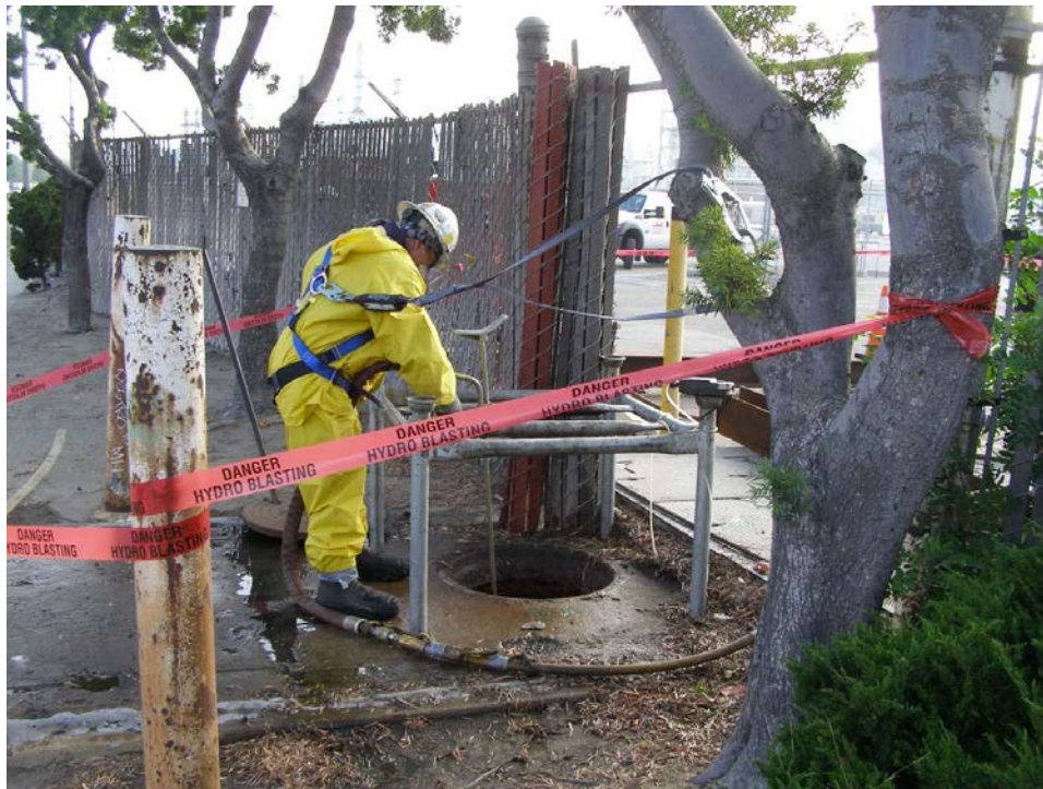
Figure 3: Worker accessing manhole B18A on 8-24-15 to hydrojet the Tesoro Refinery's line where it connects to the J.O. 'B' trunk (Photo by Districts' I.W. Inspector Shawn Cleaver).
