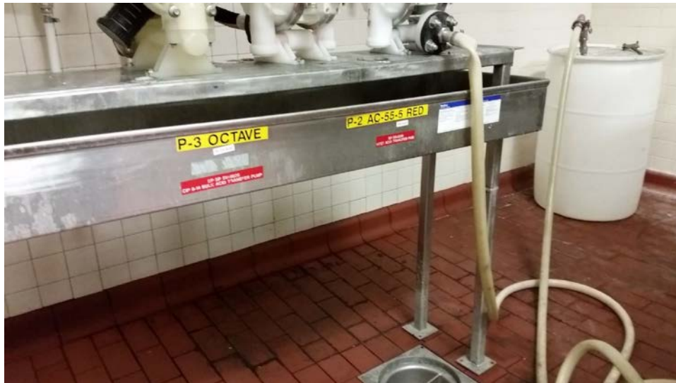
Figure 1: CIP system pump room at General Mills on 2-15-15. Note the diaphragm pumps above and the open floor drain directly beneath where the spilled acid entered the facility's industrial wastewater collection system.
