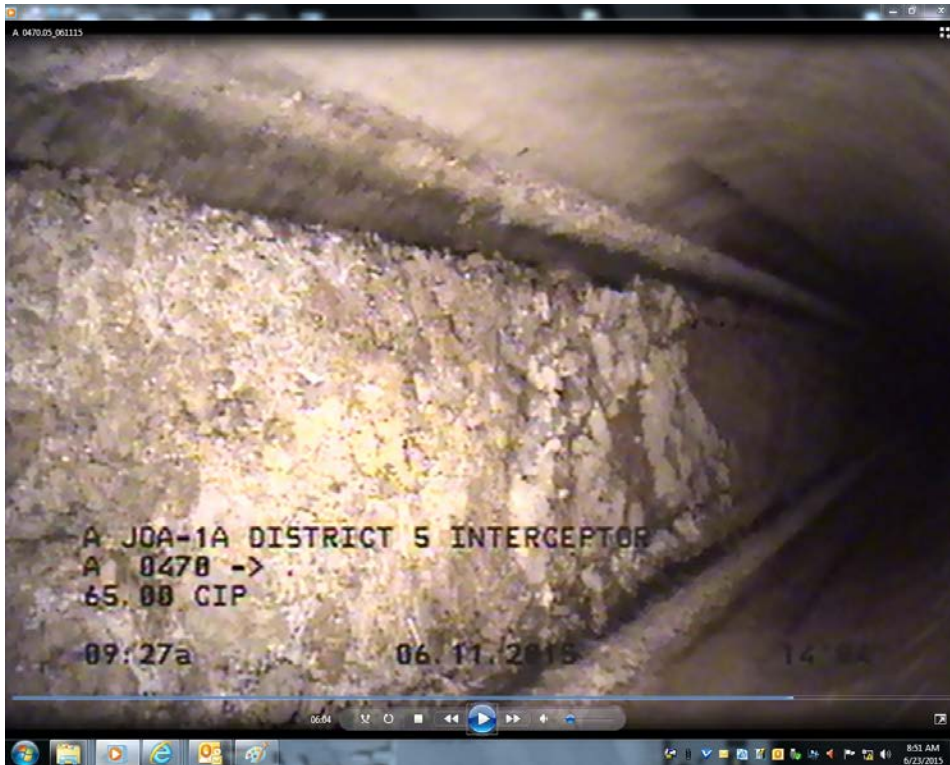
Figure 6: CCTV video screen grab photo of the FOG CCTV sewer crews encountered at MH 08A0470 on 6-11-15.
