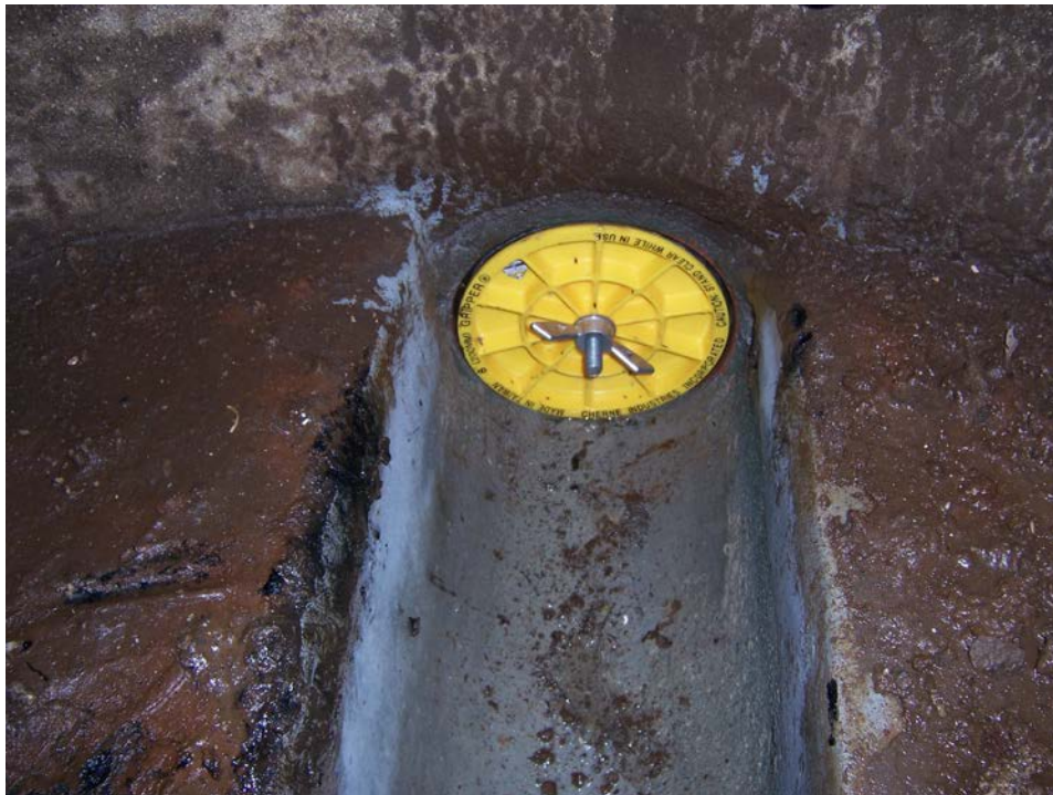
Figure 3: 8" diameter sewer line expansion plug installed by IEUA on 6-17-15 which effectively sealed Starlite Reclamation's I.W. connection.
