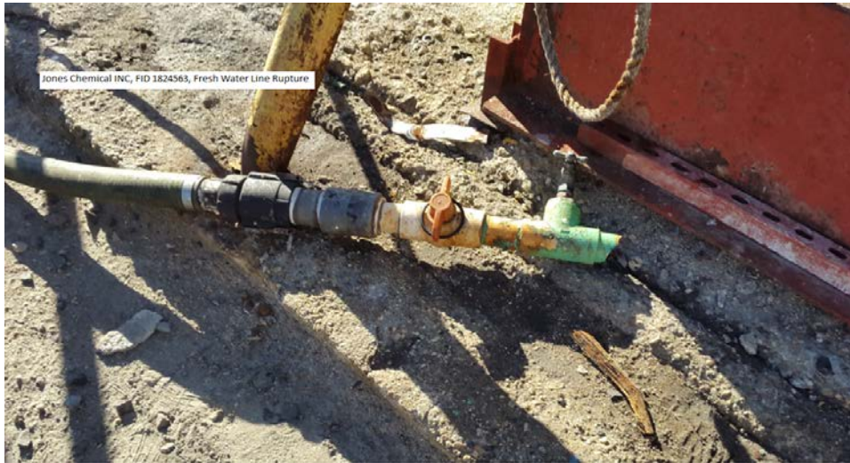
Figure 6: Broken potable water line. Note the valves which were quickly closed to limit the spill volume.
