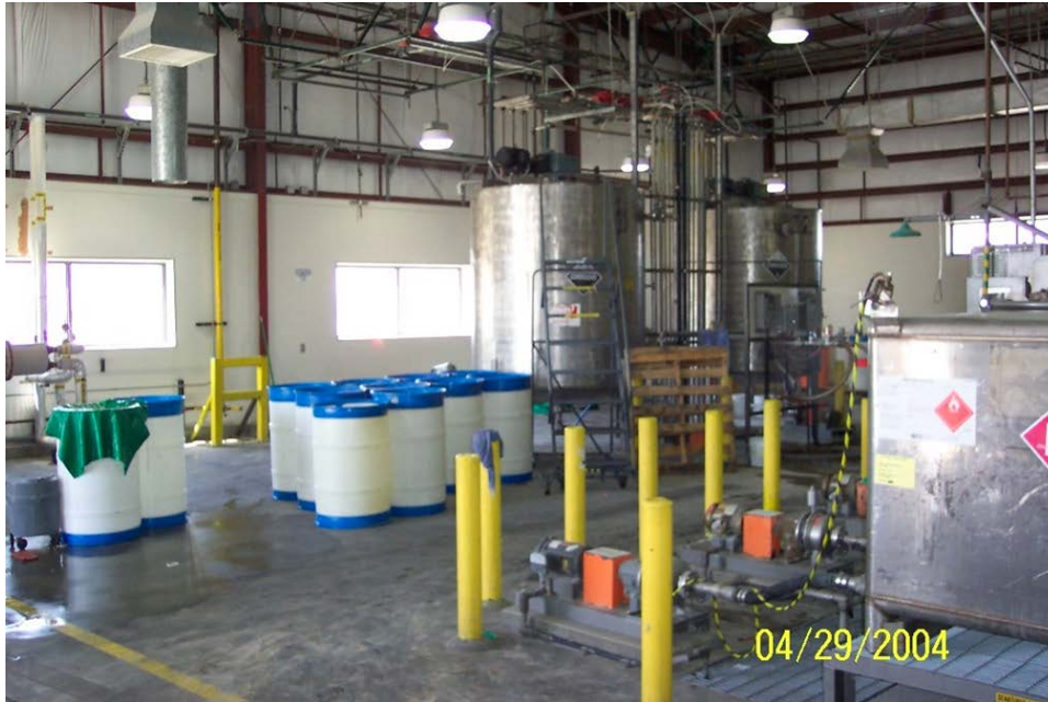
Figure 6: 2004 photo of the Prison Industry Authority soap and detergent manufacturing facility at the Lancaster State Prison facility.
