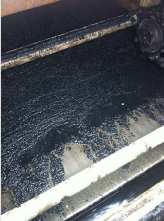
Figure 11: JWPCP Primary skimmer black solids observed on 7-30-15. Note how the solids, which come from the JWPCP Solids Processing Unit appear essentially visually identical to that of a black oily material.
