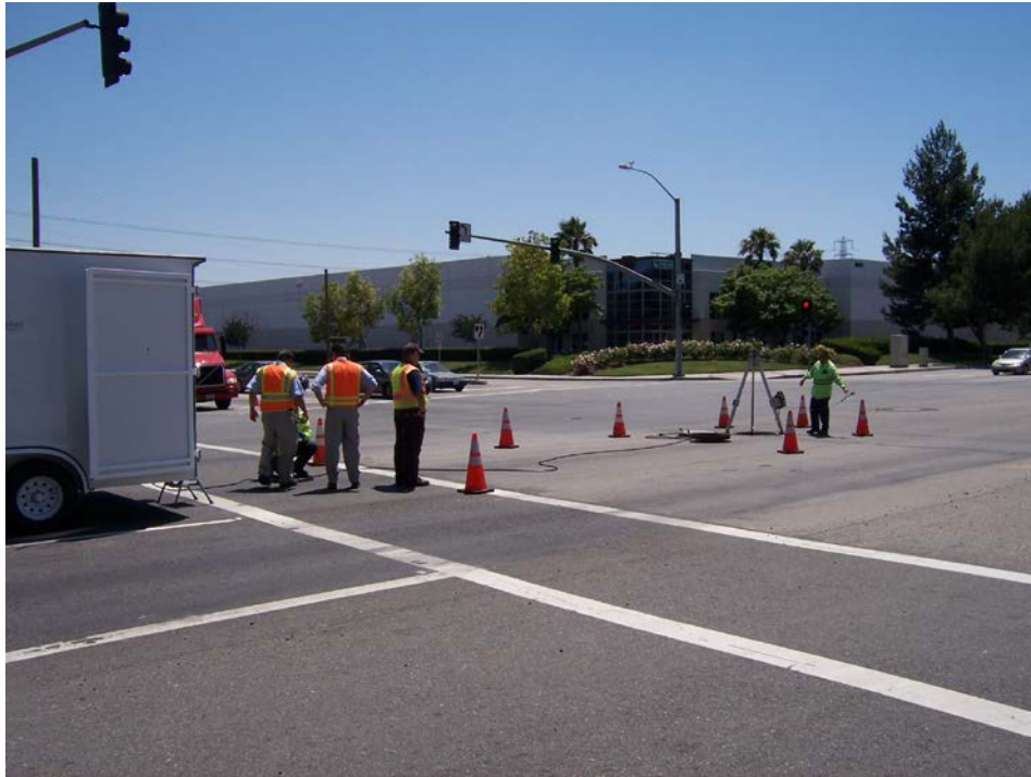
Figure 2: IEUA sewer maintenance personnel preparing to enter the manhole where they sealed the I.W. connection line from Starlite Reclamation Environmental Services, Inc. on 6-17-15.
