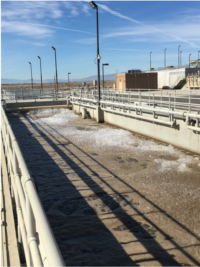
Figure 8: White foam lingering in the secondary treatment aeration tanks at the Lancaster WRP on the morning of 11-19-15.
