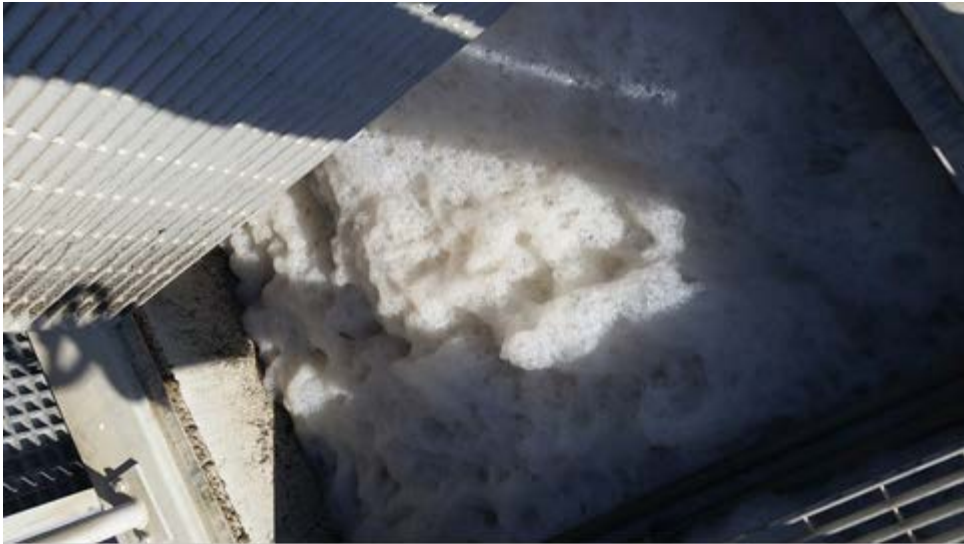
Figure 7: White foam in a Lancaster WRP grit chamber on 11-18-15 at 0815 hours.
