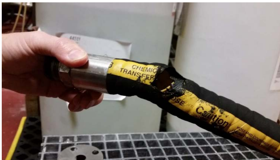
Figure 2: Ruptured acidic sanitizer solution flexible hose line at General Mills on 2-15-15.
