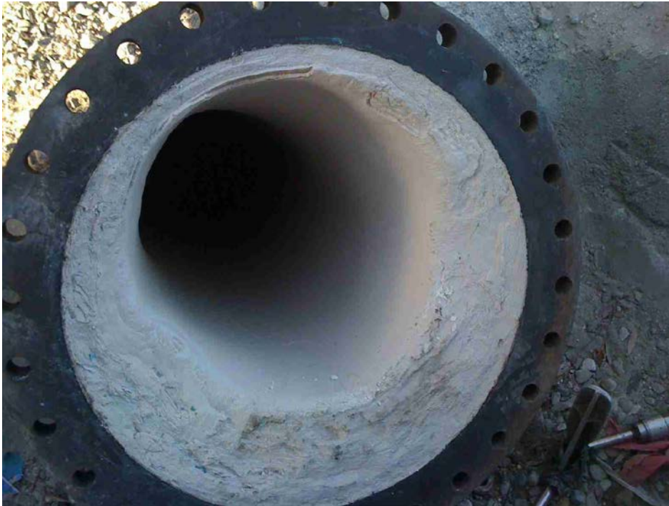
Figure 1: Example of the scale that typically builds up in the Tesoro refinery's 30" diameter I.W. discharge line. This photo was taken of the line in 2009.
