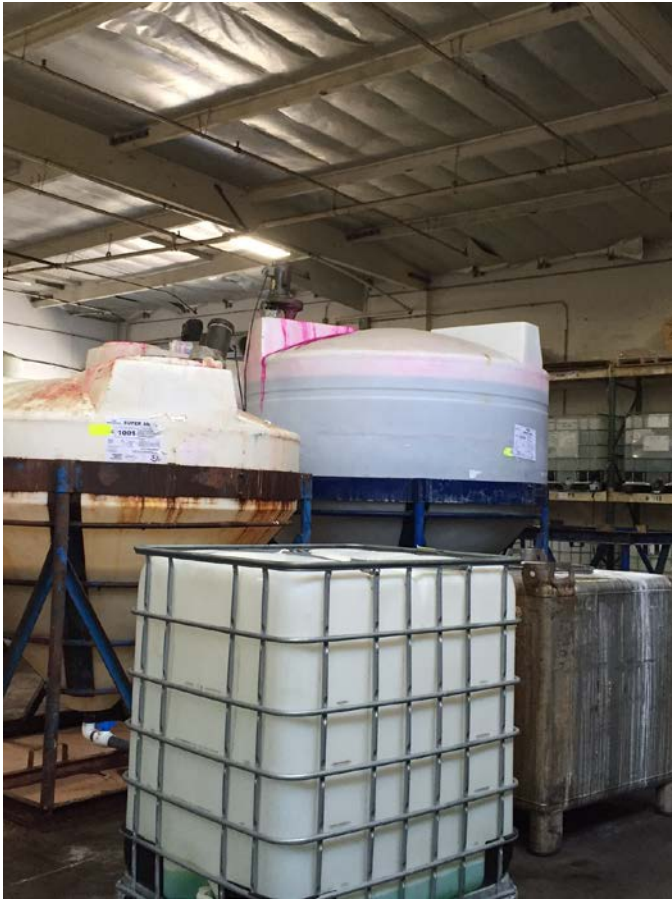
Figure 10: Approximate 1500-gallon cone-bottomed poly tank in the back of the photo nearly full of pink colored solution. Note staining present on the top of the tank.
