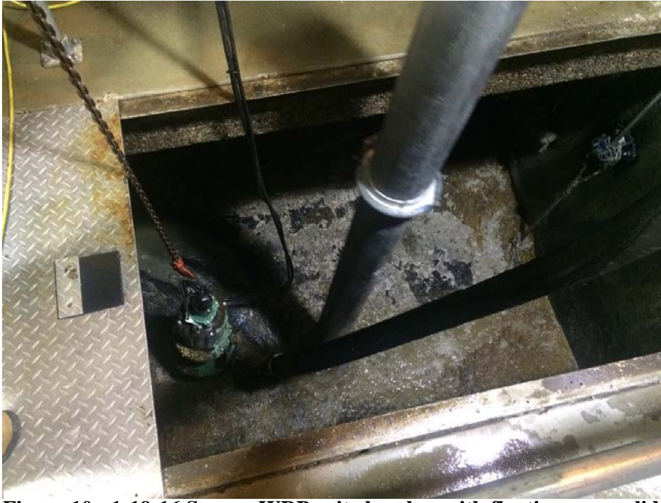
Figure 10: 1-19-16 Saugus WRP grit chamber with floating grey solids.
