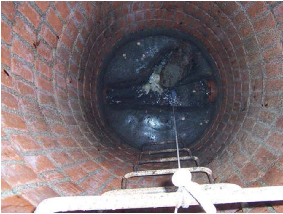
Figure 6: Gas trap valve on the SGVFO sewer line (entering from the 1:00 o'clock position) found wired open on 3-17-16.
