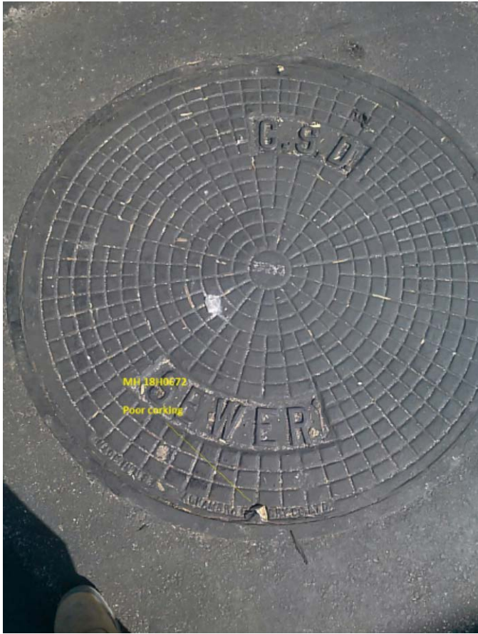
Figure 3: MH 18H0672 on 9-1-16, note partially displaced and torn cork in one of the pick holes.
