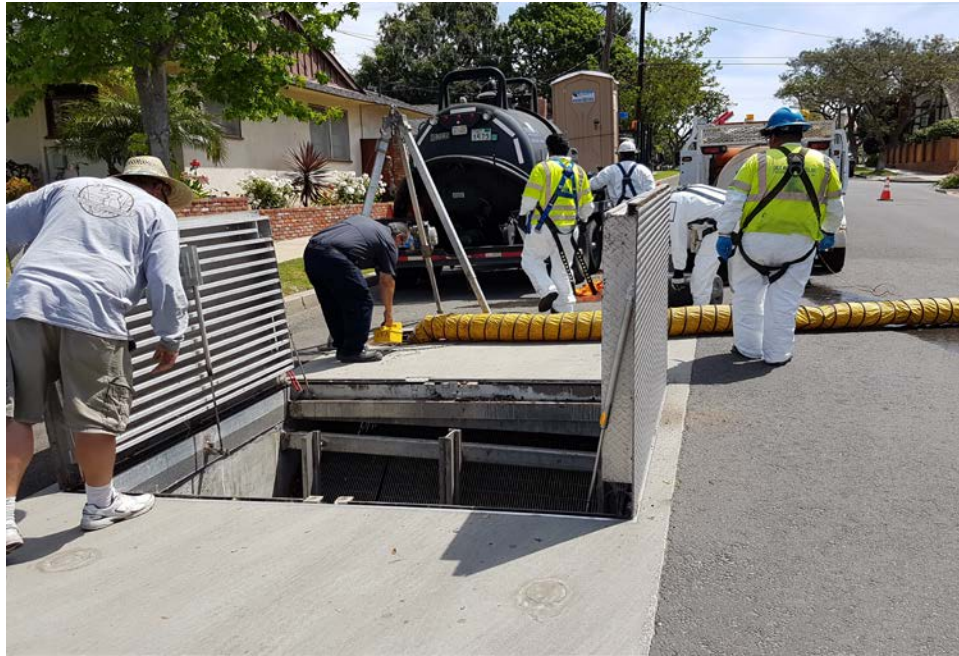
Figure 10: April 22, 2016 at 1129 hours. Ocean Blue Environmental Services contract crew cleaning up stormwater vault located just upstream of the Colorado Lagoon in Long Beach.
