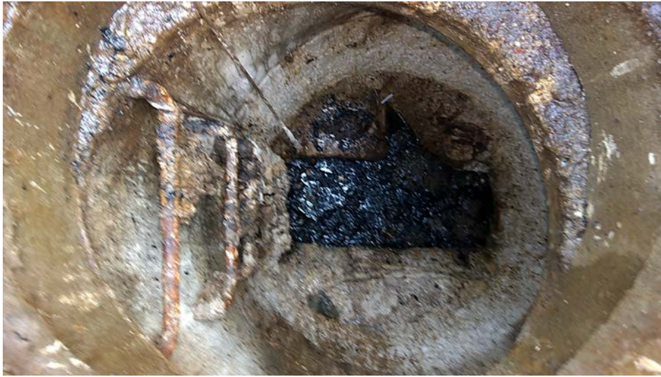
Figure 1: 1-6-16 Florence Avenue Trunk MH 1081 photo of the 2" thick layer of black oily material in the sewer channel.
