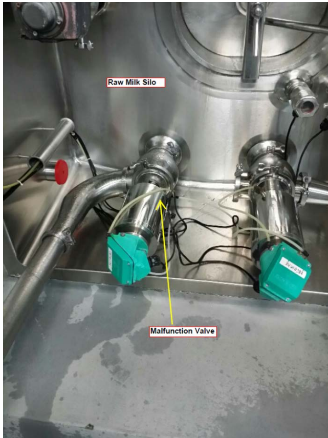
Figure 2: Base of the 50,000-gallon stainless steel raw milk silo and the tank's pneumatically controlled bottom inlet valve that failed, causing about 17,000 gallons of its contents to drain into nearby floor drains that flowed directly to the sewer.
