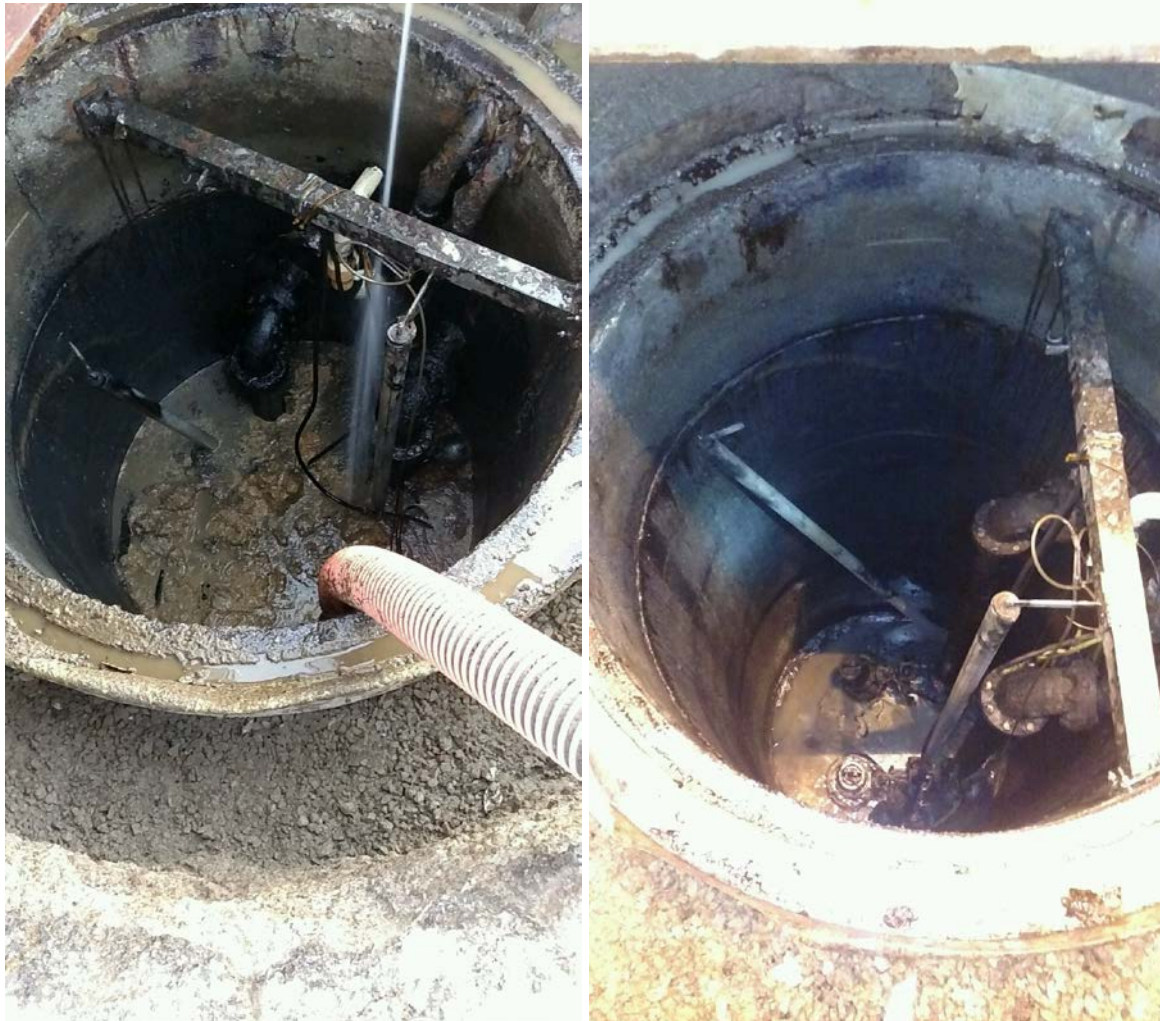
Figures 8 and 9: These photos were supplied by Ocean Blue Environmental to area I.W. Inspector Sanjay Patel to document the heavy solids they encountered when servicing the small sewage pumping station wet well at the Hanjin Terminal in Long Beach on 1-15-16.
