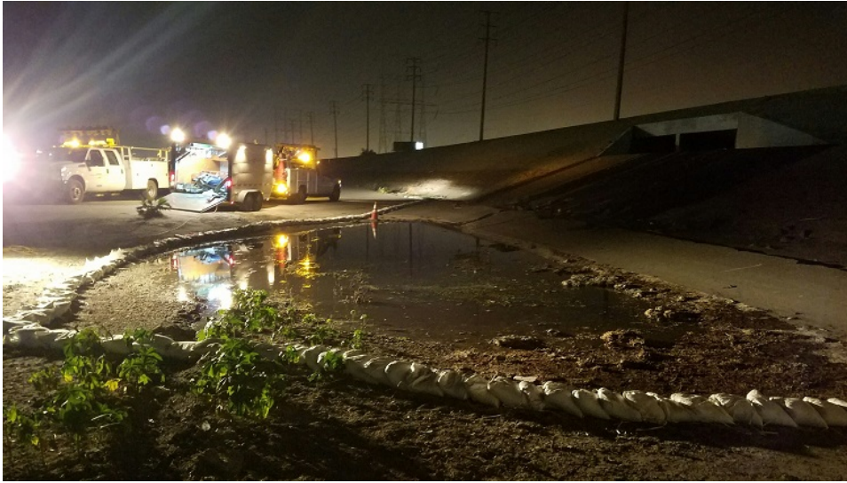
Figure 5: Districts' crew from the Compton Maintenance Yard on-site in the Los Angeles River Channel at about 2200 hours on 8-17-16 performing containment of the wastewater that entered the river.
