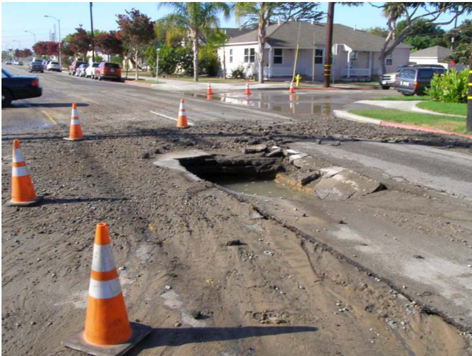
Figure 9: 9-11-16, 0830 hours sinkhole on Crenshaw Blvd.
