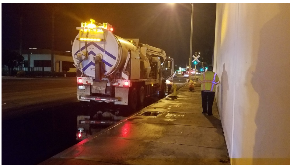
Figure 11: 10-28-16 1930 hours Vactor truck operations on Eastern Avenue removing firewater from the stormdrain system.
