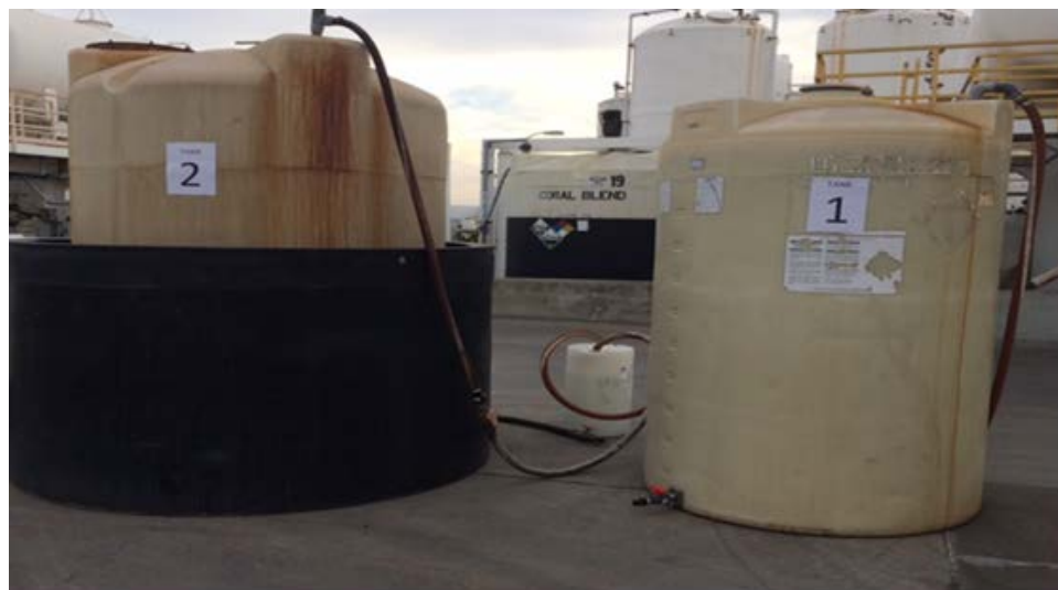
Figure 1: 11-22-16 photo from Eugene Boudreau showing the two tanks containing the spilled acid and spill containment area wash down water.
