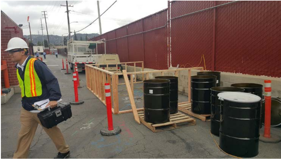
Figure 1: IW Inspector Nguyen Dang at the Quemetco sewer excavation site on 5-5-16 prior to excavation commencing.
