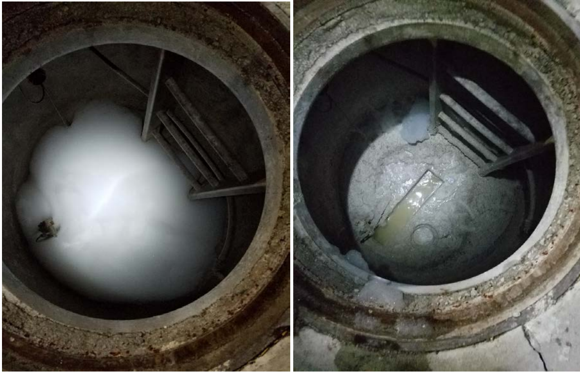
Figures 3 & 4: G & K Services legal sample point. Left photo shows \approx 2' of foam in the sample point vault at 8:15 p.m. on April 8, 2016. Right photo taken 20 minutes later shows the vault after defoamant was added.
