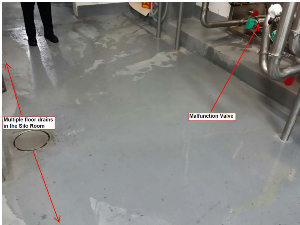
Figure 3: 7-12-16 photo showing the close proximity of the valve that failed to the nearest sewer floor drain.
