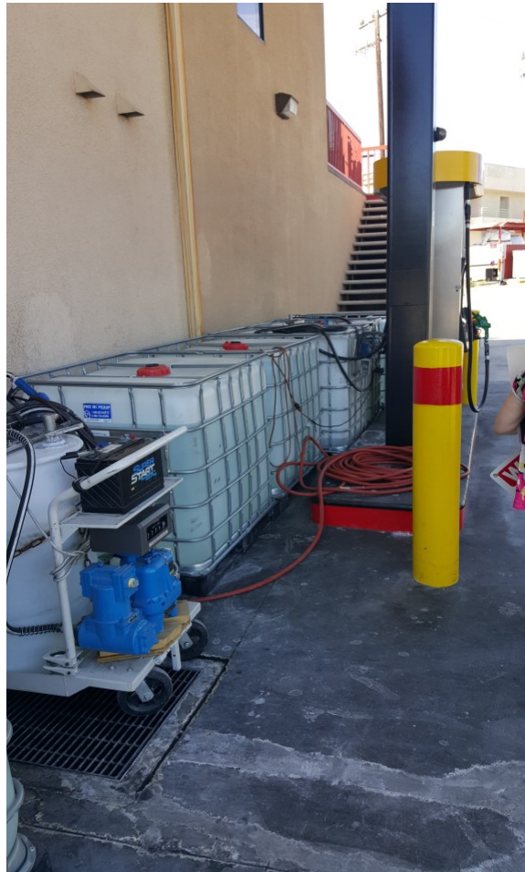
Figure 7: DEF storage tanks at the Castaic Truck Stop.
