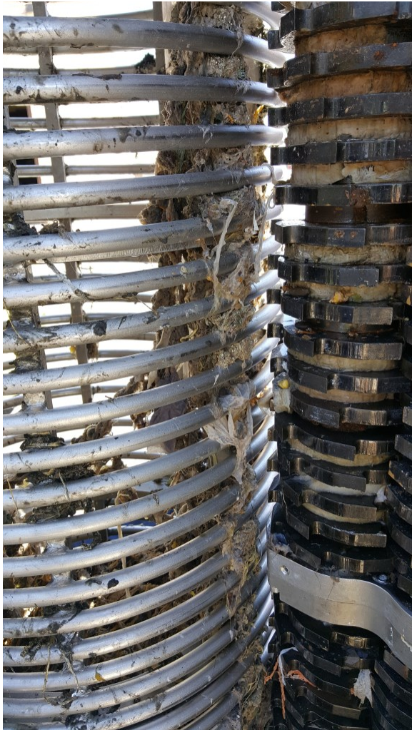
Figure 2: 8-1-16 photo of Saugus WRP Channel Monster with remnants of the “rubber band like” materials present.
