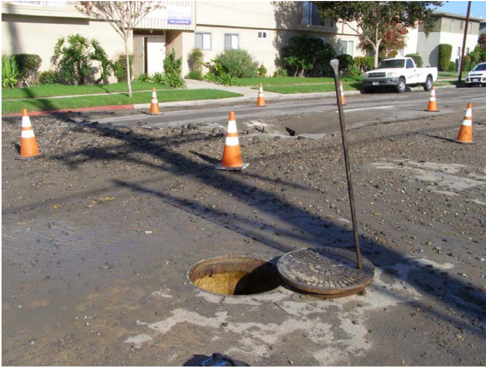
Figure 8: 9-11-16, 0830 hours MH 05 0064 on the 36" District #5 Main Trunk. Note sinkhole in the background.
