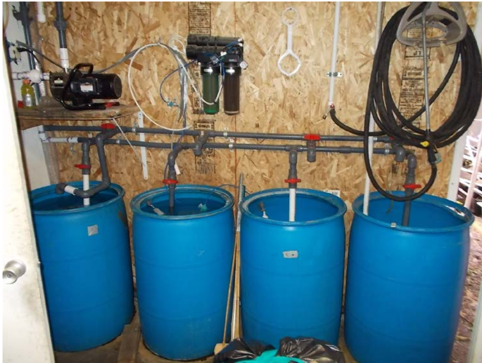
Figure 5: Jury-rigged water distribution system showing water barrels, pumps, and filters used to distribute water and fertilizer to the plants.
