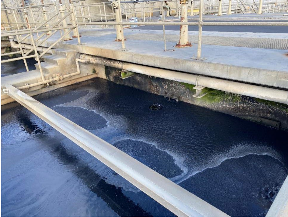
Figure 1: Unusual clarifier skimmings at JWPCP secondary tanks on October 20, at 0800 hours that appear to contain a petroleum sheen.
