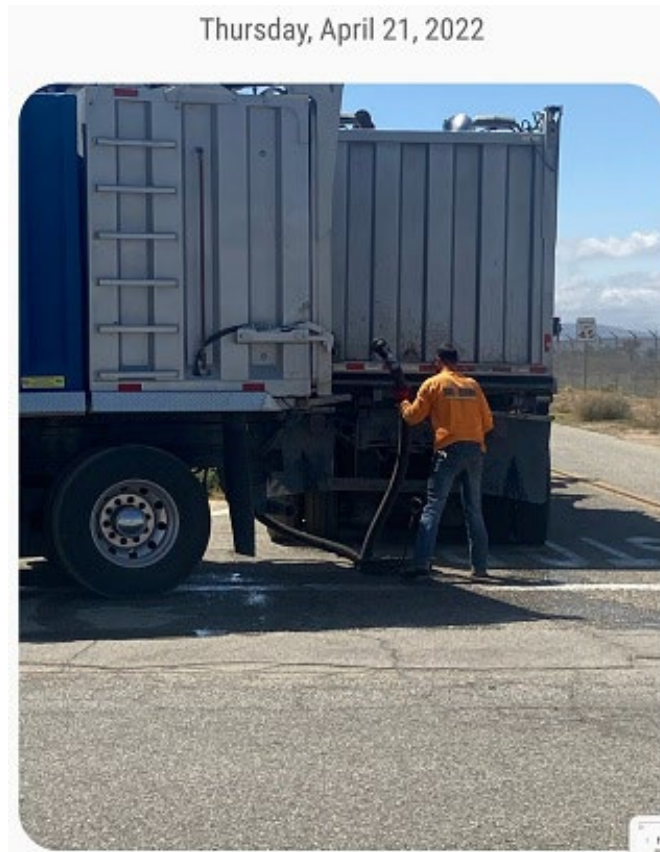
Figure 7: Photo provided by Palmdale Code Enforcement of a Cal Stripe Inc. worker discharging wastewater directly into MH 20 0100 at about 1500 hours on Thursday, 4-21-22.
