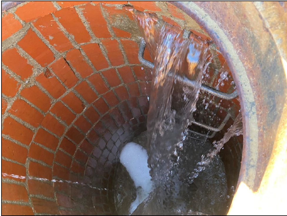
Figure 1: Photo taken on December 20, 2022, at 0900 hours showing the active infiltration of the firewater from the ruptured underground firewater line into a sewer system manhole on the Plant 42 property.
