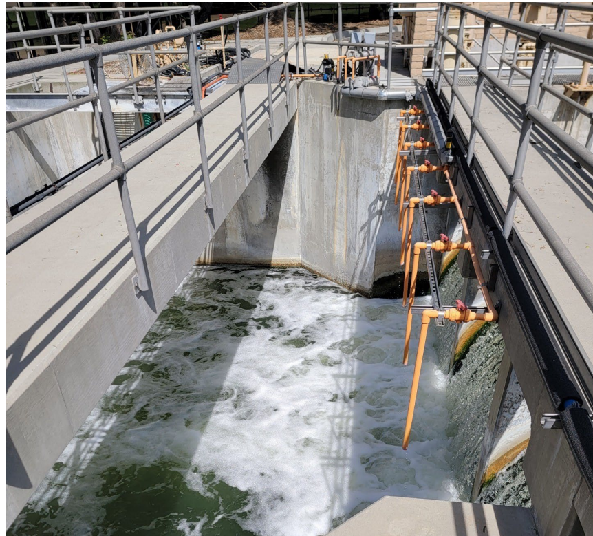
Figure 5: LCWRP Final effluent forebay at 1230 hours on 3-17-22. Note the floating white foam.
