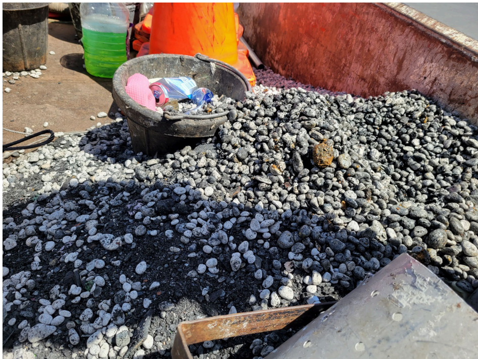
Figure 1: Pumice stone removed by Districts' sewer maintenance crews from two siphon structures in Carson on the Main Street relief trunk sewer on May 9, 2022.
