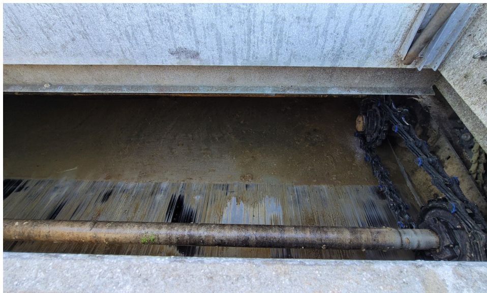
Figure 4: WNWRP primary tank skimmer. Note the brown oily material which was sampled and tested with FTIR scan analysis.
