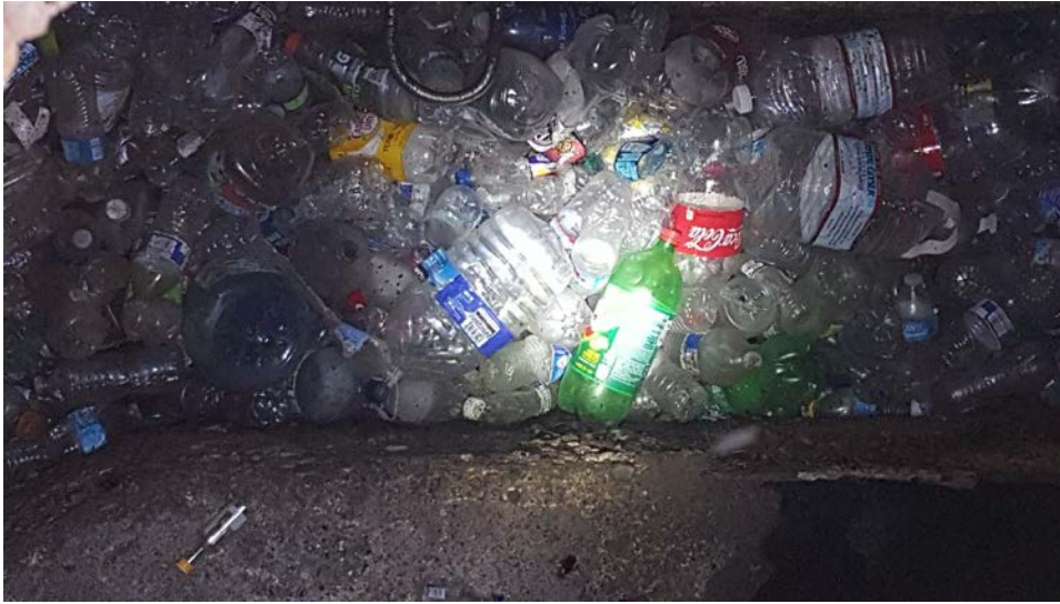
Figure 3: Plastic bottles in the Montebello Relief trunk sewer at MH 02 1530 on 9-12-17.
