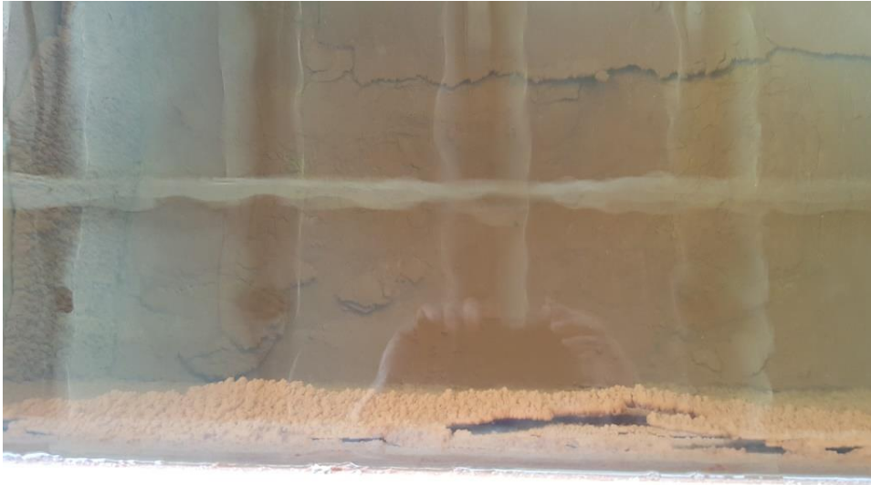
Figure 2: Calcium scale in the weir box at Davis Wire Corp. on 4-7-17. This is the same type of scale noted at MH 22 1214A.
