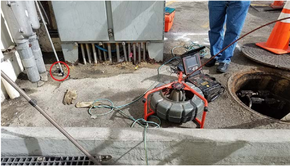
Figure 8: Rupture area. Note the approximately 5" hole in the pavement inside the red circle where the spilled wastewater came up and overflowed.
