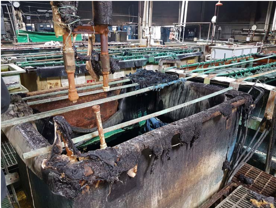
Figure 5: Aftermath of the 6-8-17 fire at Cal-Tron Plating in Santa Fe Springs. Note that the tanks containing the concentrated plating solutions remained essentially intact.
