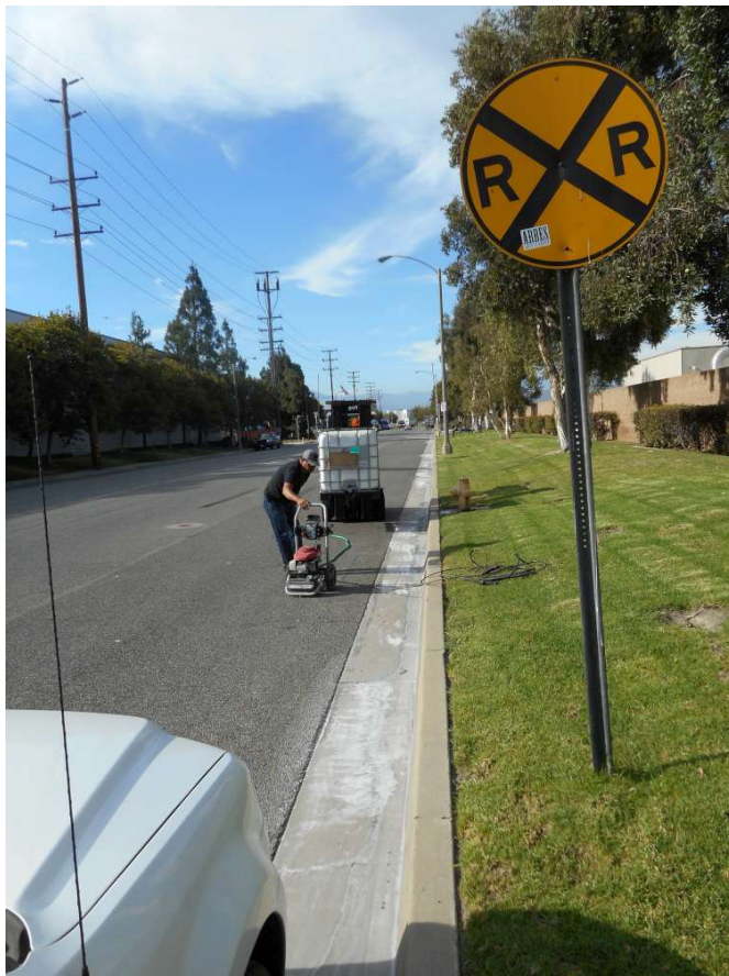
Figure 5: Contractor preparing to pressure wash the street gutter to remove residual salts on 7-27-17 at 1605 hours.
