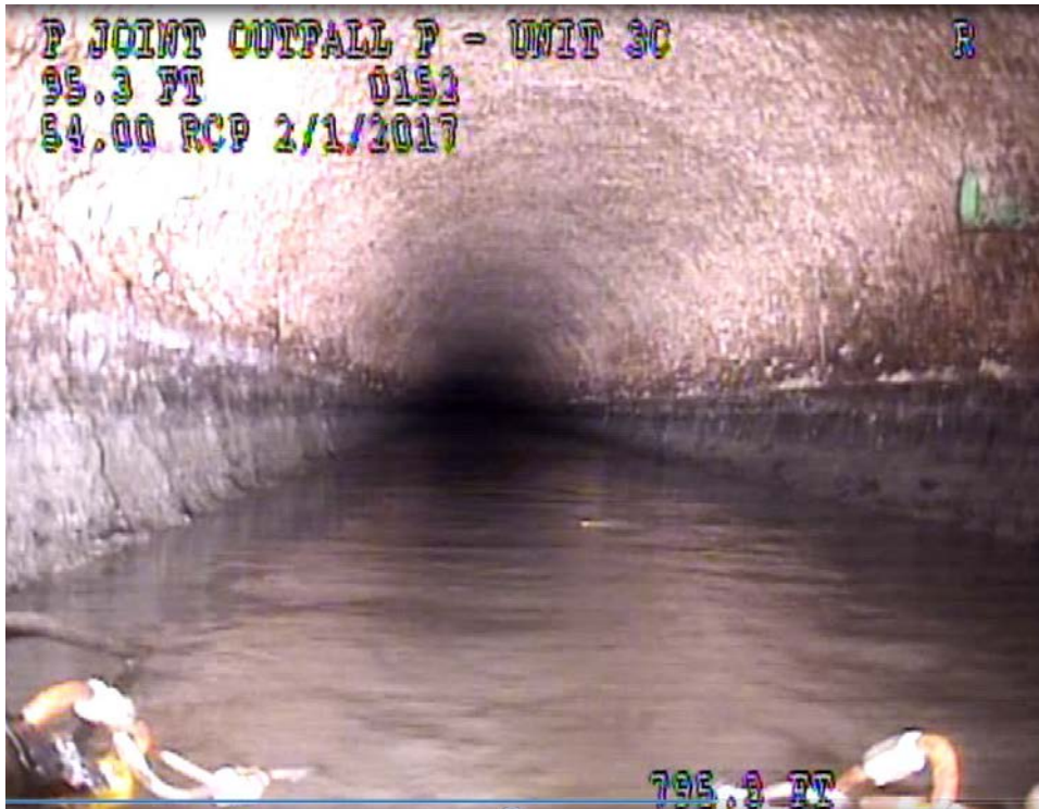
Figure 1: 2-1-17 CCTV photo grab of the illicit connection into the J.O. 'F' Unit 3C Trunk in Cerritos approximately 500' north of MH F 0152. The illicit connection pipe is located in the upper right of the photo.
