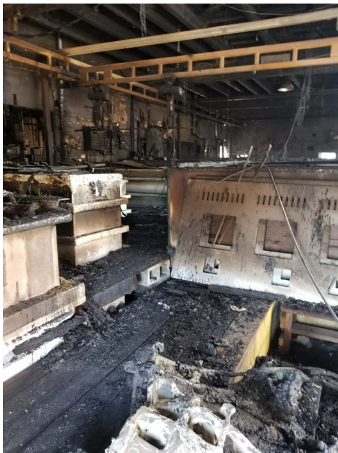
Figure 1: Interior of the processing building of Gardena Specialized Processing post fire on 8-14-17.
