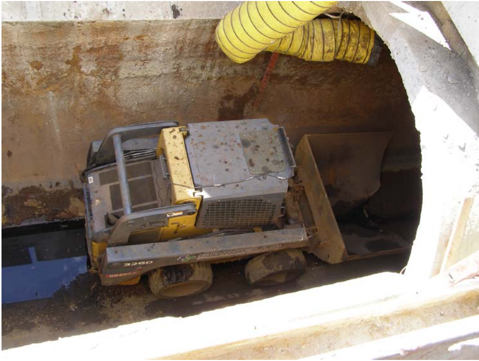
Figure 7: Bobcat excavator in the 144" J.O. 'B' Unit 1A trunk sewer at the rehabilitation project access point in between MHs B14 and B15.
