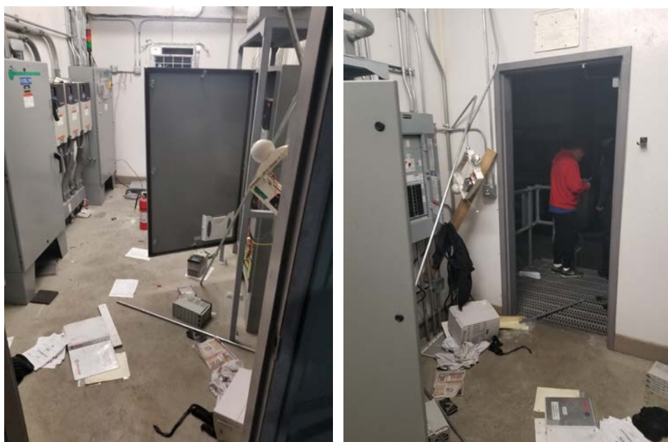
Figures 6 and 7: Photos showing the damage inside the White Wave Foods wastewater pretreatment system control room.
