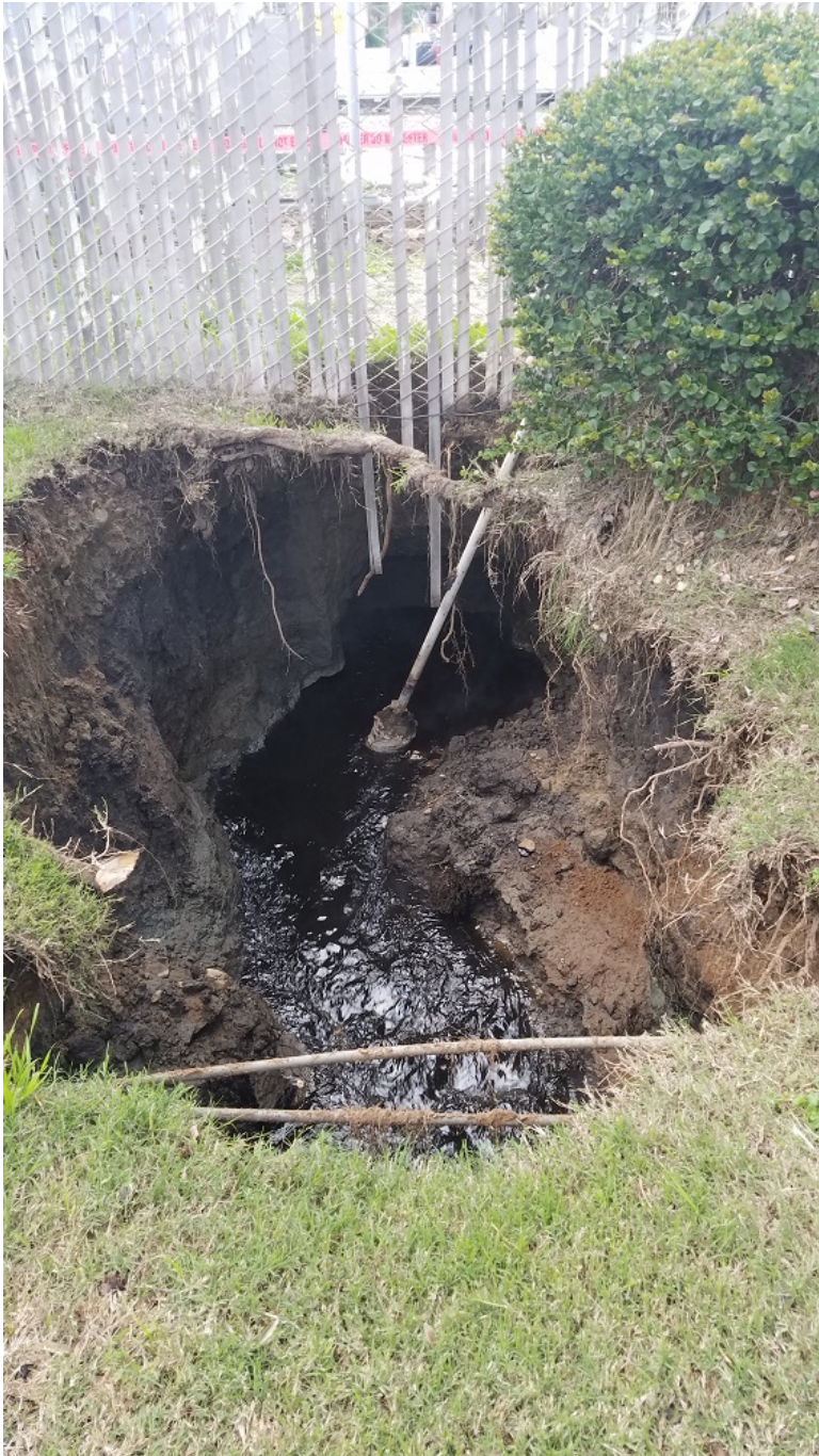
Figure 5: View of the sink hole at the Torrance Refining Company on 1-24-17.
