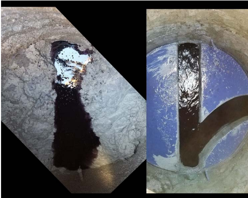
Figure 2: Comparison of the lateral line at the manhole cover 2 location. Left side is before cleaning and the right side is after cleaning and pumping.
