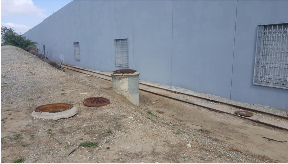
Figure 11: MH A 1047 riser (on the right) and the associated siphon structure airline manhole (on the left).
