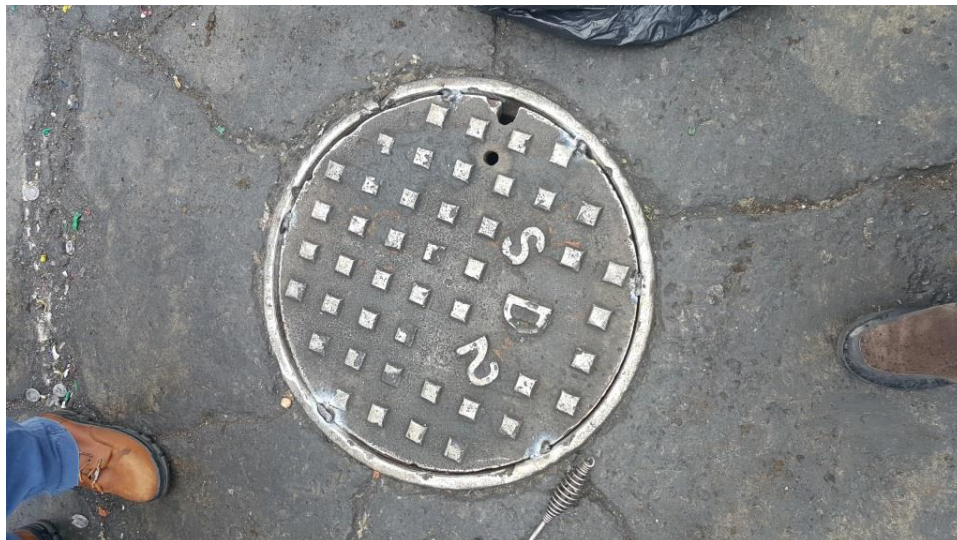
Figure 8: 9-21-17 photo of MH 02 0994 tack welded closed.
