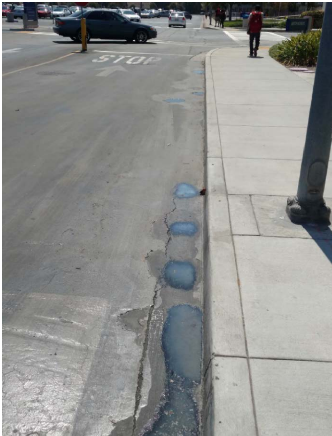
Figure 1: Small puddles of milky-white colored liquid noticed at 1235 hours on 9-6-17 by IW Inspector McCurdy at Cerritos College.
