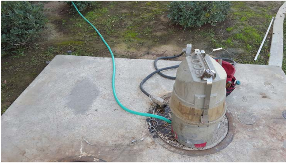
Figure 4: Potable water hose stuck through the sample box cover at La Amapola Inc. in Santa Fe Springs at 1000 hours on 10-26-17. Note the Districts' 24-hour composite sampler. Also note the effluent pH probe conduit and housing immediately adjacent to the hose.
