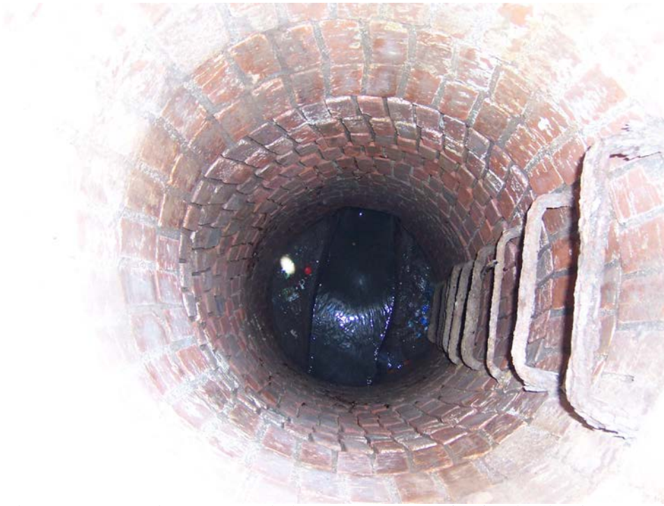
Figure 6: Plastic bottles sitting on the shelf of Districts' sewer MH 02 0994.
