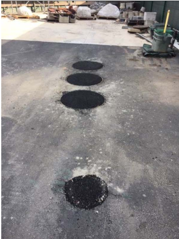
Figure 5: 4-25-17 photo of the sealed and abandoned washpad drain and clarifier.
