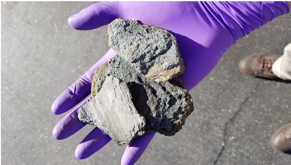
Figure 3: Pieces of stone debris found in the lateral line at the discharge location of A's Match Dyeing Company.
