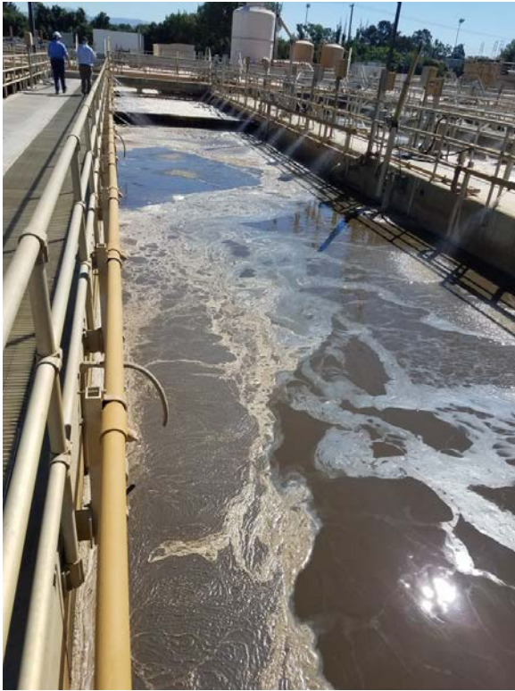
Figure 10: 6-15-17 Valencia WRP secondary treatment tank with floating material.
