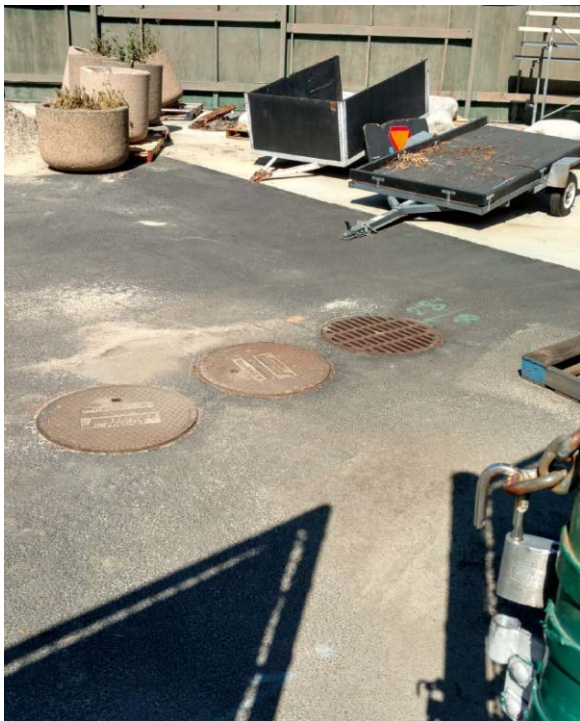
Figure 4: Drain and 2-stage clarifier next to the Cerritos College Baseball field that was illicitly connected to the J.O. 'F' Unit 3C Trunk in Cerritos.
