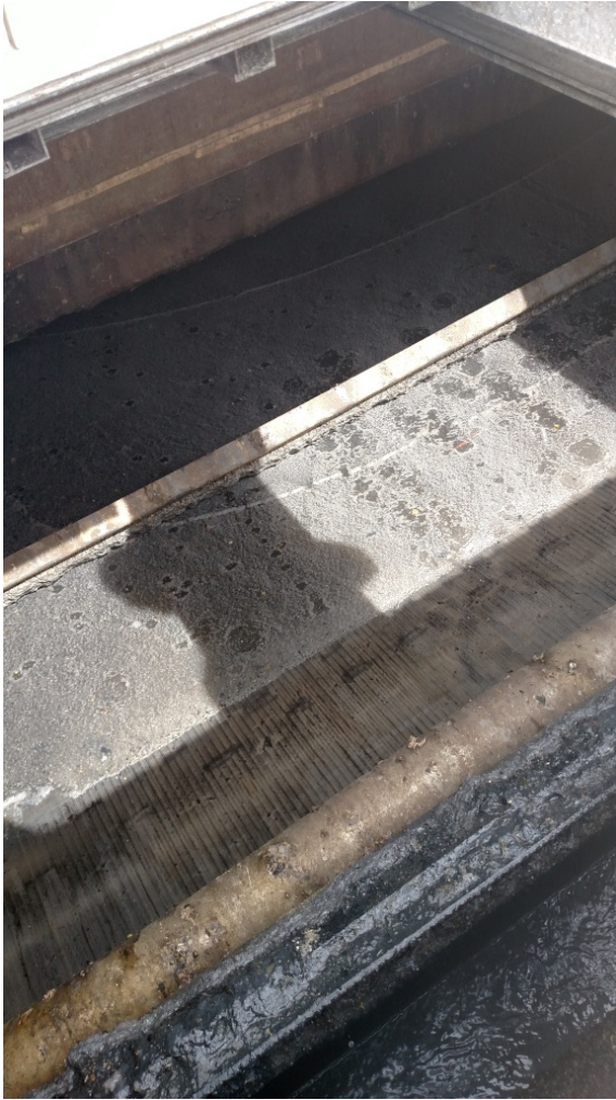
Figure 7: Unusual bubbles/foam on the primary tanks at Valencia WRP on 3-22 17.
