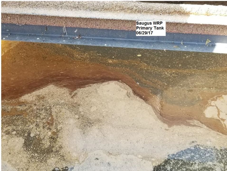
Figure 12: Oily material in a Saugus primary tank on 6-29-17.
