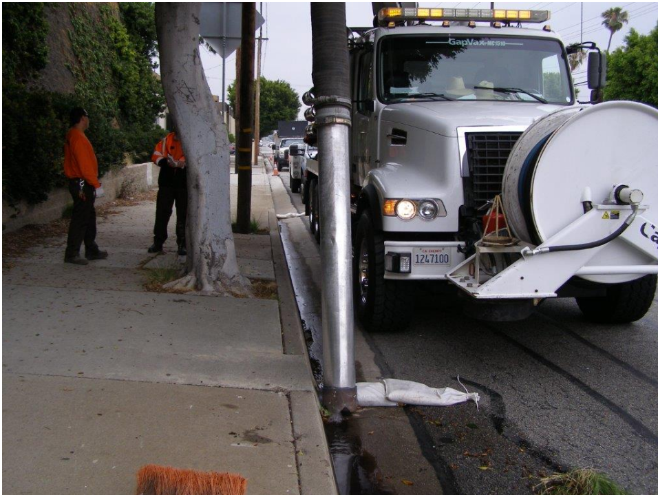
Figure 7: City of Hawthorne maintenance crew Jet Vac truck and sand bag containment.
