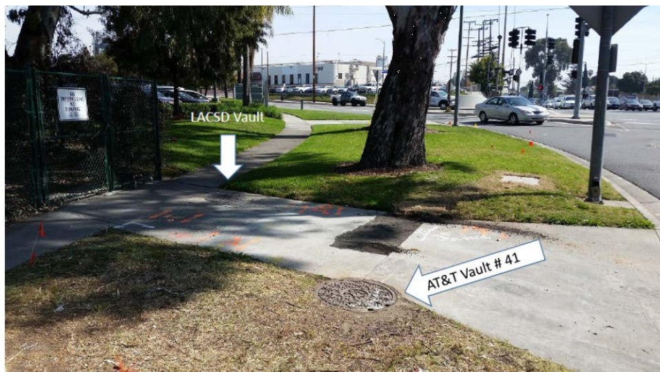
Figure 2: AT&T photo showing the AT&T vault that was reported to contain sewage, and the adjacent "LACSD Vault" (actually Manhole 05 0018 on the 48" District 5 Main Trunk).
