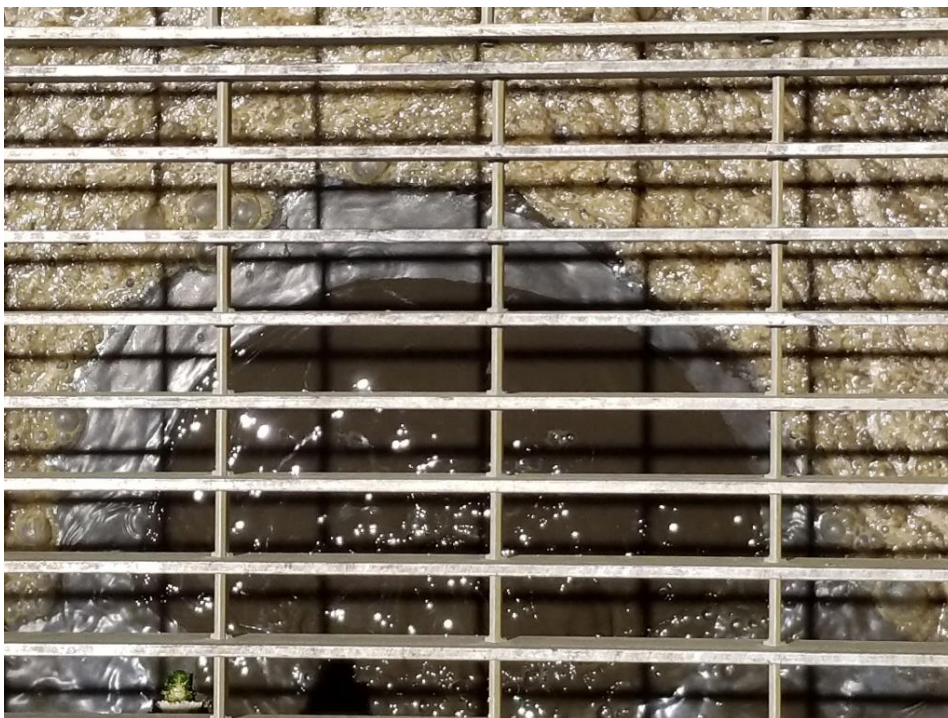
Figure 6: 6-15-17 Valencia WRP secondary treatment tank bubbles showing the slight sheen reported both on 6-15-17 and again on 7-28-17.
