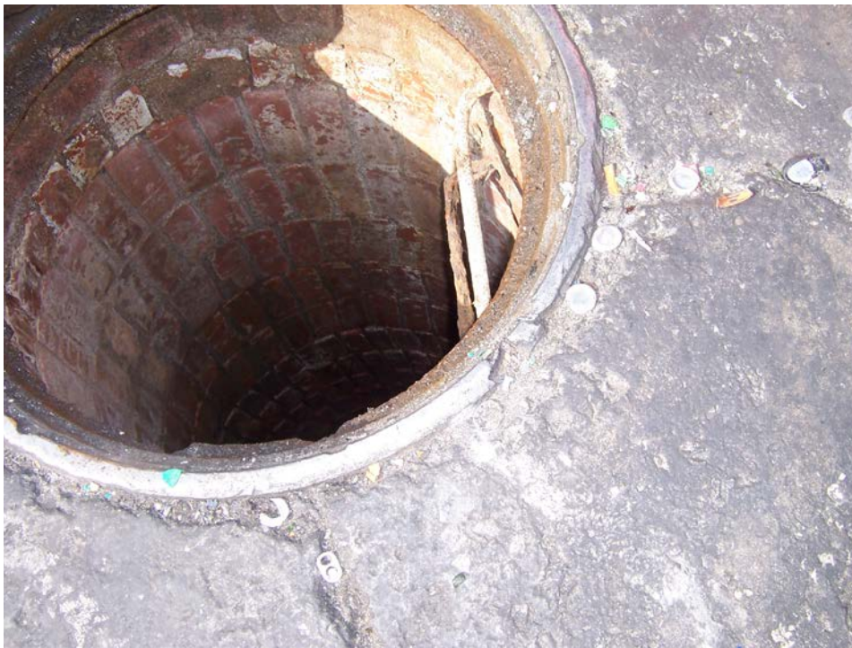
Figure 7: Damaged frame of MH 02 0994 indicating it is subjected to frequent "heavy hits." Note that the manhole cover is a non-locking type.
