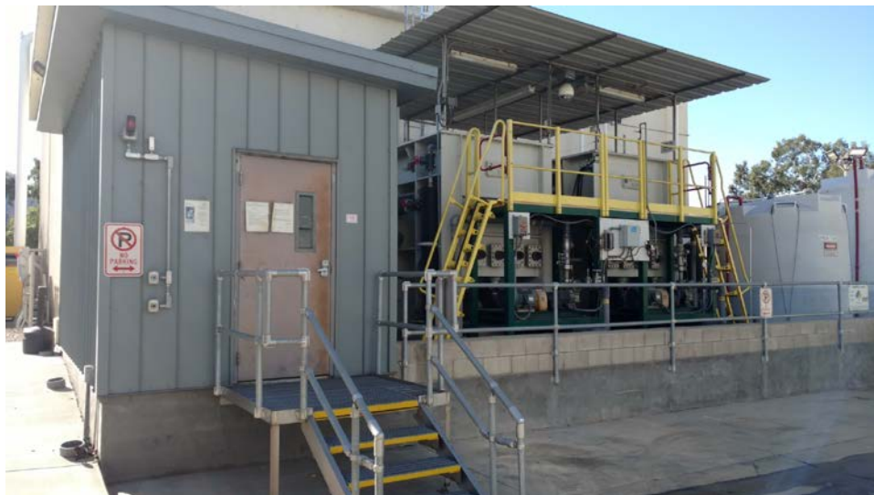
Figure 5: The pretreatment system (on the right) and its control room (grey building on the left) at White Wave Foods.
