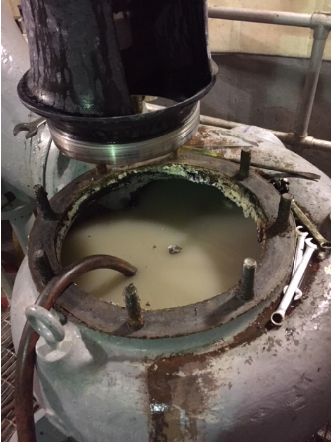
Figure 5: 12-17-17 photo of the Coyote Creek pumping plant pump taken by PP maintenance staff. Operators stated the grease shown inside the pump housing/chest was at least several inches thick.
