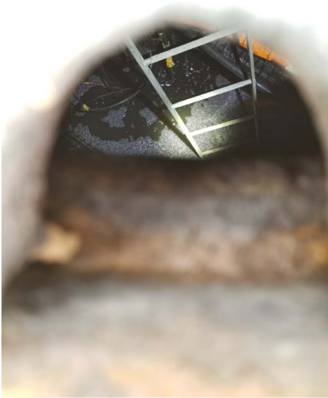
Figure 3: 10-19-17 photo of the AT&T vault interior through the vault cover pick hole. It was noted the water visible inside was not flowing, but that there were bubbles present, likely coming from the AT&T lines, through which air is fed to keep moisture out.
