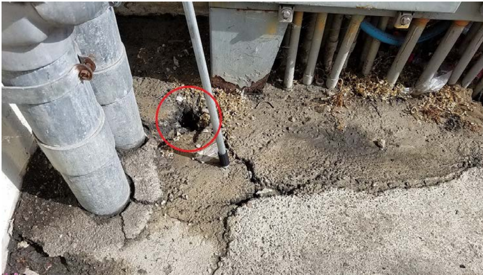
Figure 9: Close-up photo of the rupture hole.
