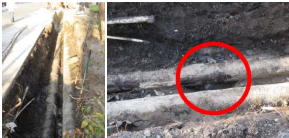
Figures 4 and 5: Excavated pipeline and small hole in the pipeline that was the source of the leak/spill.
