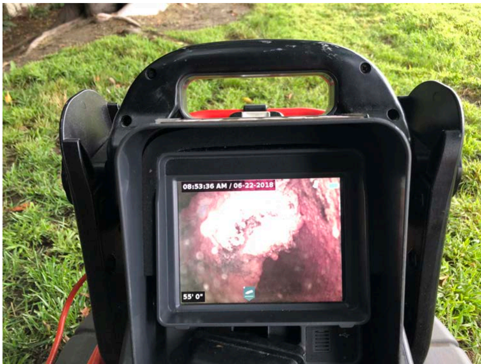
Figure 10: 6-22-18 contractor CCTV view of scale in the private line.
