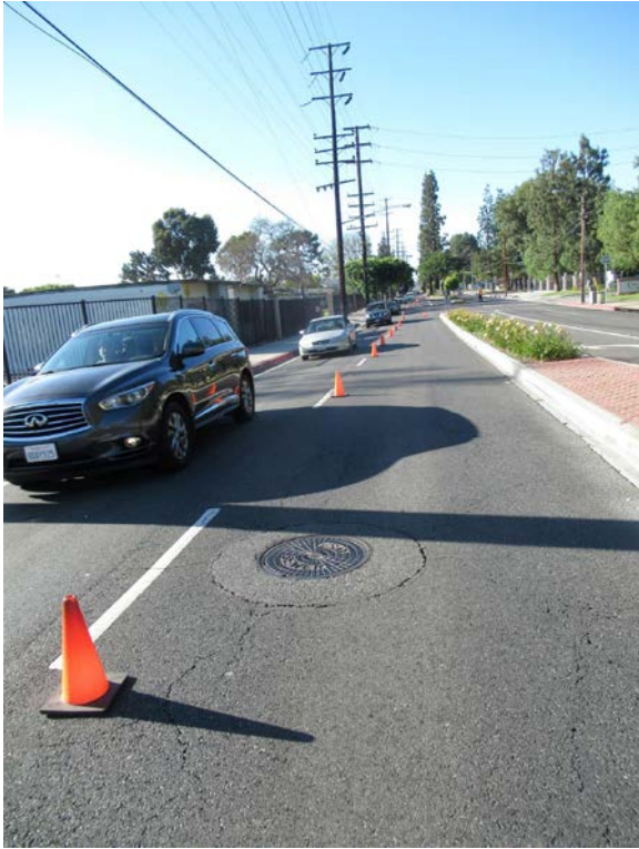
Figure 8: 6-13-18, 1756 hours MH 02 0390 on the 15" Downey Ave. Extension Trunk. Note traffic diversion set up by Woods and McIntosh to check the line.
