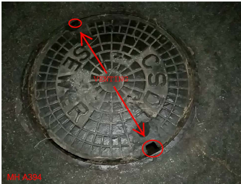
Figure 3: 12-14-18, 1720 hours photo of MH A394. Note the open pickhole notches that were found to be venting sewer headspace gas.
