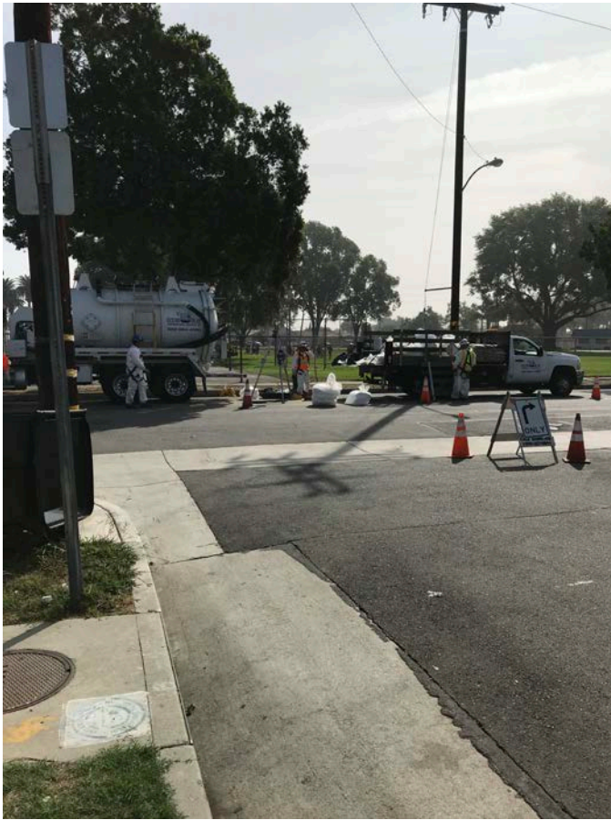
Figure 3: 10-29-18 photo of contractor Ocean Blue Environmental Services conducting clean-up in the street and storm drains impacted by the spill.
