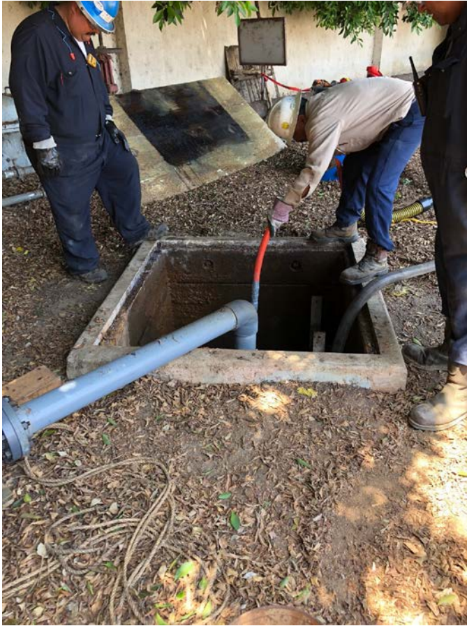
Figure 2: Contractor jetting the line scale at the AltAir Paramount facility's private lateral line on 7-17-18.
