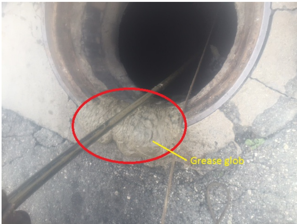
Figure 1: Glob of grey grease removed from the 21" J.O. 'H' unit 2F trunk sewer in Vernon on 4-2-18.
