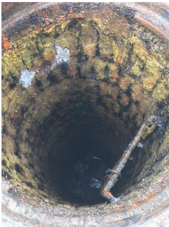
Figure 5: MH 08 0150 riser on 3-14-18. Note the layer of biological slime growth.
