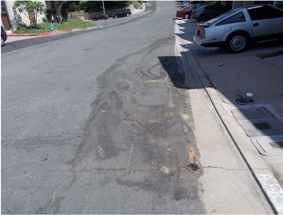
Figure 2: Photo taken on 6-26-18 by Finn of the street cracks with whitish/yellowish powder residue in the asphalt where he noted the odorous (sulfide) gas was emanating. Note the staining indicating that either some liquid is also coming out or that someone is periodically washing down the area.
