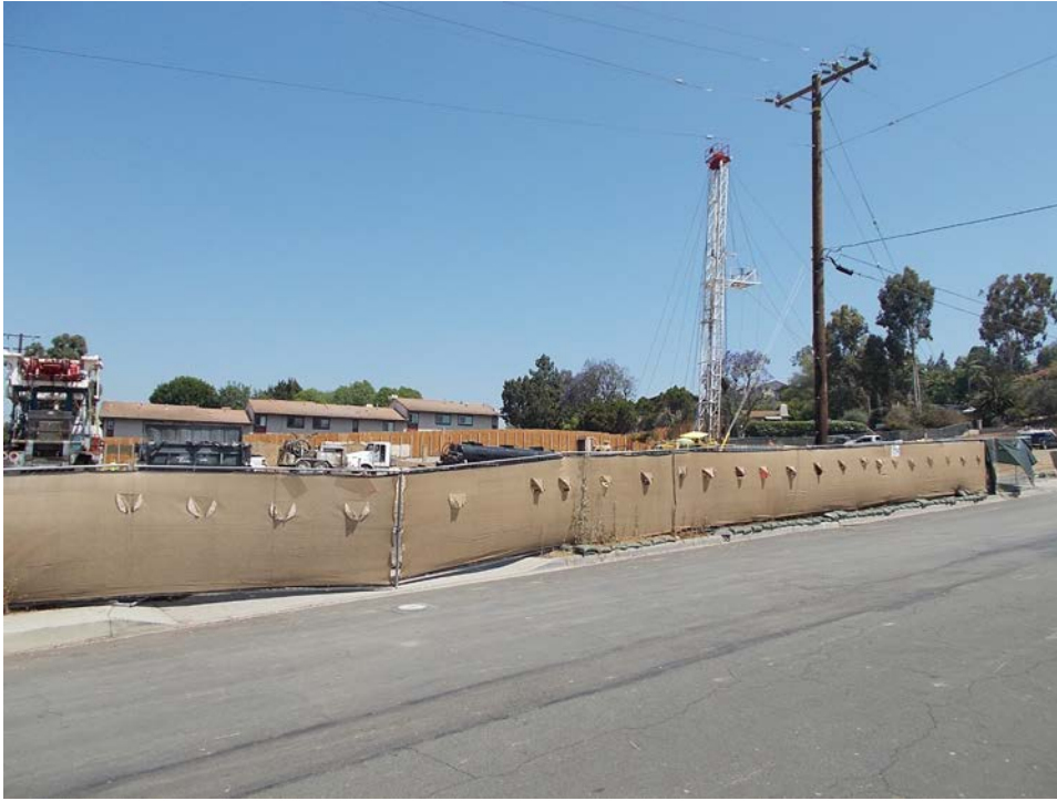
Figure 2: Photo of the oil well abandonment construction site looking north from Davidson Drive. The home where the sewer/sulfide odor was reported is located beyond the far fence line visible in the photo.
