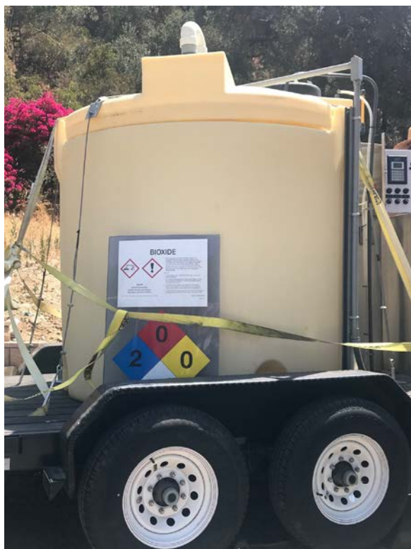
Figure 7: 8-24-18 photo of the 750-gallon poly tank of "Bioxide" solution at the Meritage Homes' development sewer lift station.
