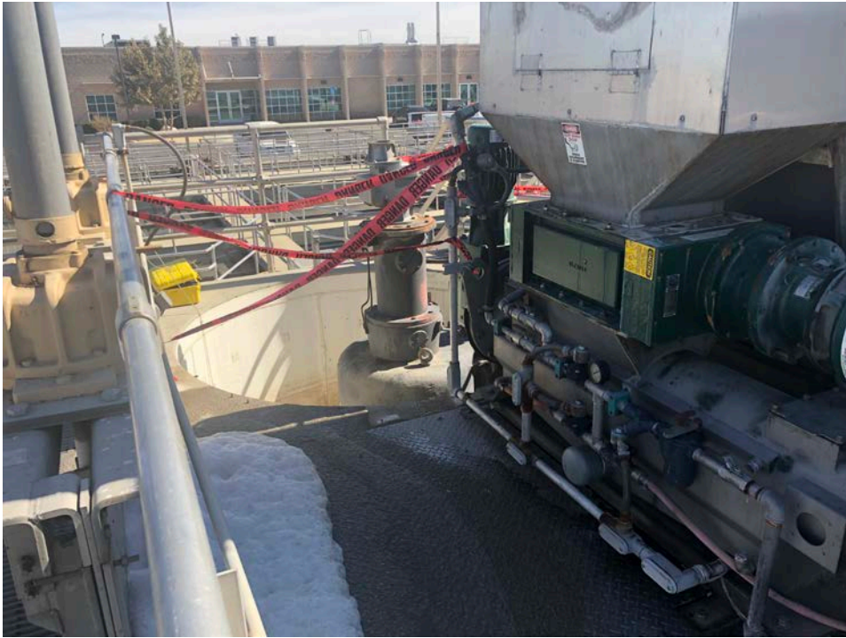
Figure 4: 10-29-18 photo of the foam at the Palmdale WRP headworks.
