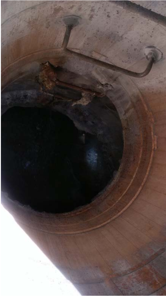
Figure 13: 3-30-18, 1330 hour photo of the MH A1087 riser. Note that at that time only a small residual of the white foam remained on the manhole shelves. In order to escape through the pick holes it must have completely filled the riser earlier.
