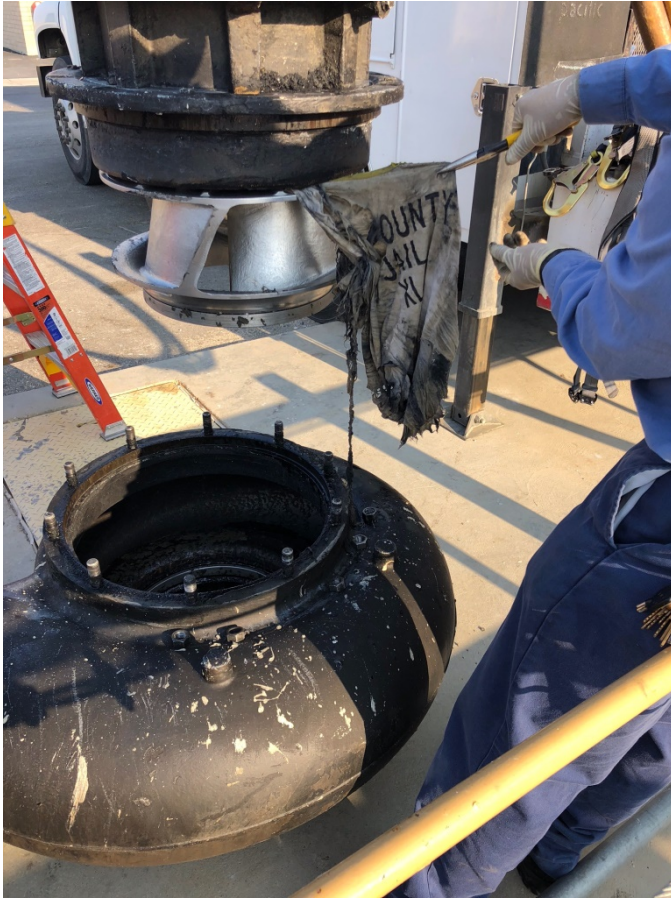
Figure 4: 7-21-18 photo of the rag removed from the influent pump.
